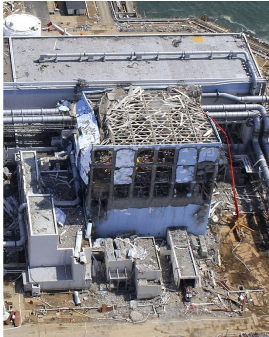
March 24, 2011. The Air Photo Service UAV image shows the damaged Unit 4 of the crippled Fukushima Dai-ichi nuclear plant.
