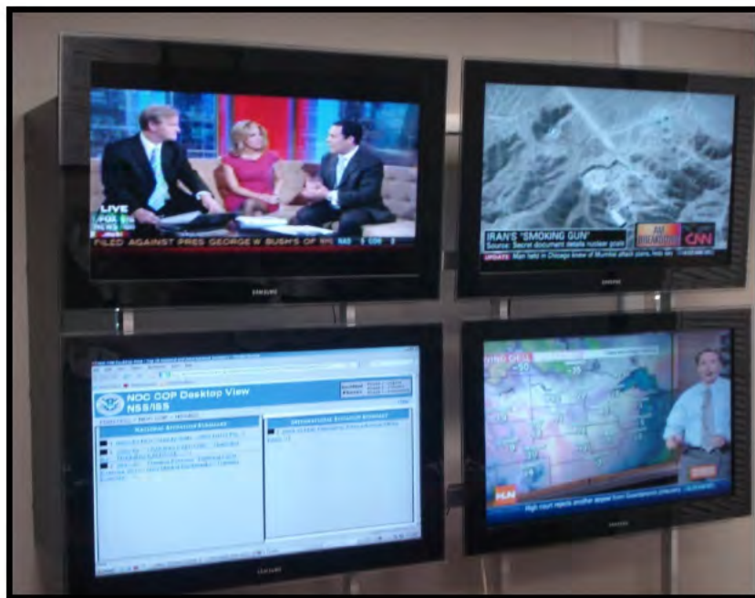
MMC Front of Room Monitors
