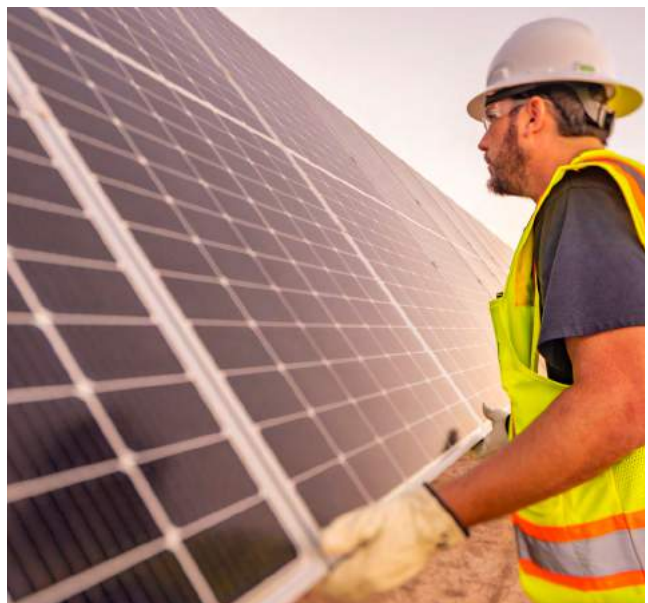
Image courtesy of Enel Green Power
