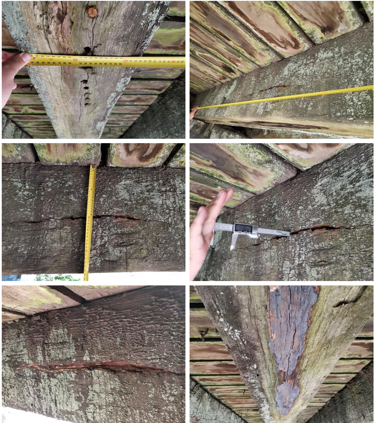
Figure 4 Timber Stringer No. 4 Defects
