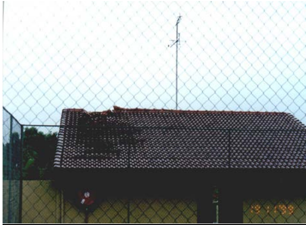
Figure 2.3: Structural damage to a club house due to direct lightning strike (McKechnie and Jandrell, 2008).
