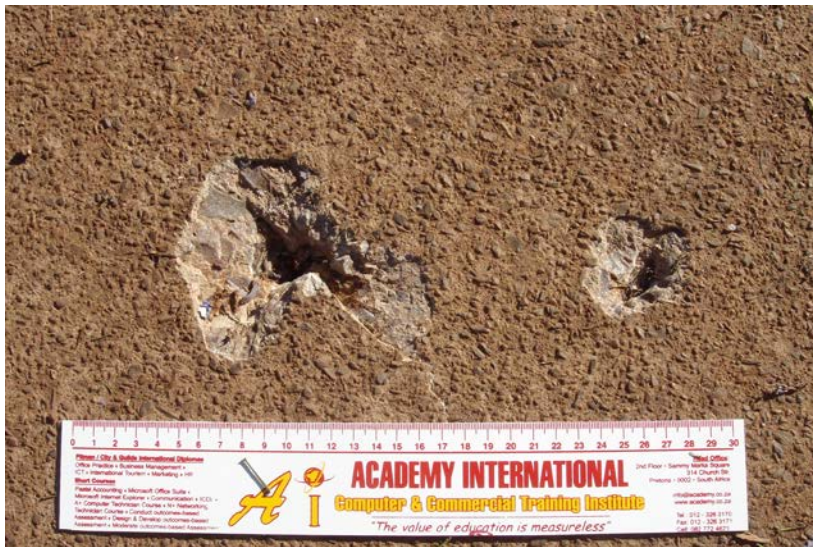
Figure 3.3: Blast / explosion effects from the lightning noted on the concrete pavement on the right side of the victim.
