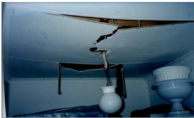
Figure 2.4: Signs of a roof having collapsed. Structural damage caused to a club house building as a result of direct lightning strike (McKechnie and Jandrell, 2008).
