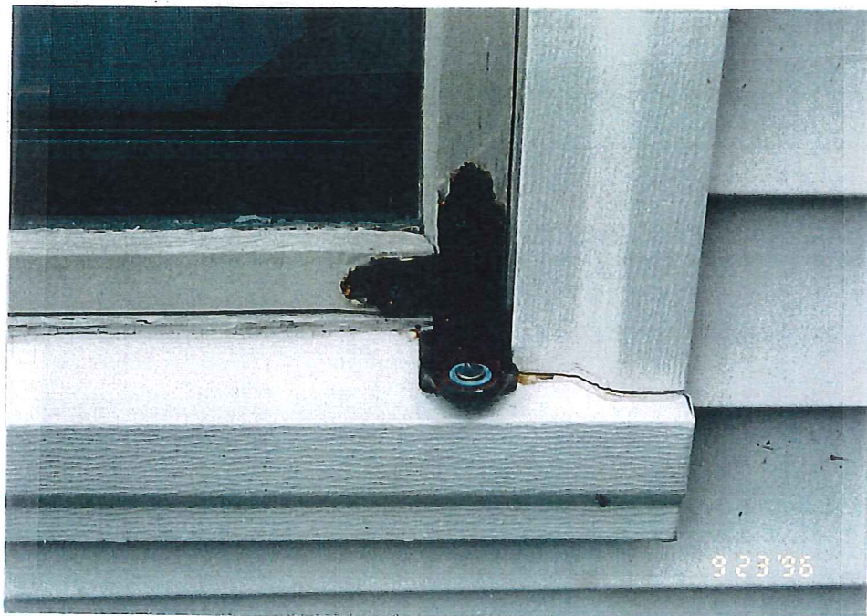
RUSTY WINDOW HARDWARE.
