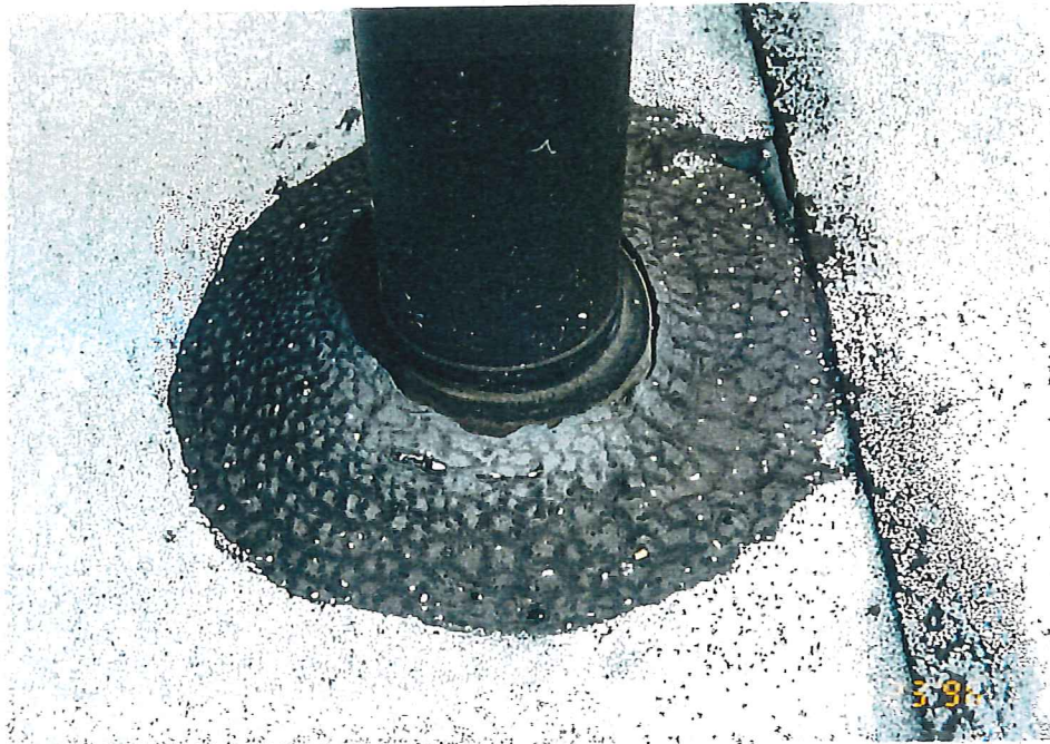
CRACKS IN ROOF PENETRATION FLASHING.
