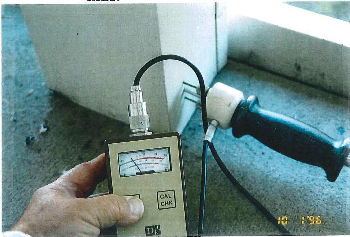
MOISTURE CONTENT IS 12% AT WALKWAY POST BASE.
