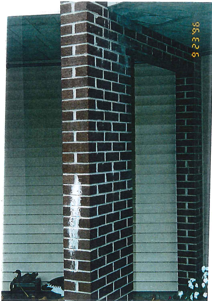
EFFLORESCENCE IN PIER.
