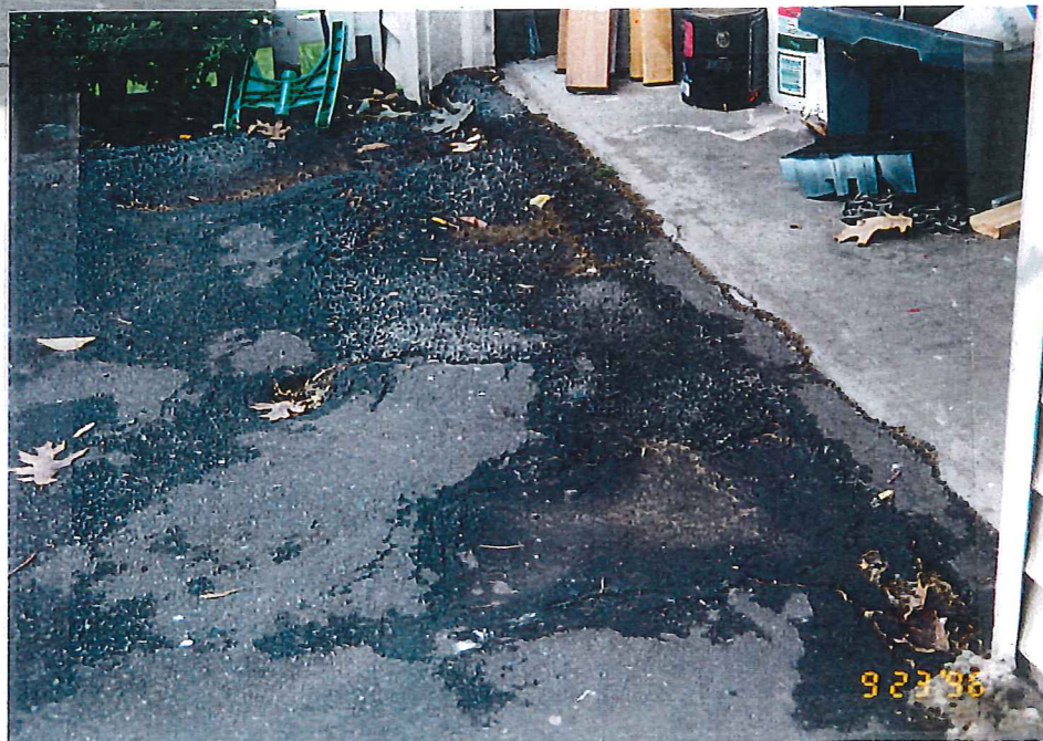
CRACKED PAVING, SUBSIDING SOIL AT MAINTENANCE GARAGE.
