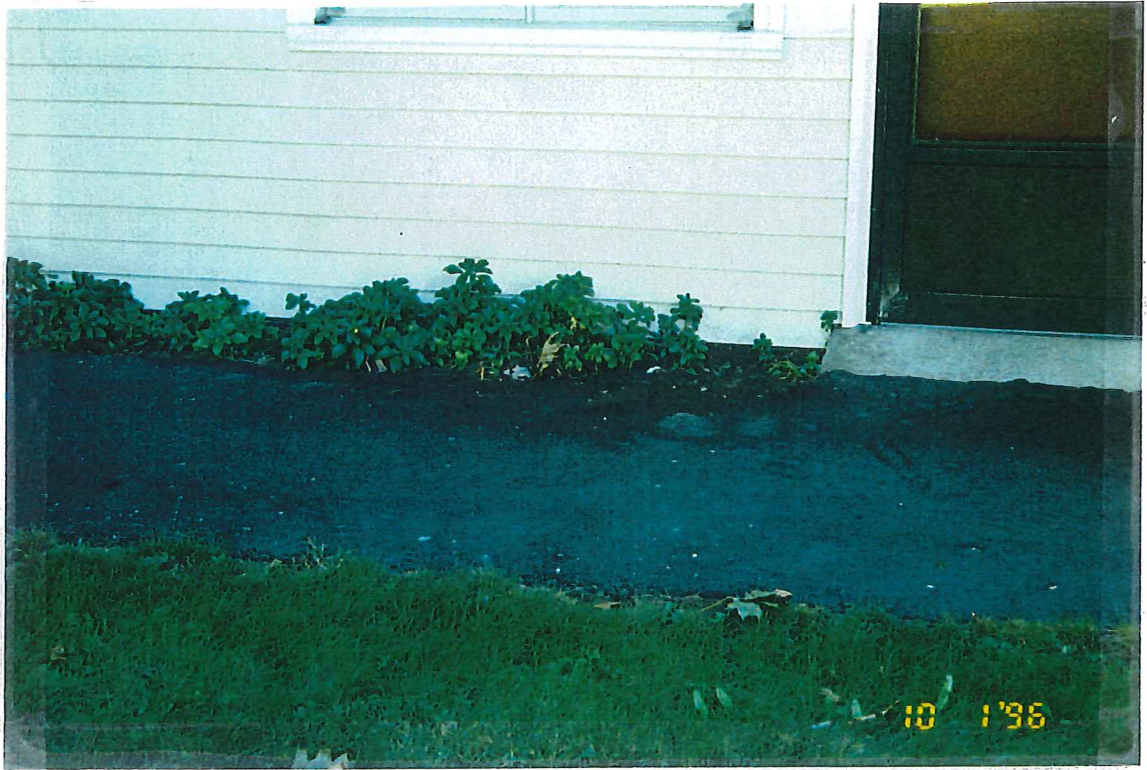
SIDING EXTENDS DOWN TO & BELOW GRADE.
