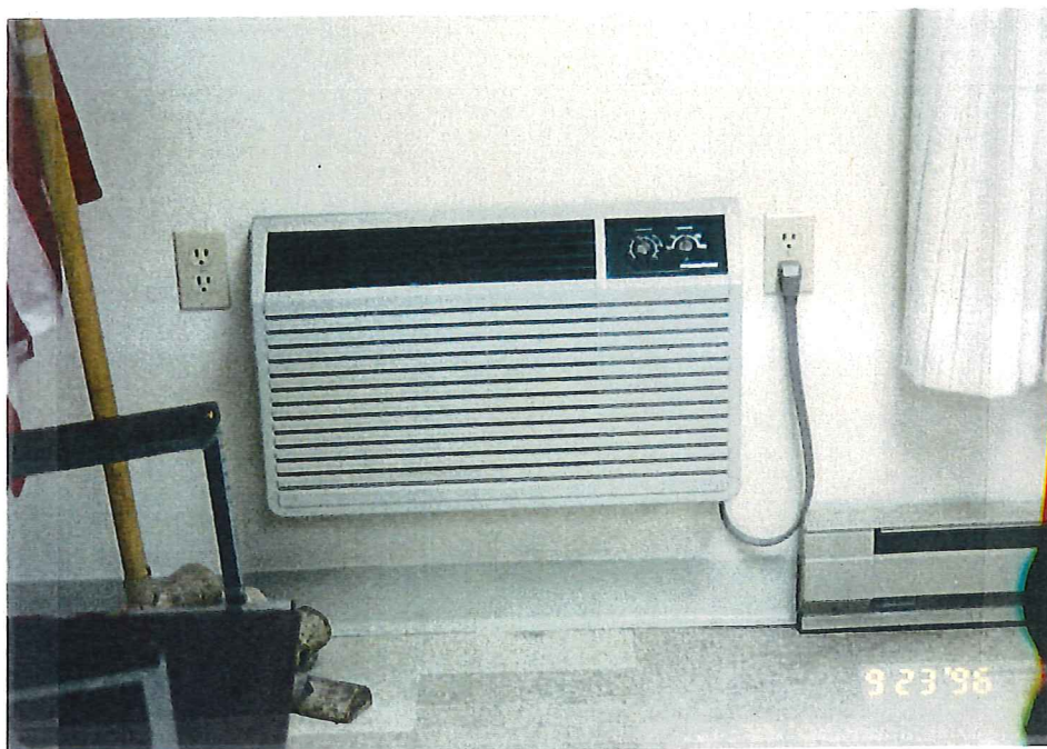
OUTLET TOO CLOSE TO BASEBOARD CONNECTOR.
