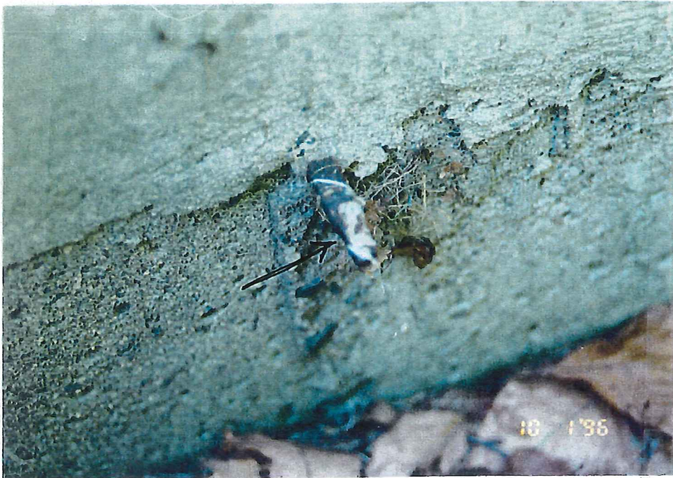
SHARP, PROTRUDING FORM TIE.
