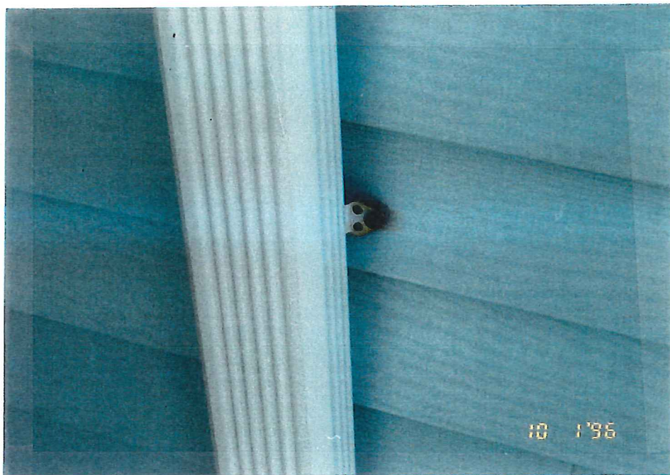
RUSTY GUTTER STRAP NAIL.
