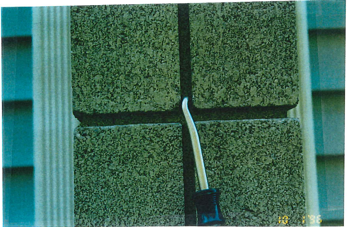
SMALL VOID IN MORTAR JOINT.
