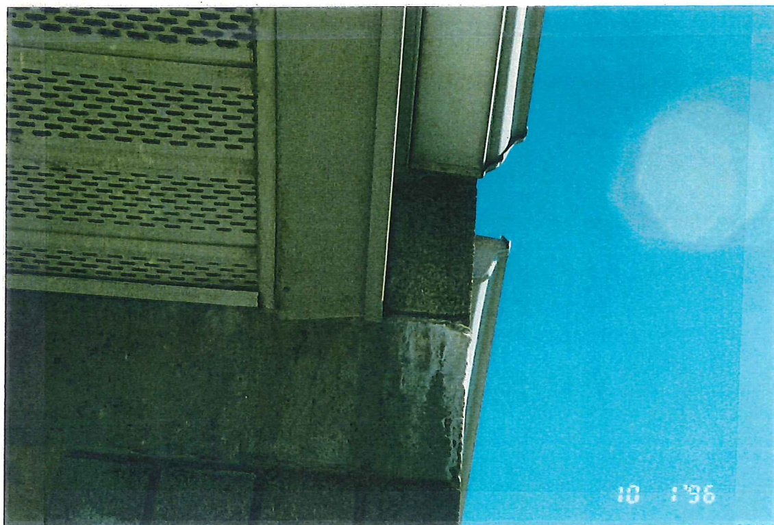
EFFLORESCENCE AT MASONRY PIER.
