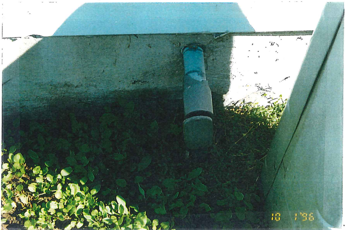
ELECTRICAL SERVICE COVER LOOSE.
