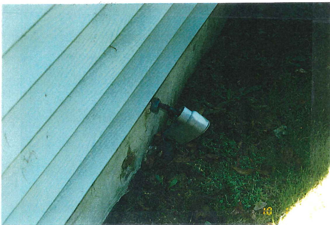
BROKEN ELECTRICAL ENTRANCE.
