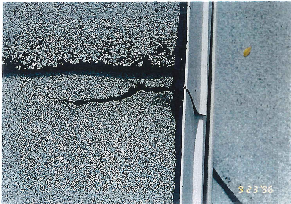
TEARS IN ROOFING.
