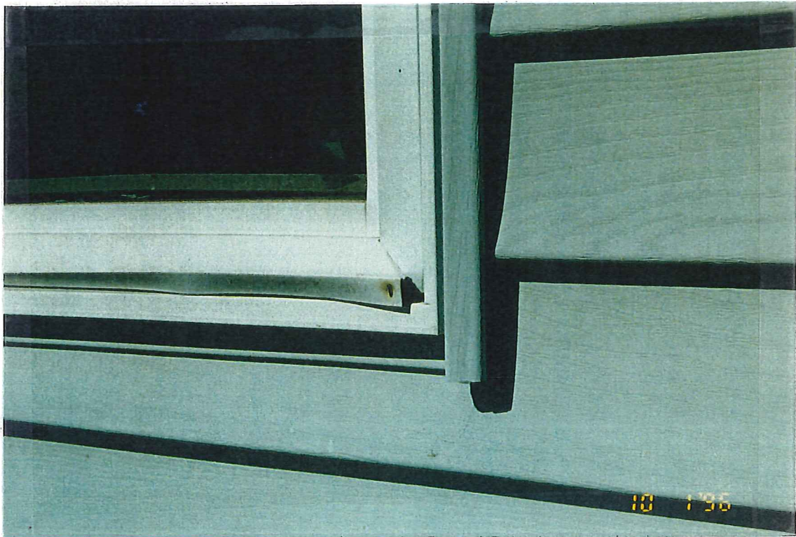
VINYL CLADDING LOOSE ON WINDOW.
