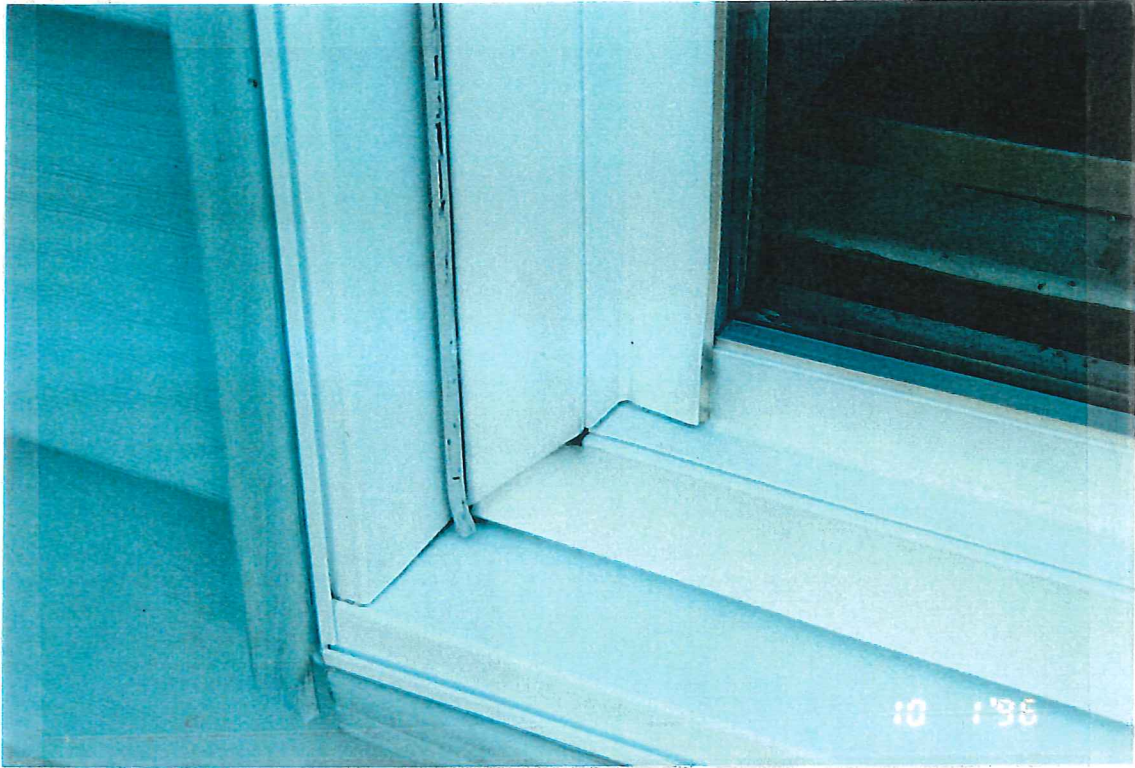
OPEN JOINTS IN WINDOW VINYL CLADDING.
