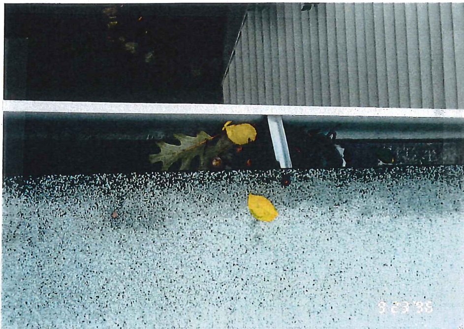
ROTTED DEBRIS IN GUTTER.
