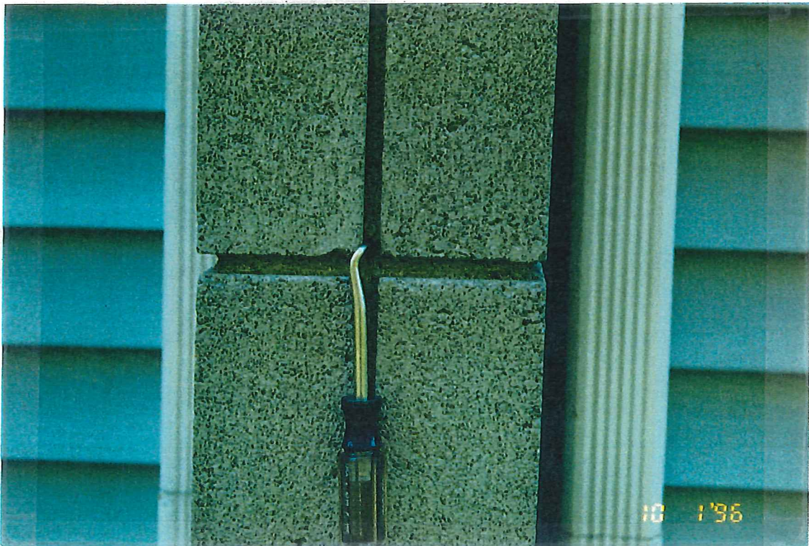
SMALL VOID IN MORTAR JOINT.
