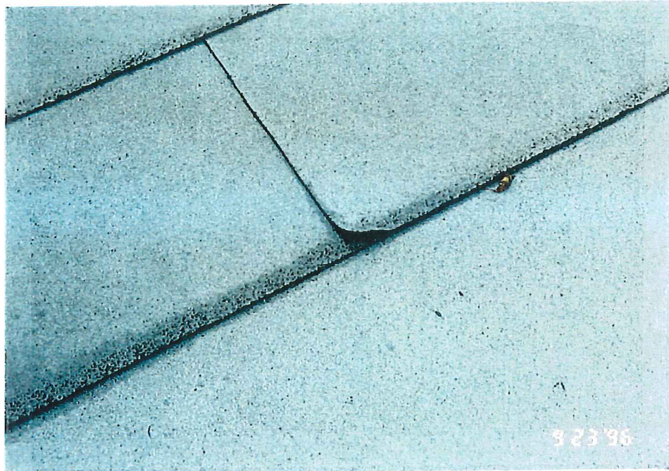
WARPED, LOOSE ROOFING CORNER.
