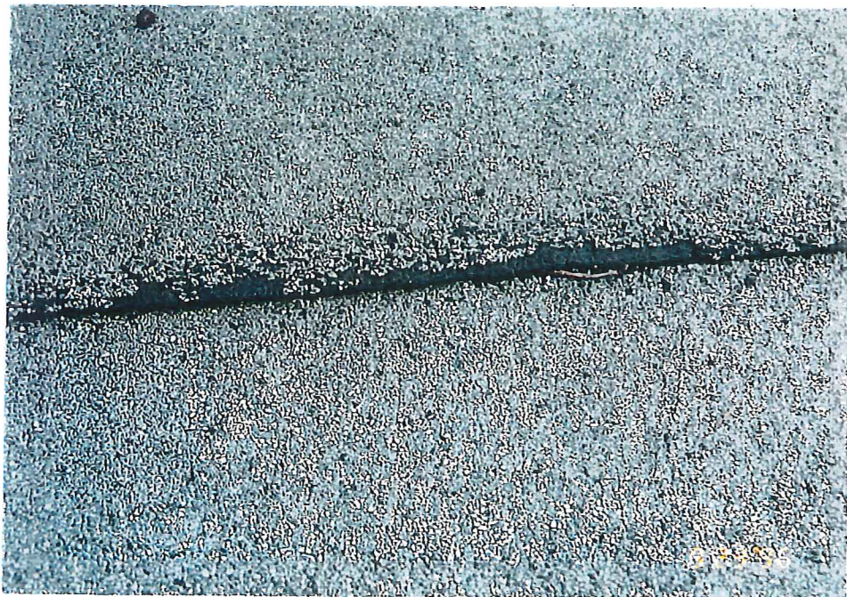
ERODED COATING ON ROOFING.
