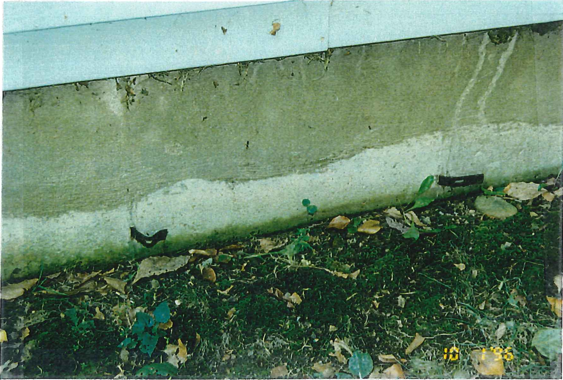
PROTRUDING RUSTY FORM TIES BENT BACK.
