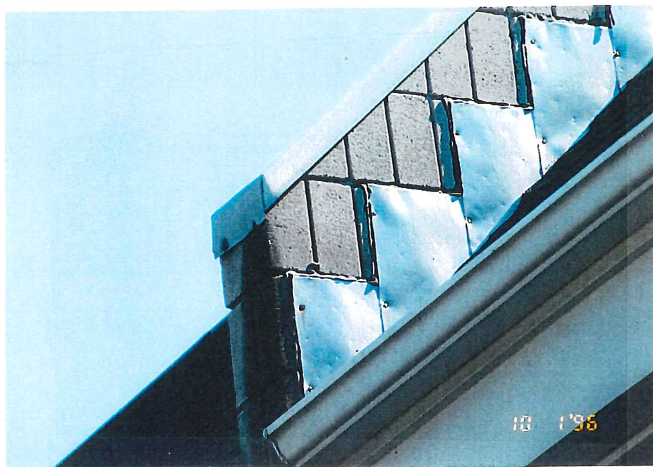
ROOF COUNTERFLASHINGS. NOTE STAINS ON LEFT FACE.
