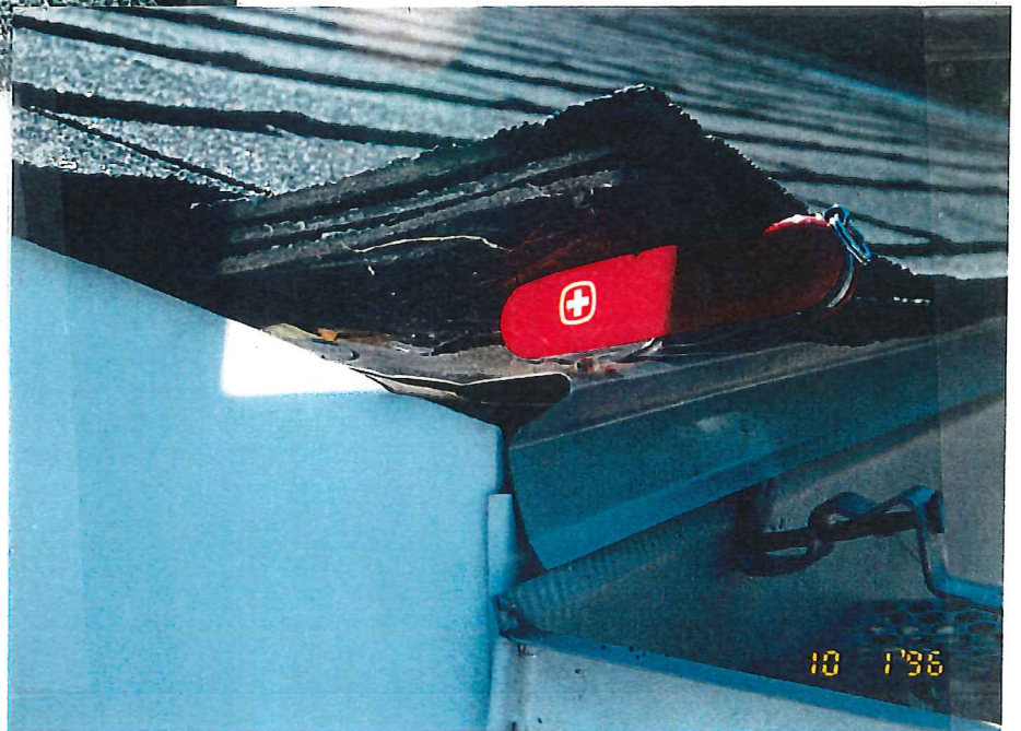
SHOWING PLYWOOD SHEATHING UNDER SHINGLES; NO UNDERLAYMENT OF EAVE FLASHING.
