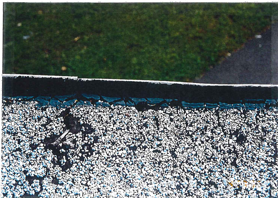
CRACKED ROOF EDGE SEAL; DISINTEGRATING ROOFING.
