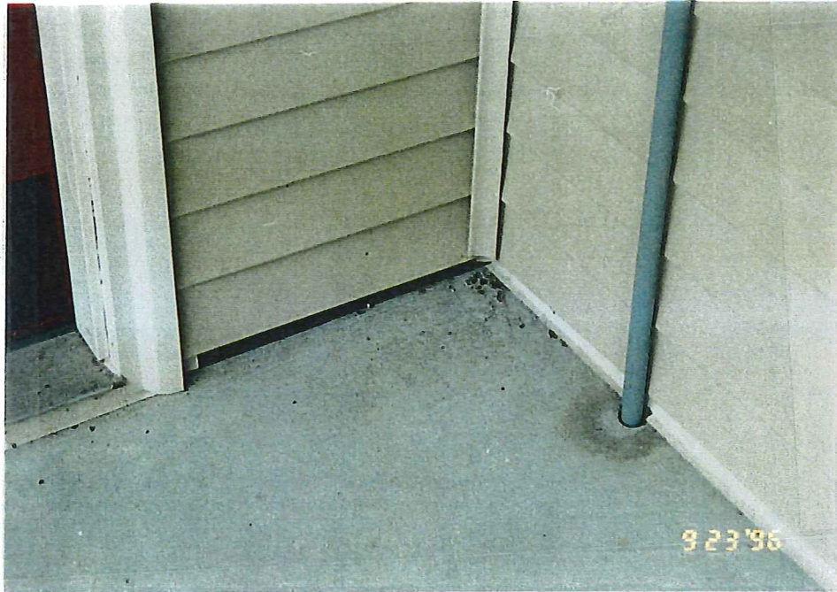
SIDING VERY CLOSE TO WALKWAY, SECOND FLOOR.
