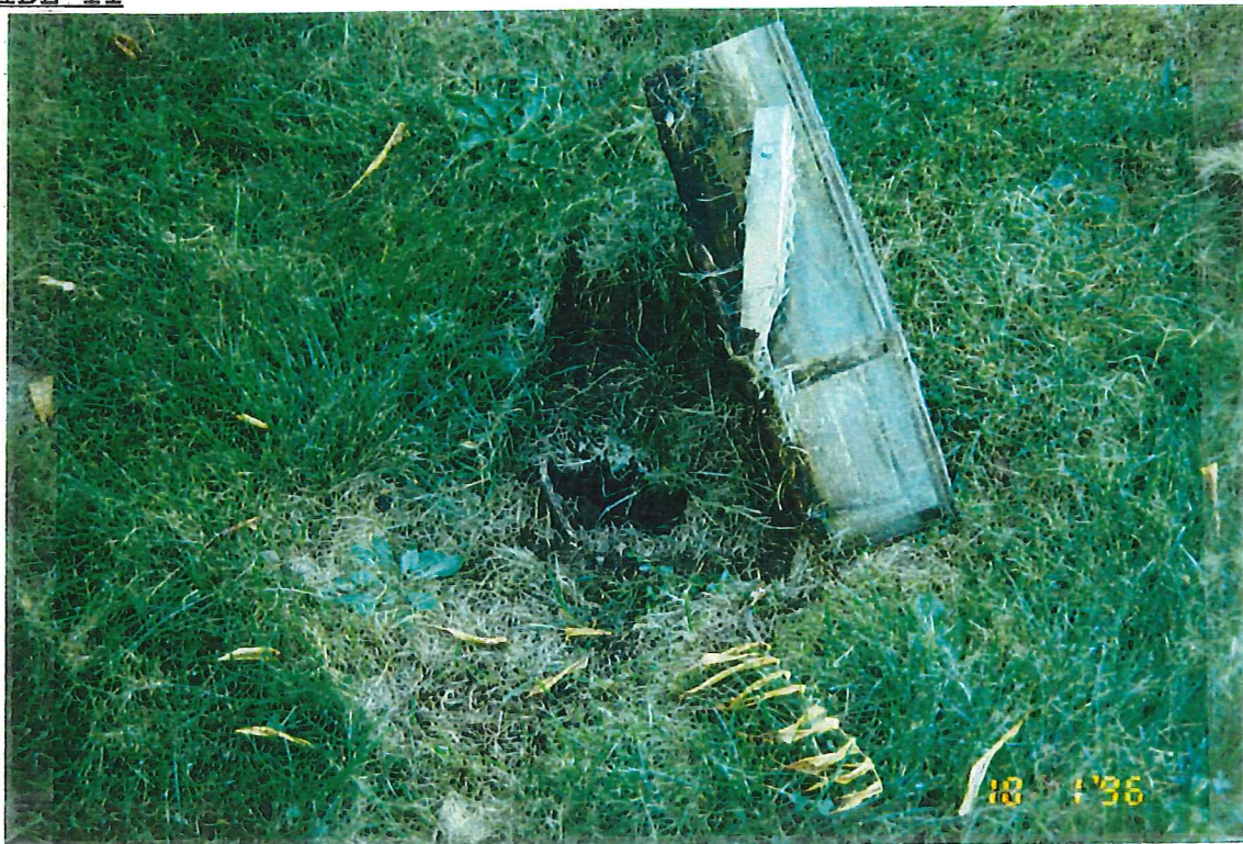
BROKEN PIPE COVERED WITH WOODEN BOX.
