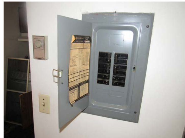
View of General Electric unit-level circuit breaker panel
