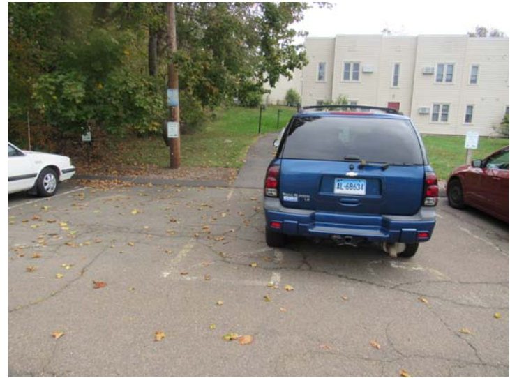
View of resident provided surface parking as seen towards west end of development –note cracking and faded/weathered striping
