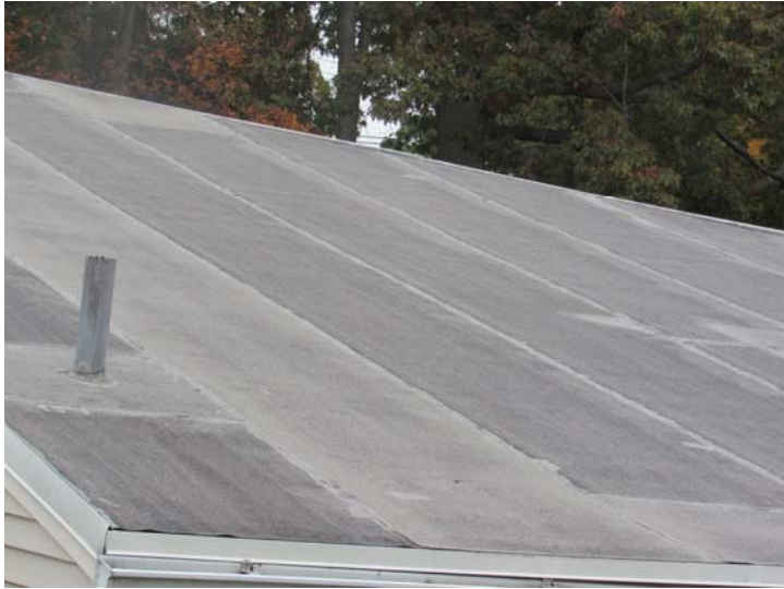
View of typical roofing system conditions – appears to be modified bituminous sheet membrane roof assembly from available vantage points
