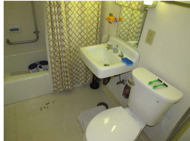
View of typical unit bathroom finishes and fixtures – isolated toilets appear to have been replaced in recent years
