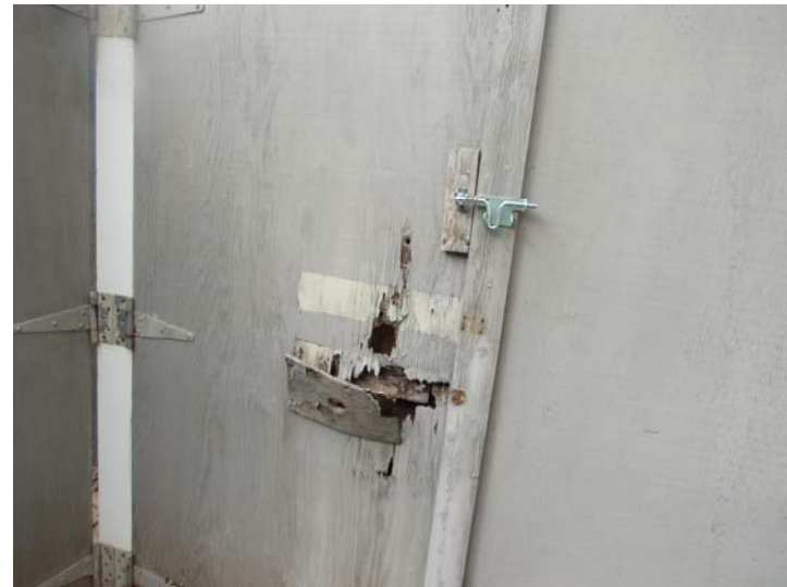
View of electrical closet wood doors exhibiting pronounced deterioration/weathering as seen at Building C
