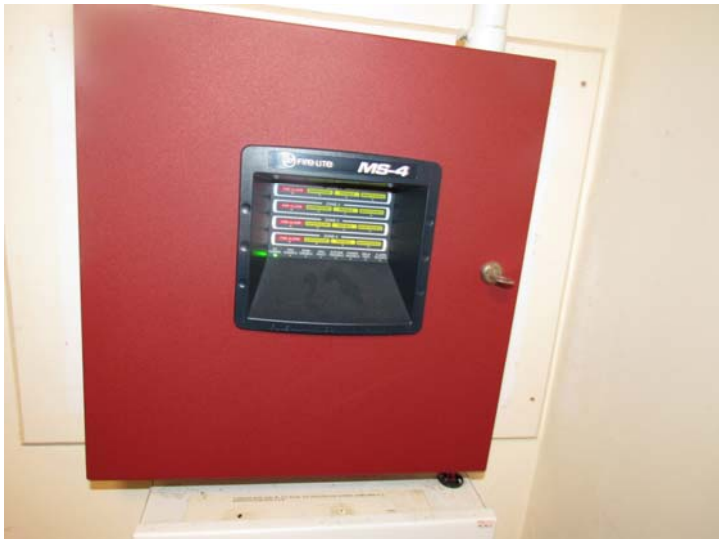
View of typical residential building central fire alarm control panel monitoring hardwired end devices – panel as seen at Building B
