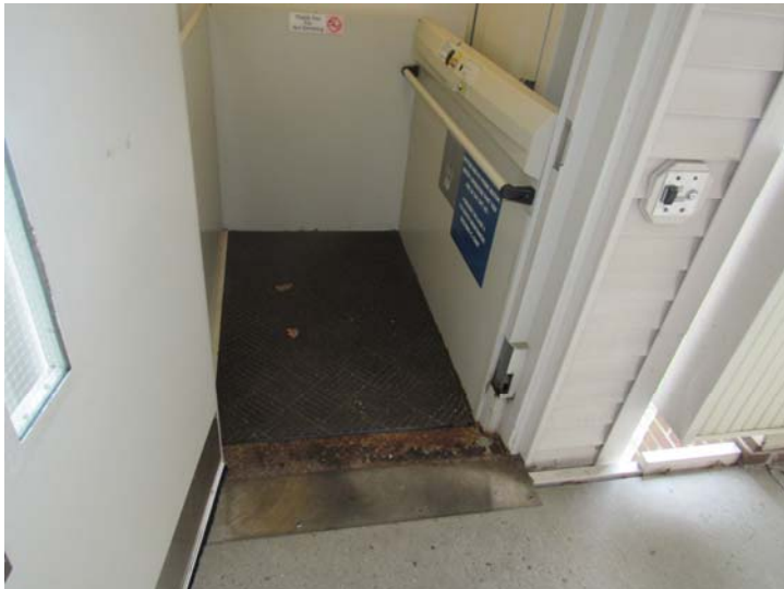
View of one of four vertical platform lifts serving residential buildings (i.e. 2 at Building C, and 1 each at Buildings A and B) – note corrosion at threshold
