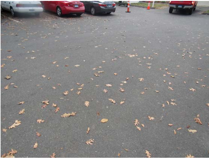
View of asphalt-paved surface parking area constructed at front of development off S Montowese Street
