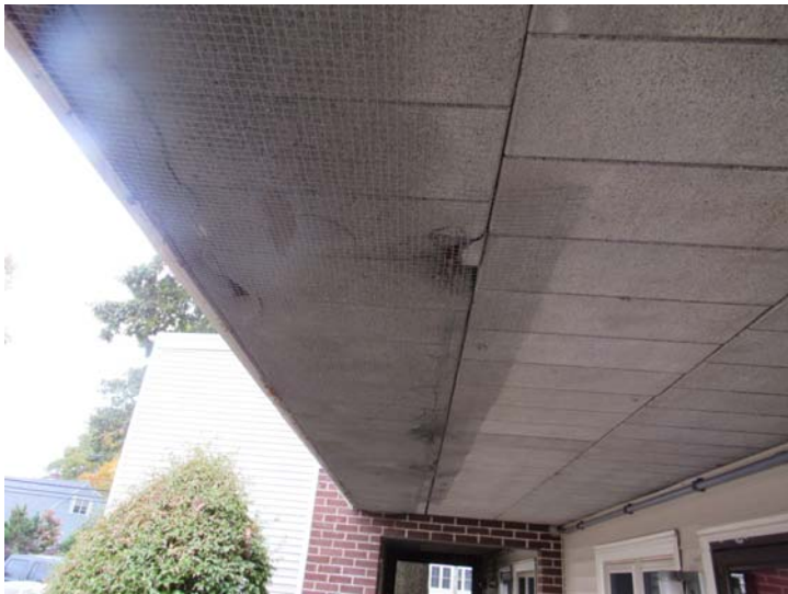
Additional view of concrete deterioration as seen at soffit/underside of second floor deck
