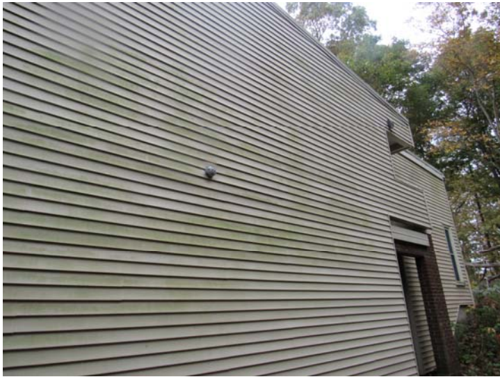
Localized staining from water-runoff observed on vinyl siding at buildings
