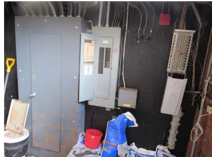
View of typical residential building main electrical closet containing service panel and distribution equipment
