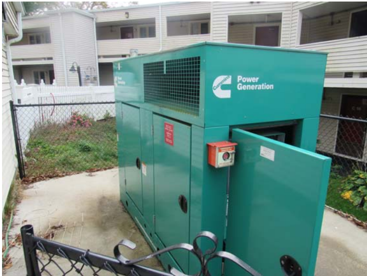
View of propane-fueled emergency generator serving community building in the event of a power failure
