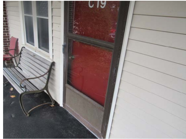
View of typical unit exterior entry doorway conditions – note oxidation on storm door
