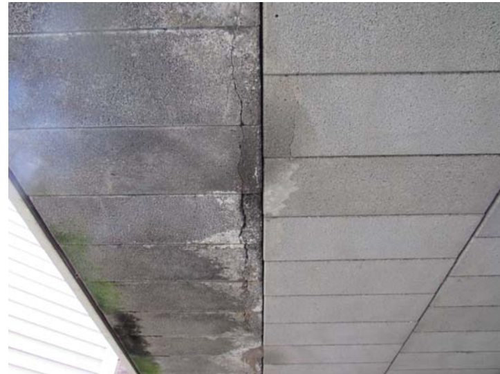
View of underside of second floor deck – concrete soffit exhibits widespread cracking/deterioration
