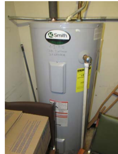
View of electric domestic water heater serving community building
