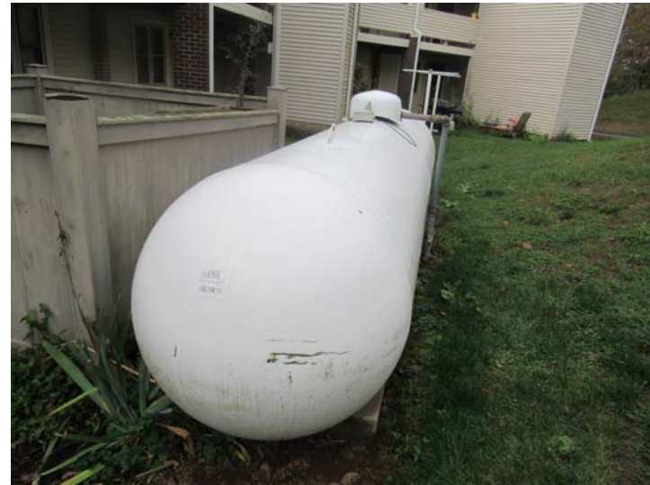
View of 1,000-gallon capacity propane storage tank serving emergency generator
