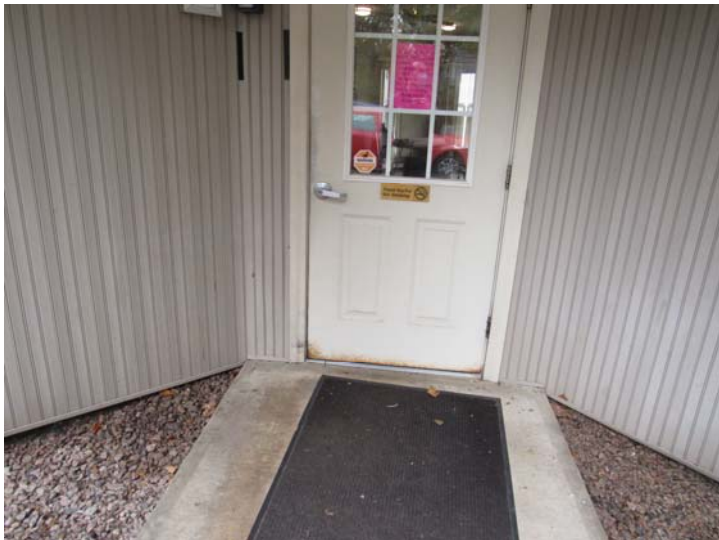
View of corrosion along base of community building main entry doorway
