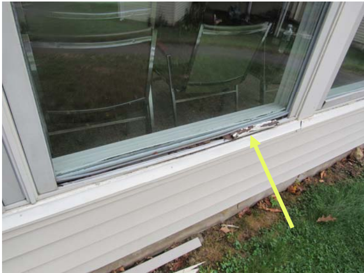
View of wood rot/deterioration as seen along base of community building exterior window
