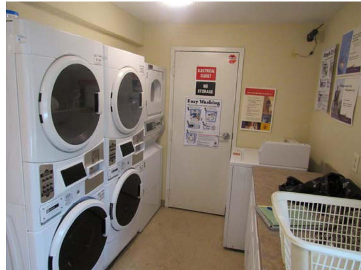
View of laundry room finishes and equipment
