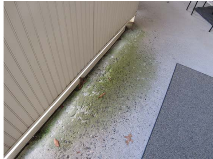
View of top surface of second floor concrete deck exhibiting surface scaling/deterioration – localized areas of cracking also observed
