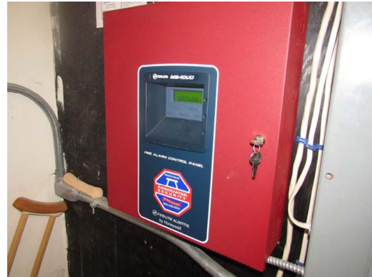
View of central fire alarm control panel monitoring hardwired end devices at community building
