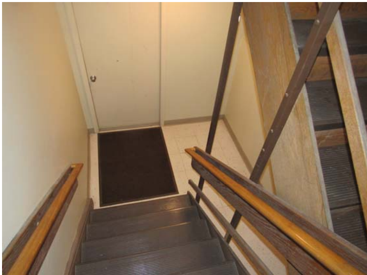
View of typical common stairway finishes – note stairway railings do not meet current safety standards
