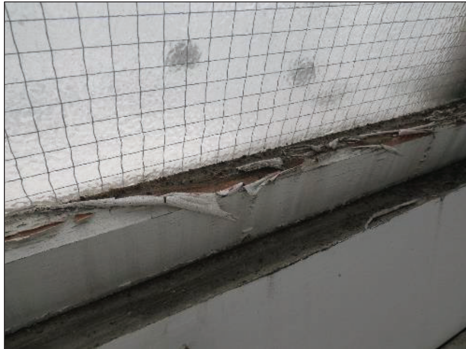
Windowsill of rafter clerestory windows, peeling paint, dust debris including supporting fungal spores, a condensation plane. These areas are too high for standard cleaning operations and require specialist access equipment.
