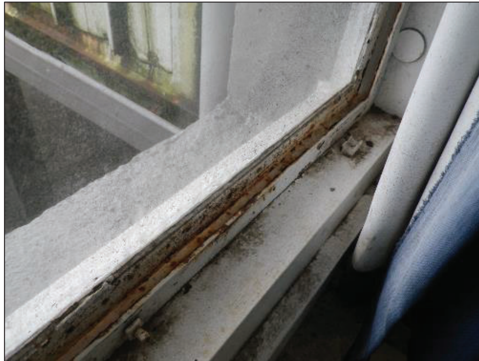
Corroding steel window frame. Slightly open allows saturated internal air to bleed to the exterior keeping the steel frame in a moist environment encouraging corrosion.
