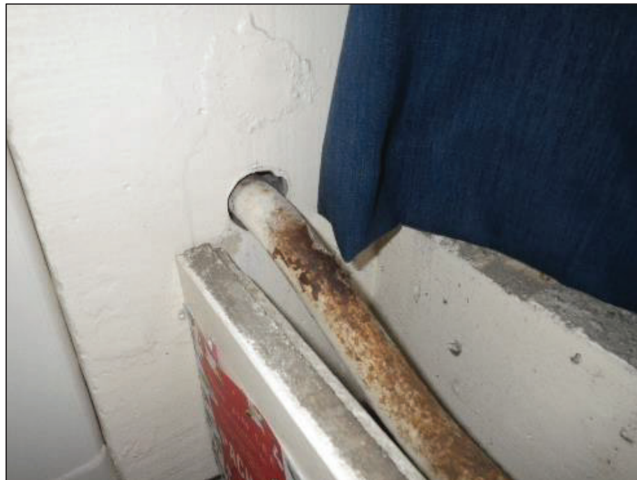
Surface corrosion to service pipes forming a condensation plane. Service pipes at pelmet level within the classrooms sit in the zone of moisture rich damp internal air.
