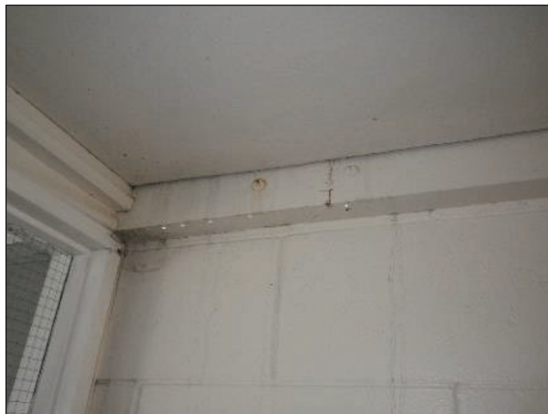
Water leaks into corridor from service void roofing drip onto the floor. There was light mist rain most of the day 29/3/2021.
