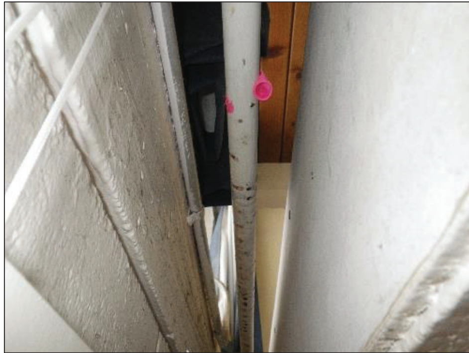
Lower face of same pipe showing water stain trails and drip point from the service pipe.
