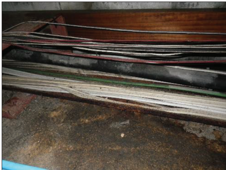
Corroded cable tray, electrical cables sitting in water. Decaying ceiling linings to walkway ceiling.
