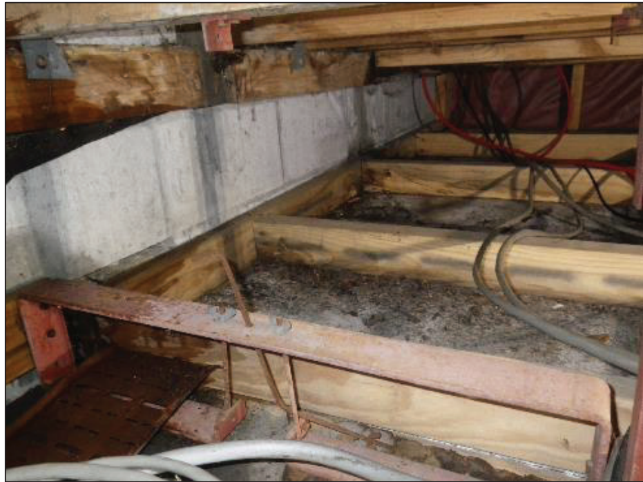
Repeated water damage in the service void ceiling.
