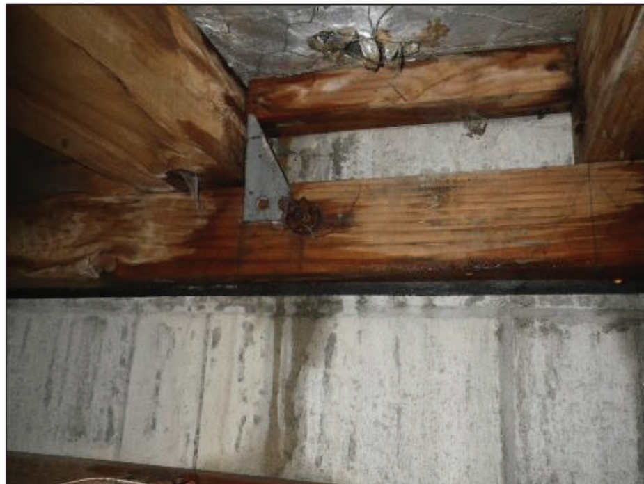
Water leaks corroding anchor bolts, saturating structural timber framing eventually end up at floor level. The leaks increase the moisture loading of the roof cavity leach timber treatments and encourage fungal decay. Foil roof underlay is non-breathable or vapour permeable.
