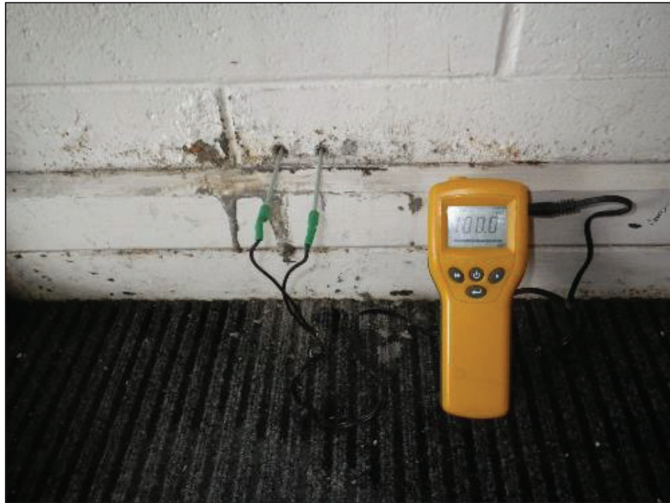
Saturated core to lower course of concrete blocks, corridor internal wall. Results of longstanding roof leaks.
