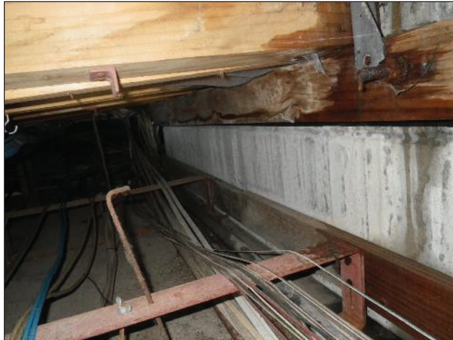
Corroding cable trays and steel hangers, corroding bolt fixings to framing, saturated framing timbers, 50 years of dust debris in service ceiling cavity.
