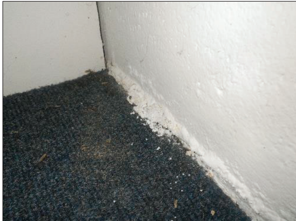
Efflorescence bleed from saturated concrete blocks, results of longstanding roof leaks.
