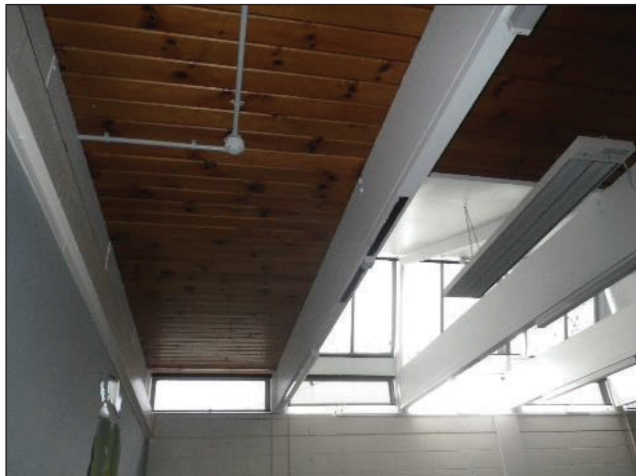
Roof areas of the classrooms with elevated rafter clerestory roof windows and lower pitched flat roof areas, roof mass only 100mm deep in general.
