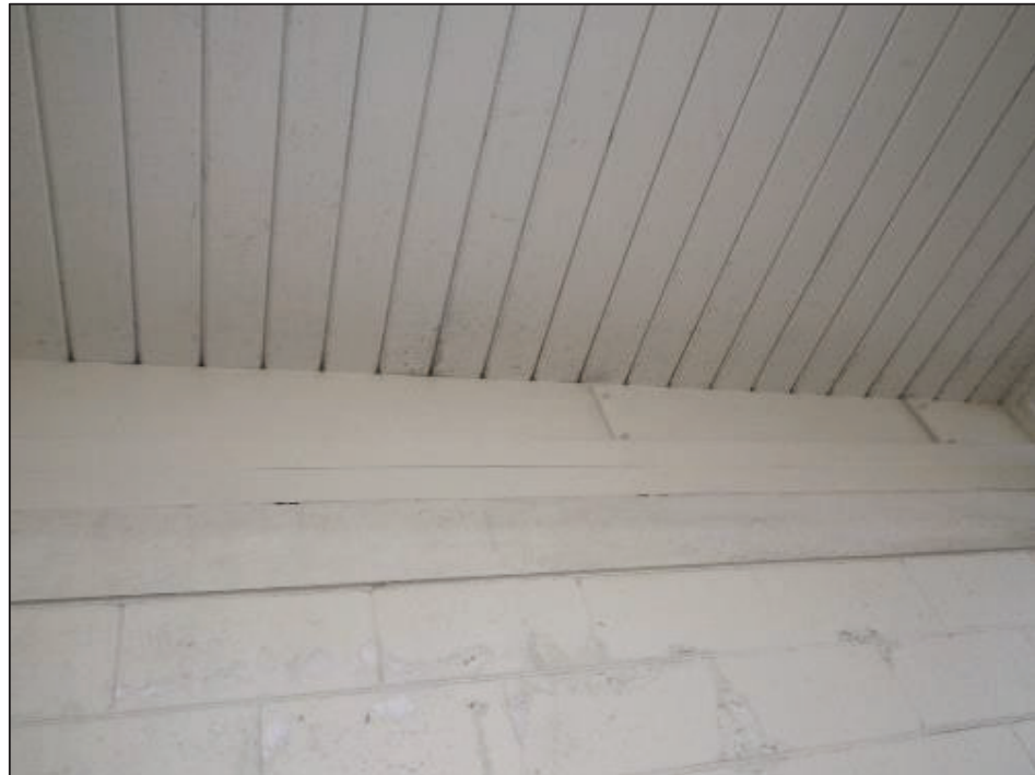
Ceiling / roof forming condensation plane in bathrooms. Discolouration is fungal growth on the ceiling surface.
