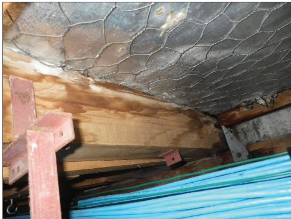
Foil roof underlay non-breathable traps moisture vapour, moisture damage to roof framing, active leak zone.
