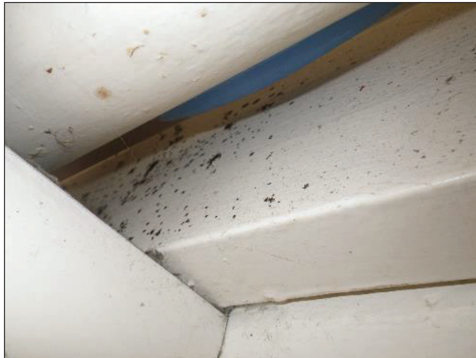
Fungal spotting to surface in roof area with passing moist air in the bathrooms.
