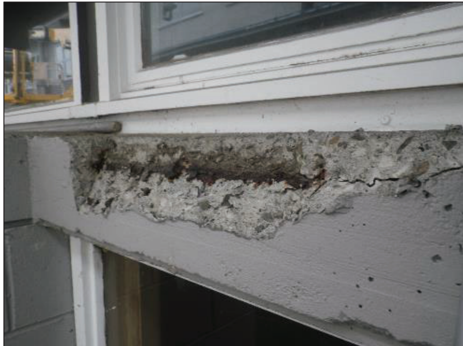
Localised spalling of concrete through sections of the bond beam due to insufficient concrete cover allowing moisture entry and resulting corrosion.
