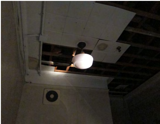
A136 Typical Light Fixture
