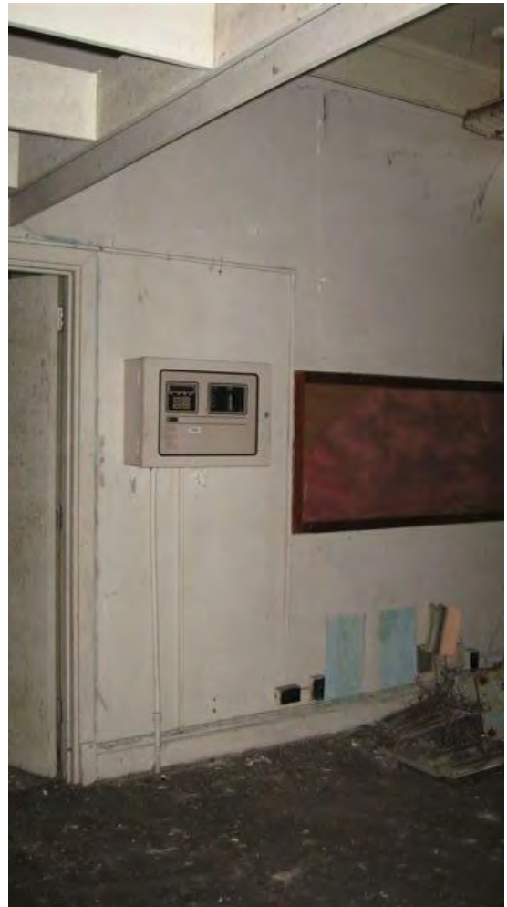
A129 Clock System Control Panel
