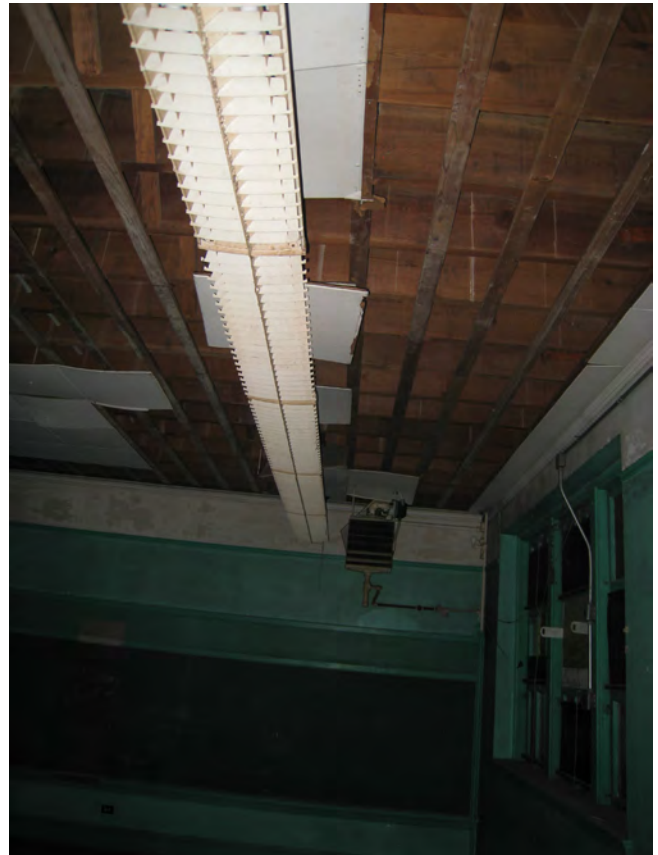
E03 Non-Functioning Lighting
