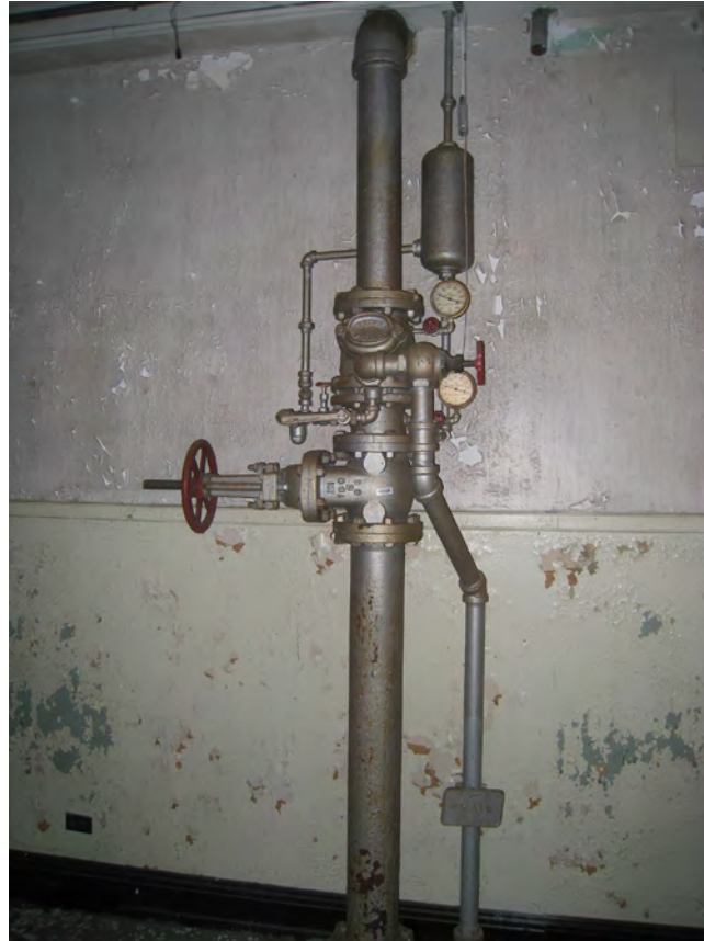
FP01 Non-Functioning Sprinkler Rig
