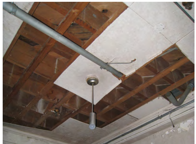
E04 Non-Functioning Components
