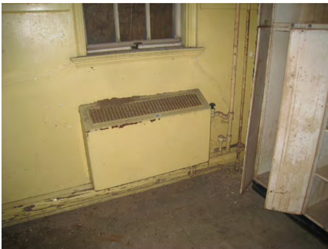
M03 Non-Functioning Radiator
