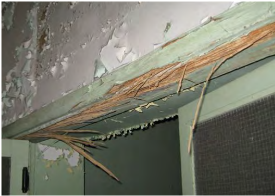
A107 Termite Damage at Door Frame
