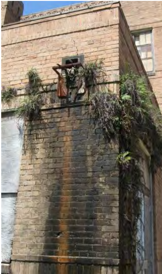
A28 Plant Growth in Masonry at Boiler Room
