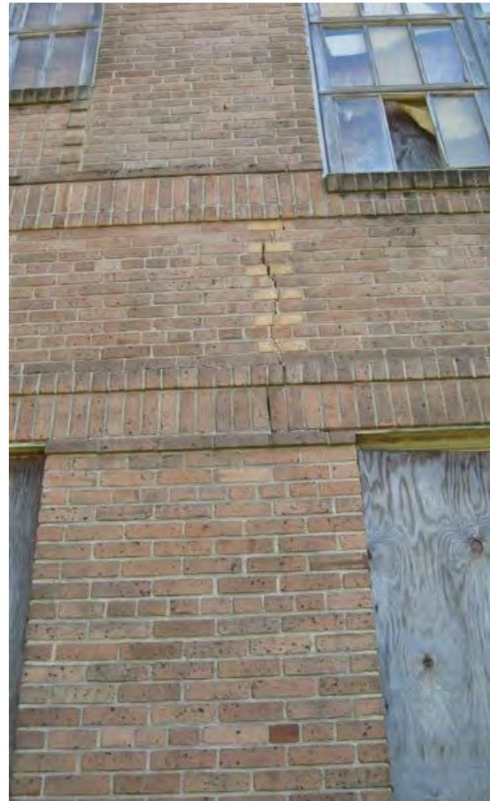
A12 Masonry Crack at Northwest Façade
