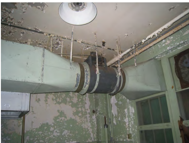
M05 Non-Functioning Fan
