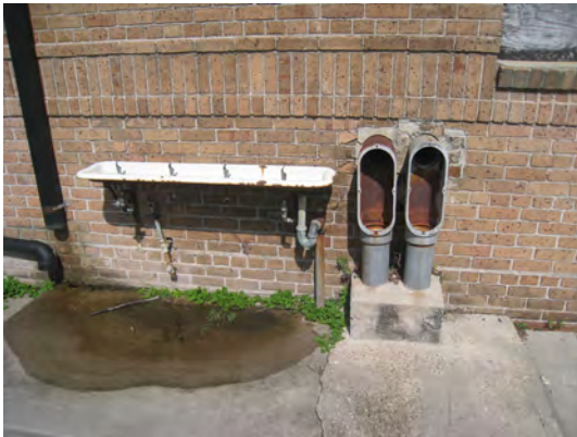
P01 Non-Functioning Storm Water
