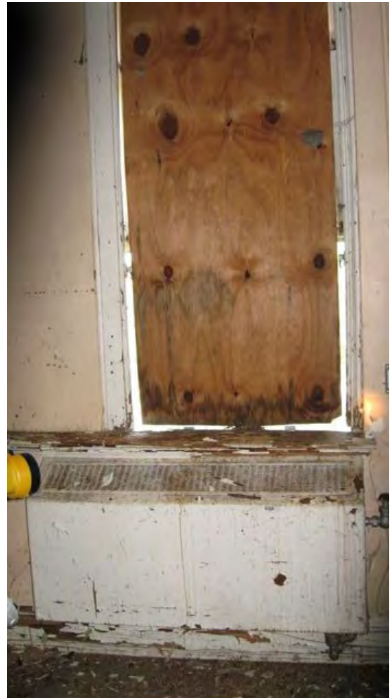
A127 Termite Damage at Window Stool
