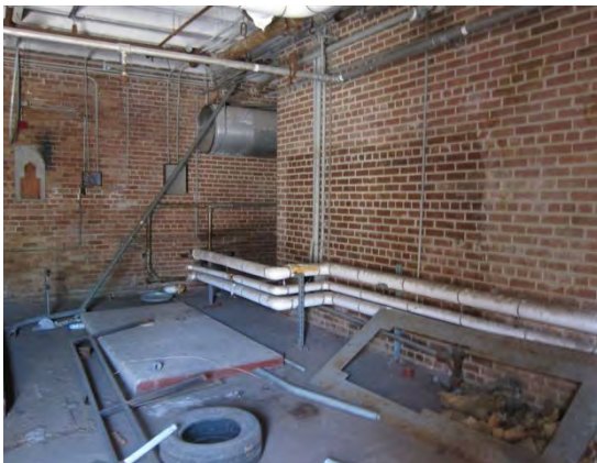
A122 Boiler Room
