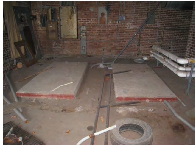
M02 Missing Boilers
