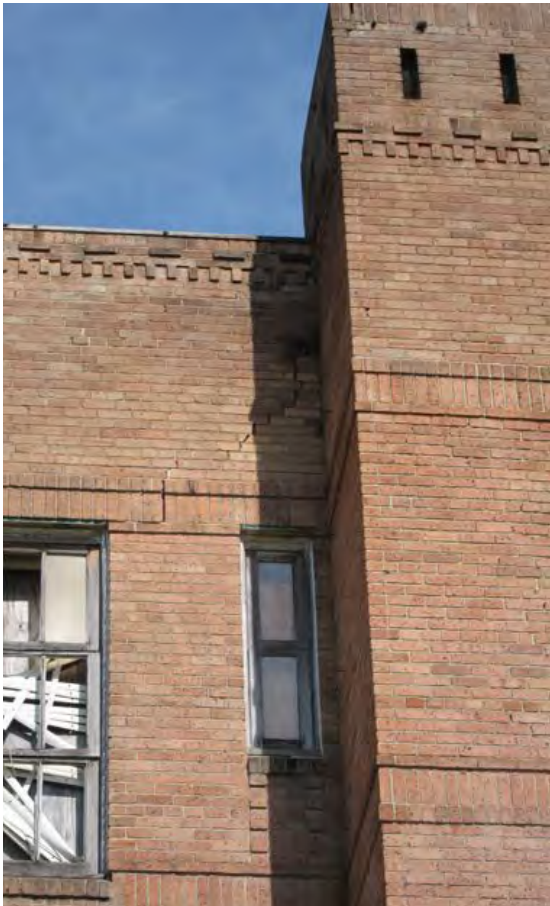
A51 Masonry Cracking Adjacent to Boiler Stack
