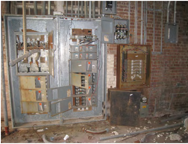
E01 Gutted Power Distribution
