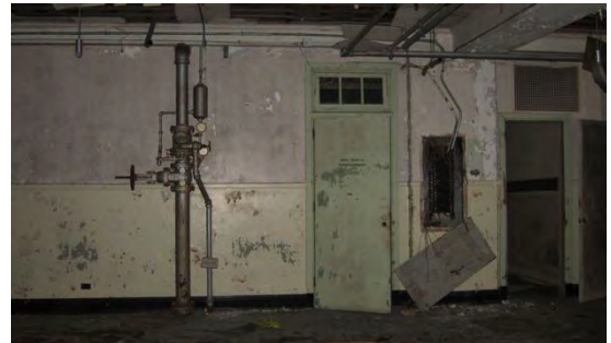
A119 Typical Exposed Sprinkler and Electrical at Cafeteria
