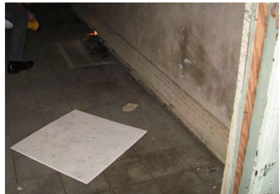
A106 Settlement at First Floor Slab
