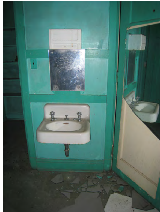
P02 Non-Functioning Sink
