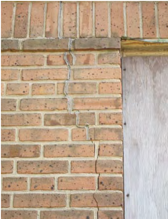
A36 Masonry Crack Adjacent to Window
