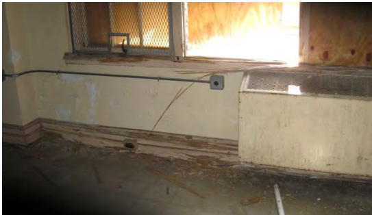
A118 Termite Damage at Interior Woodwork
