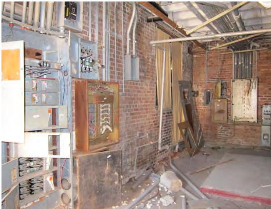
A123 Boiler Room
