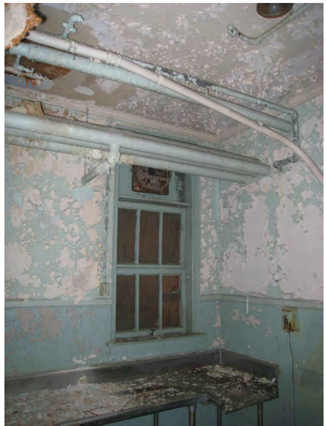
M04 Non-Functioning Piping
