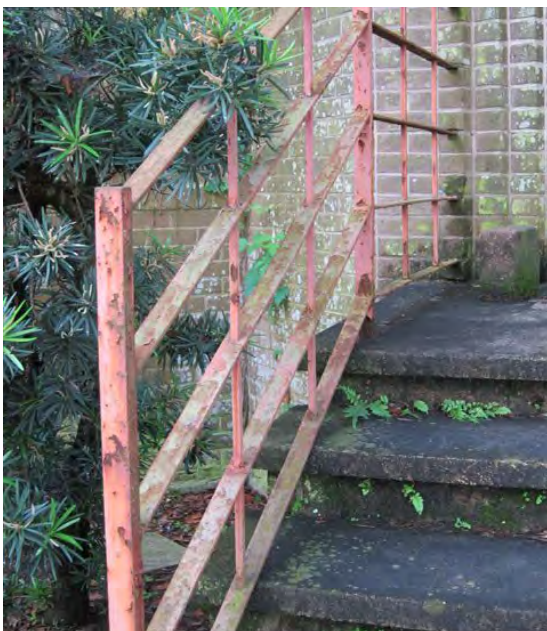
A14 Handrail at Main Entry
