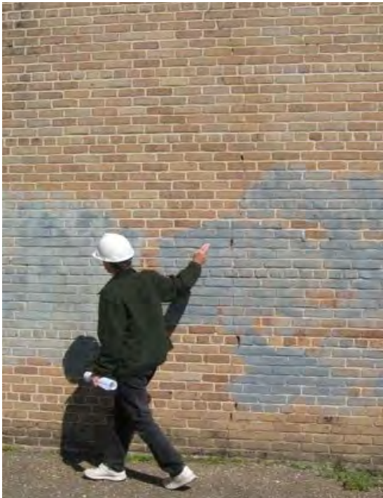
A42 Masonry Cracks in Gym Wall
