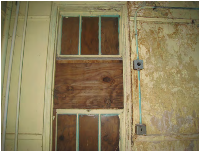
M01 Missing Window Unit
