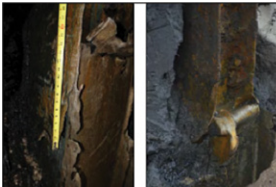
Photograph of bridge footing corrosion resulting from fly ash. Wisconsin Dept of Trans 1-43 Leo Frigo Memorial Bridge Investigation Report ID 1220-15-01. August 27, 2014.
