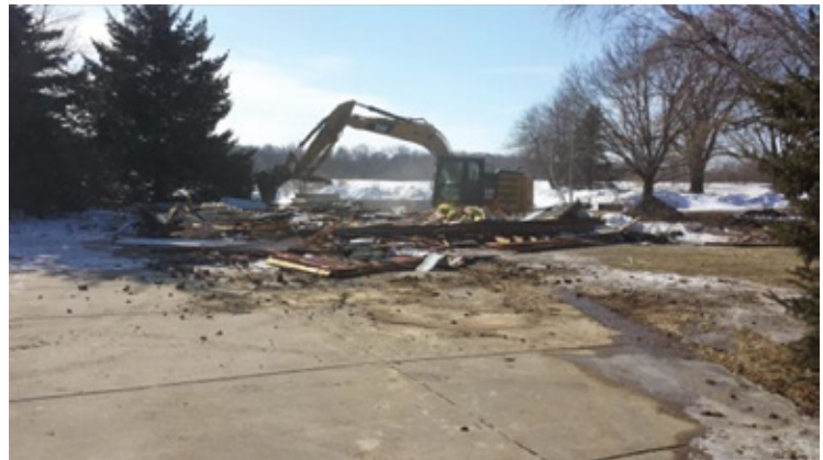
Photograph of house demolition near the Oak Creek Power Plant. Caledonia Wisconsin. January 2014.
