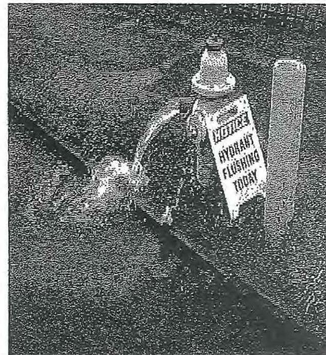
Flushing out discolored water
