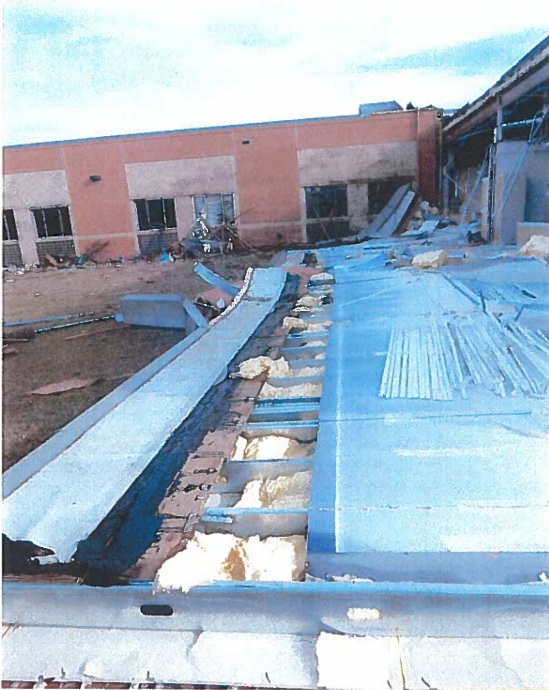
Photo #2: Example of exterior non-load bearing wall damage.
