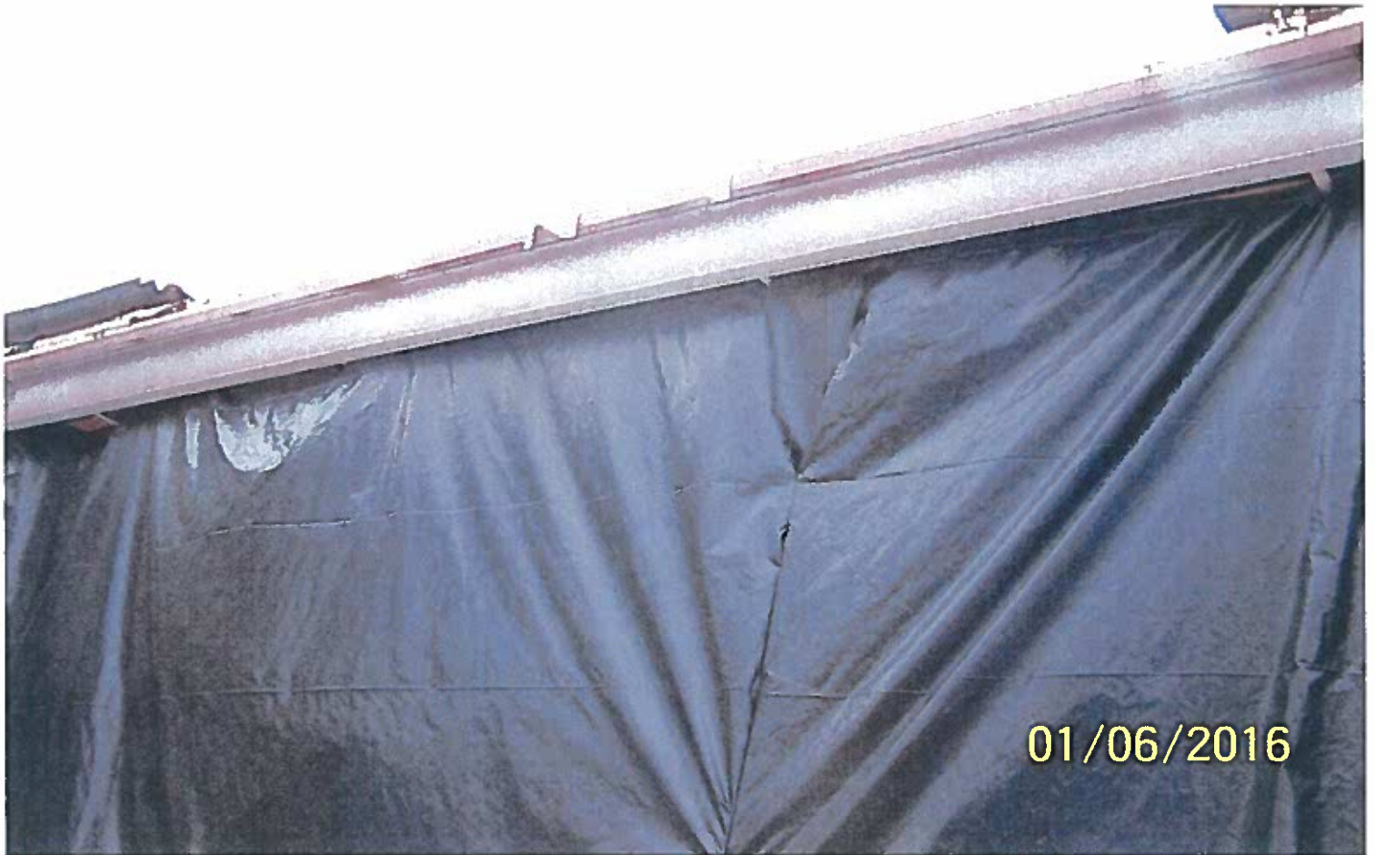
Photo #11: Another example of studs not being attached to clips which may have added additional load on adjacent connections.
