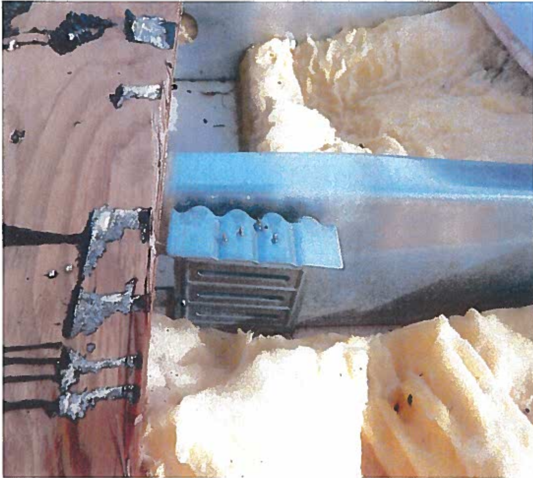
Photo #13: Example of improper installation, and not enough fastener penetration into steel causing connection failure. Missing screws from clip to studs.
