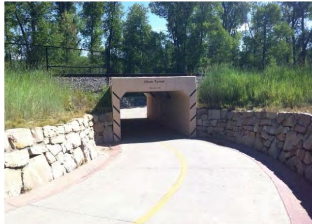
Figure 135: Trail underpasses separate trail users from motor vehicle traffic and/or rail traffic, reducing delays for all users.
