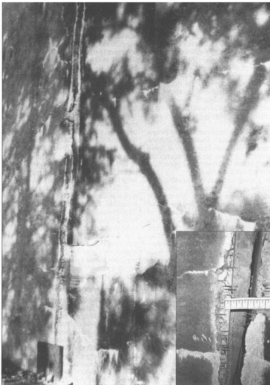
A wire-wound posttensioned concrete tank, constructed in 1964 by alternate pours of the vertical panels, in the La Purissima Water District emptied because of the collapse of its column-supported roof slab and the opening of one of the vertical panel joints (inset) after the earthquake.
