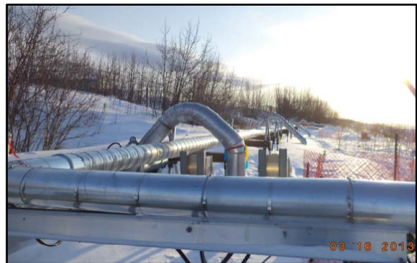
LTMA - Refinery Bank Gathering System
