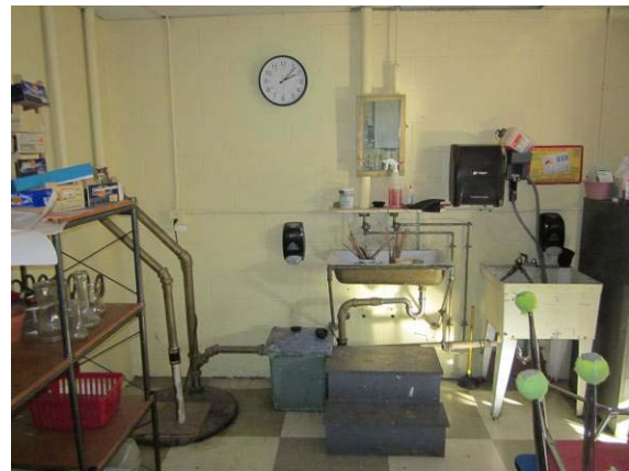
Art room plumbing fixtures
