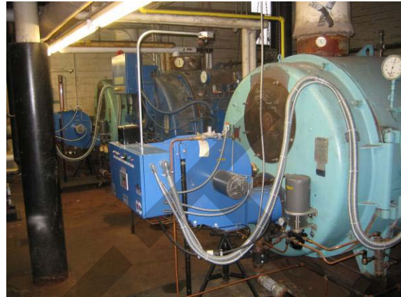
Deering High School boilers
