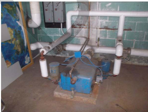
Electric steam condensate pumping station
