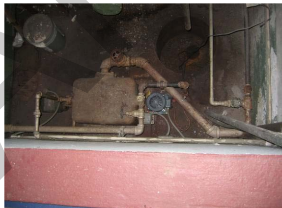
Electric steam condensate pumping station
