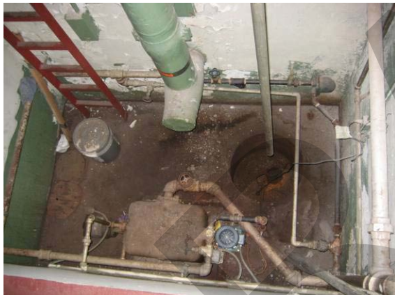
Underground steam piping
