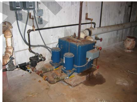
Electric steam condensate pumping station
