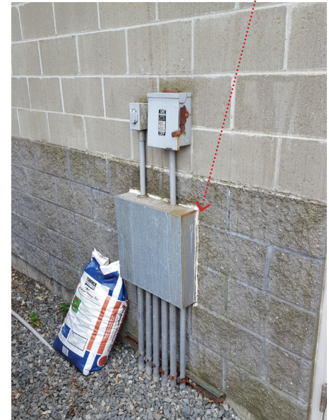
Fig. 074. Exposed Electrical Switching
