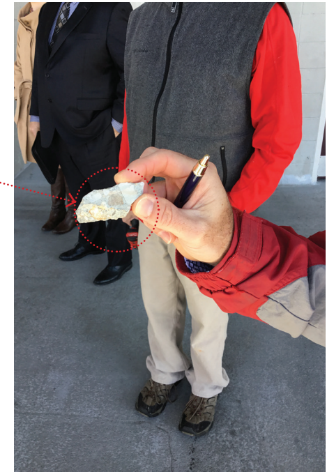
Fig 043. Example of Spalled Concrete
