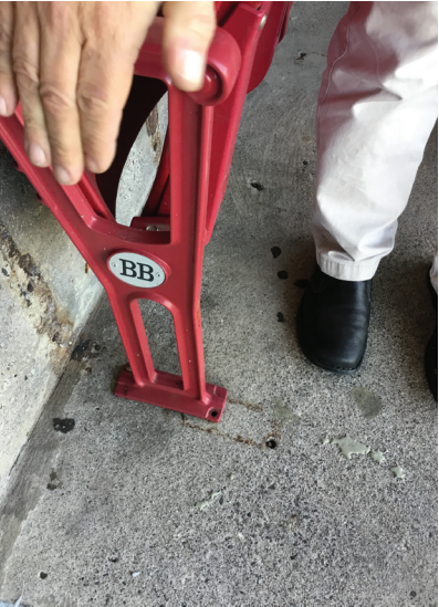
Fig. 109. Missing Fixed Seating Hardware
