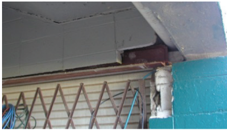
Fig. 046. Failing Lintel Support
