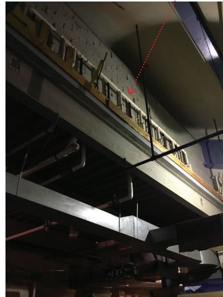
Fig. 061. Exposed PVC Piping @ Rear Of 1999 Toilet Room Addition
