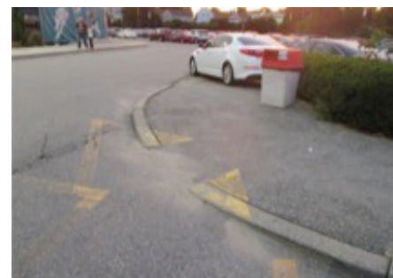
Fig 026. Example of Missing/Deteriorated Striping
