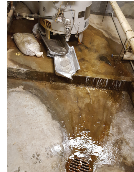
Fig. 055. Actively Leaking Domestic Hot Water Heater
