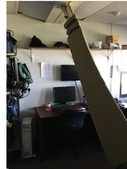
Fig. 130. Head-Knock Condition @ Press Box
