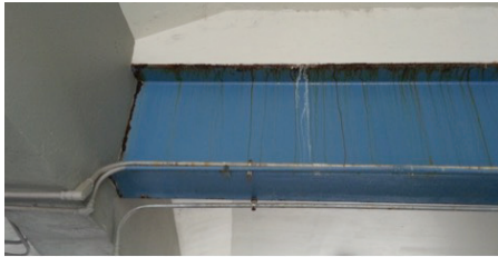
Fig. 045. Tower Ramps - Steel Beam Corrosion
