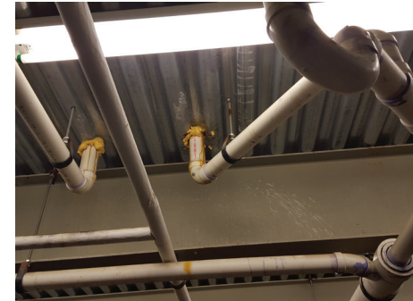
Fig. 062. Areas Of Water Infiltration @ Deck Drains
