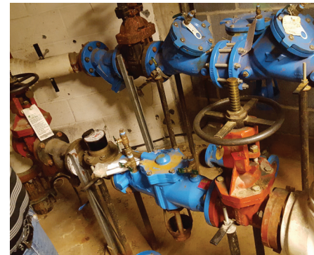
Fig. 054. Water Service Entry W/ Non-Potable Water Branch In Foreground - Note Corrosion
