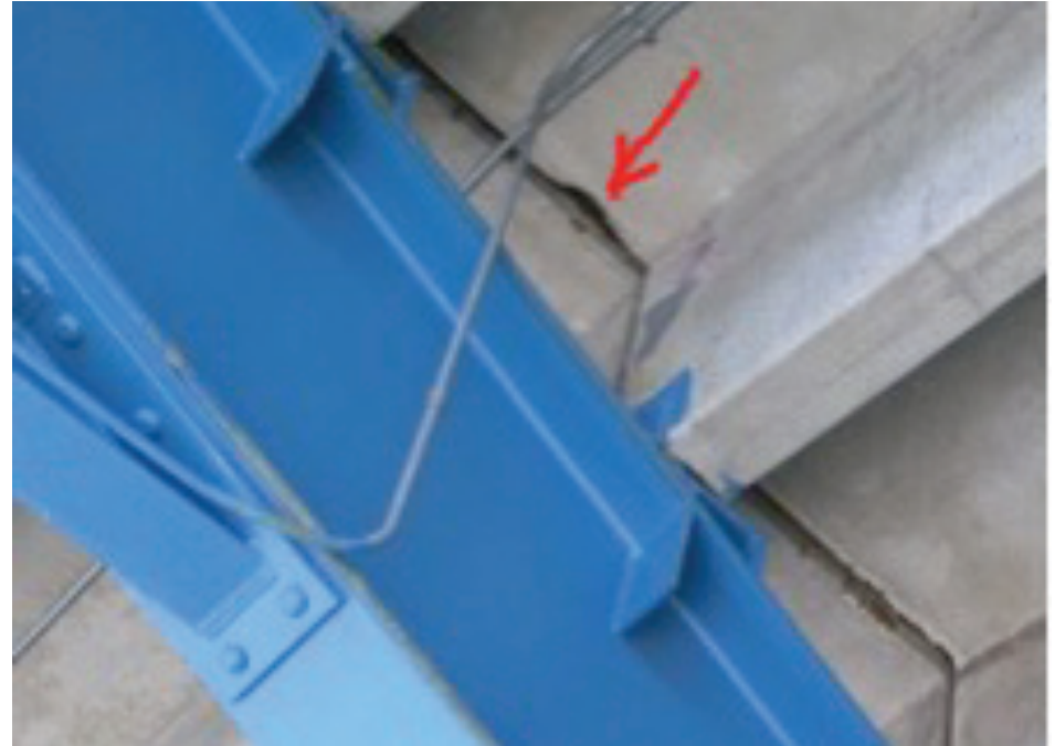
Fig. 049. Shims Involuntarily Moving
