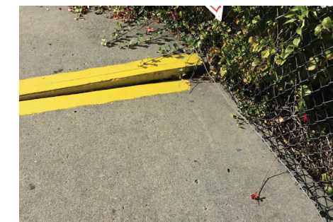
Fig 027. Example of Pavement Differential Settlement
