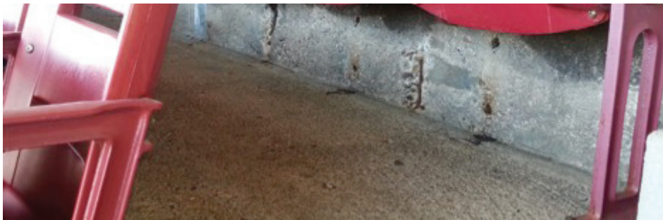
Fig. 048. Exposed Rebar - Rust/Corrosion
