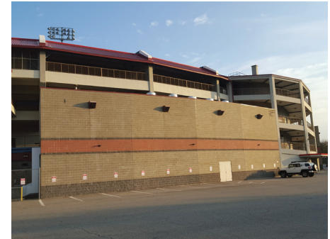
Fig. 073. Example of Inoperable Wall Packs
