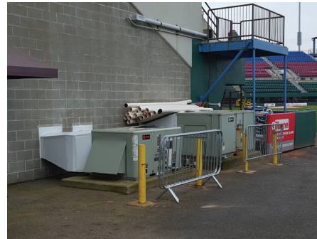
Fig. 071. Exposed HVAC @ Field Access Area
