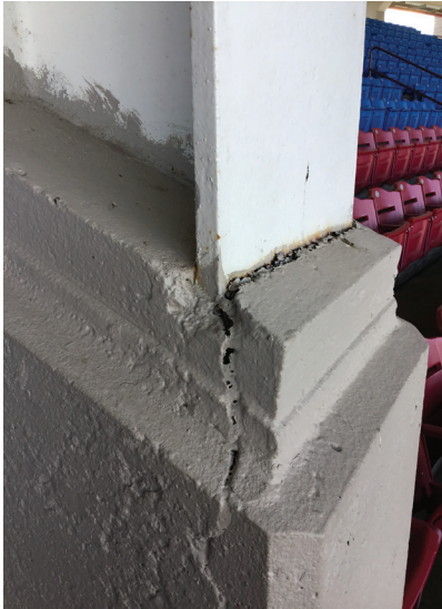
Fig. 105. Cracked Concrete = Water Entry
