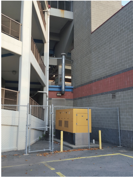
Fig. 056. Domestic Hot Water Heater Vent Termination Below Roof And Above Walkway - Note Proximity To Generator
