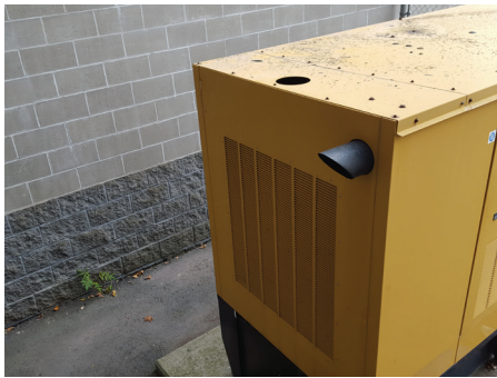
Fig 058. Generator Exhaust To Be Extended To Roof
