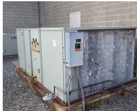
Fig. 053. 1998 Vintage On-Grade AHU - Damaged Coils & Corrosion - Note Pressure Relief Vents & Gas Regulators
