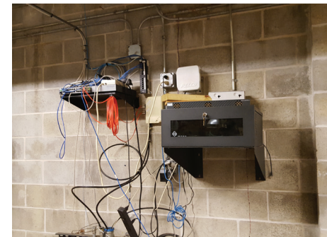
Fig. 064. Technology Equipment In Electrical Room
