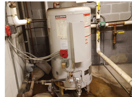
Fig. 063. Boiler Scheduled For Replacement - Much Sooner Than Typical (6 Years Old)
