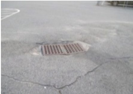
Fig. 019. Sample Deteriorating Basin
