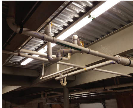
Fig 057. PVC Plumbing Piping Exposed within The Out-Building Electrical Room
