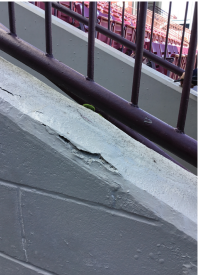
Fig. 110. Moss Growing Due to Standing Water
