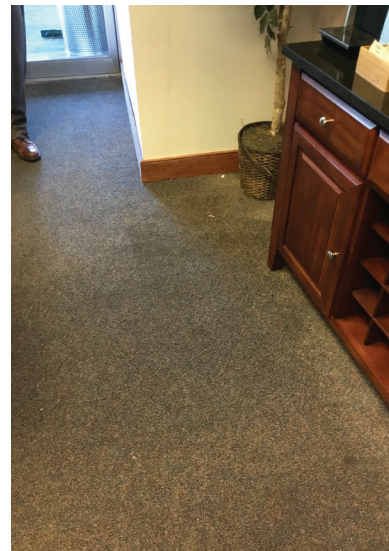
Fig. 127. Water Infiltration = Damaged Carpet
