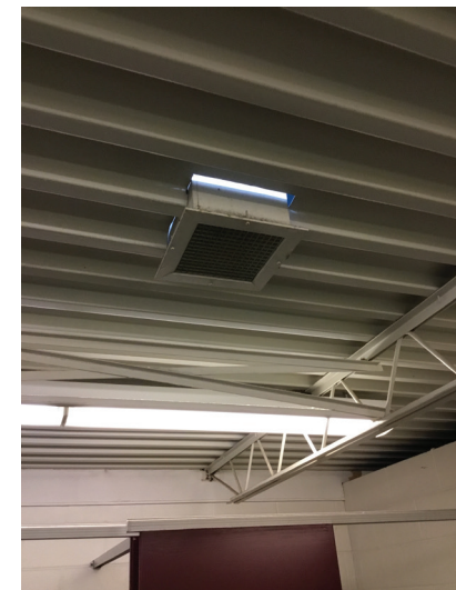
Fig. 172. Enclosed Areas Not Weather Tight
