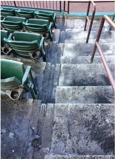
Fig 106. Example of Expansion Joint Condition
