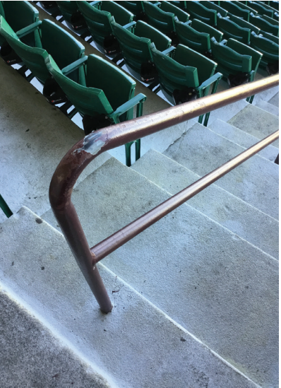
Fig. 111. Dangerous Railing Conditions
