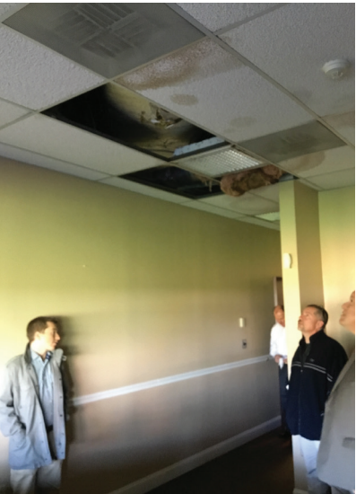
Fig. 108. Major Water Damage At Suites
