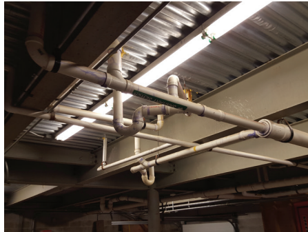
Fig. 059. PVC Plumbing Piping Exposed within The Out-Building Electrical Room
