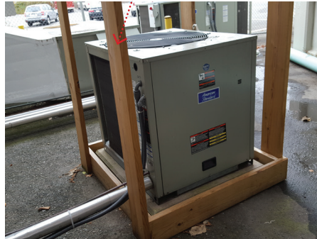
Fig. 067. Example Of At Grade HVAC Unit
