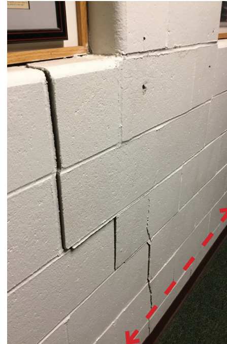
Fig 039. CMU Wall Shifted Out Of Plumb
