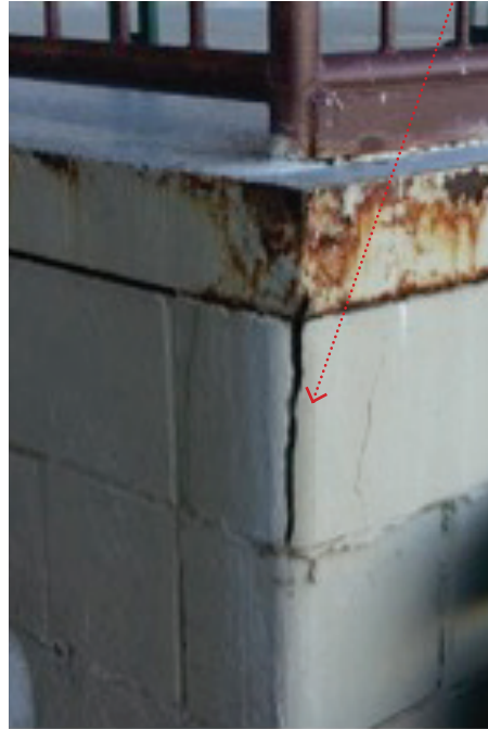
Fig. 047. Corrosion Due To Water Infiltration
