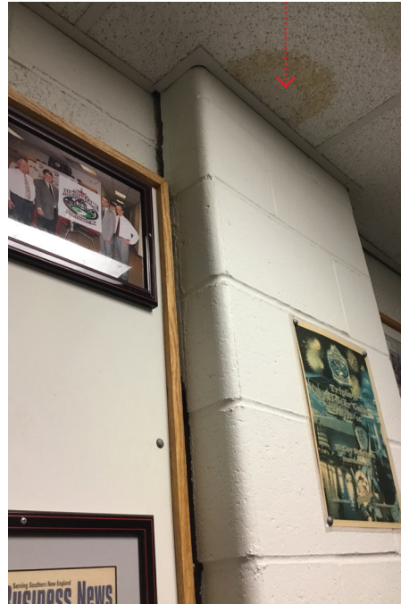
Fig 038. Example Of CMU Wall Movement
