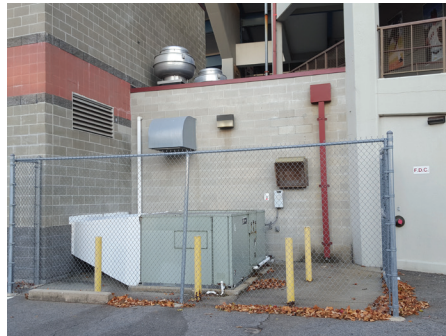
Fig. 068. HVAC Equipment Exposed @ Exterior
