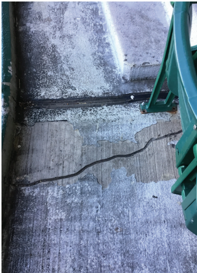
Fig. 104. Major Cracks In Horizontal Assembly
