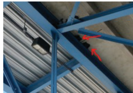
Fig. 050. Shims Involuntarily Moving
