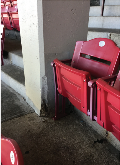
Fig 107. Major Chips & Cracks At Columns
