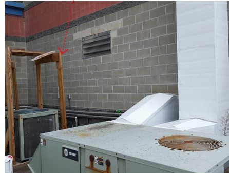
Fig. 070. Example Of At Grade HVAC Unit
