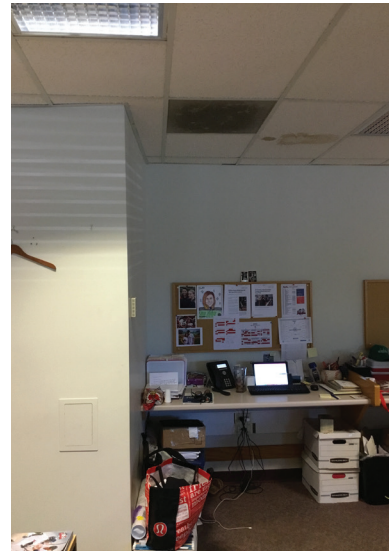
Fig. 128. Stained Ceiling Tile In Admin. Space
