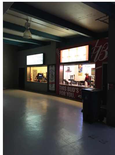
Fig. 150. Malfunctioning Concourse Lighting
