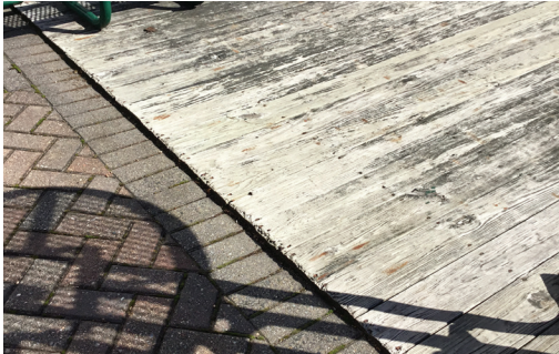
Fig 033. Uneven Pavement Exceeding 1/2"
