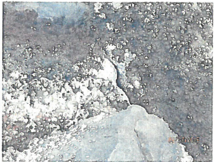
Fig. 22. Damage to west edge of impact boulder
