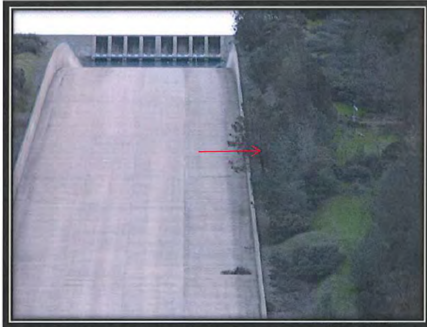
9. This view looking upstream along the FCO discharge chute shows one tree (arrow) that needs to be removed following a significant effort to remove brush along the outside of the wall.
