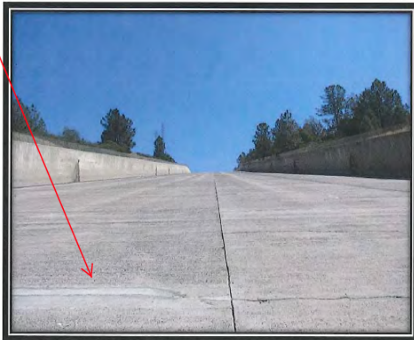
13. This view is looking upstream along the FCO channel from the dentates. Dark, vertical stains along the walls indicate the location of the drain outfalls.
