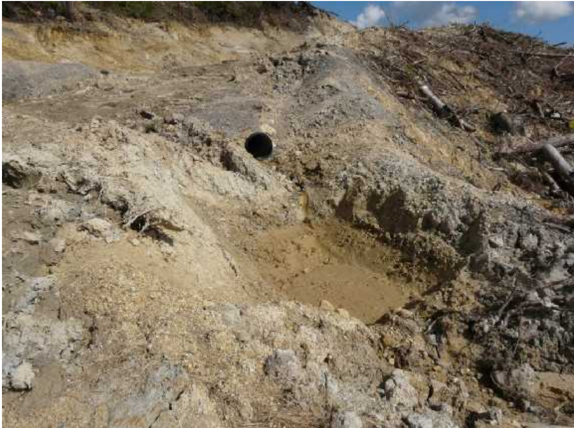
Figure 10: Example of a storm water control device in Ngunguru Forest. Shown here is a culvert pipe emptying into a sump located in an apparently unstable bank, indicating the need for continuous maintenance and monitoring for effectiveness. Photo Wade Doak.28/08/2011
