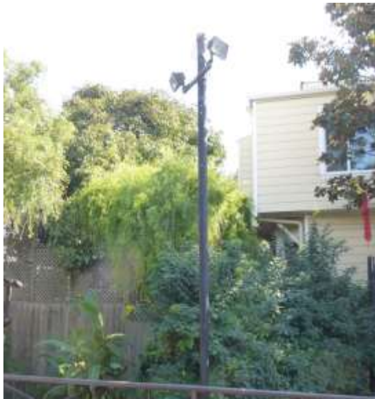
New Light Fixtures
