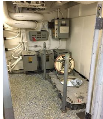
Figure 13 – Sample Berthing 2 Starboard Side Egress – Scuttle Down to Forward IC (no outlet)
