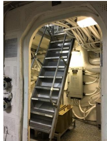
Figure 16 - Non-watertight door frame from Berthing 2 to the ladder going up to Berthing 1 Access Trunk. There is no hatch at the top of this ladder to prevent water from flooding up into Berthing 1.
