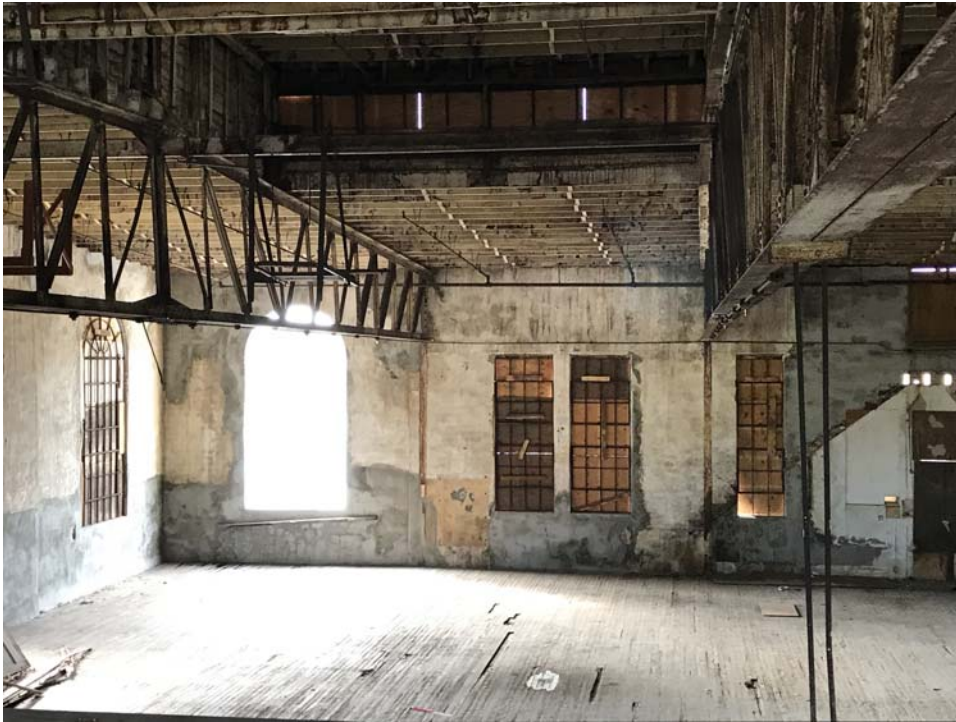
Figure 12: Sixth Truss from West End and dislodged window 09-25-2017
