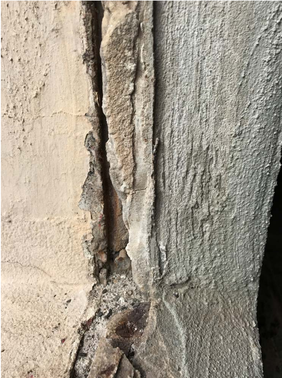
Figure 18: Sill and jamb of dislodged window
