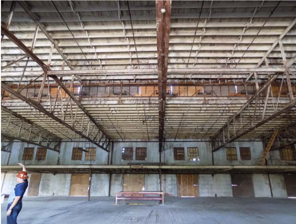
Figure 8: Second, Third, Fourth, Fifth and Sixth Roof Trusses from West End Looking North 07-25-2017
