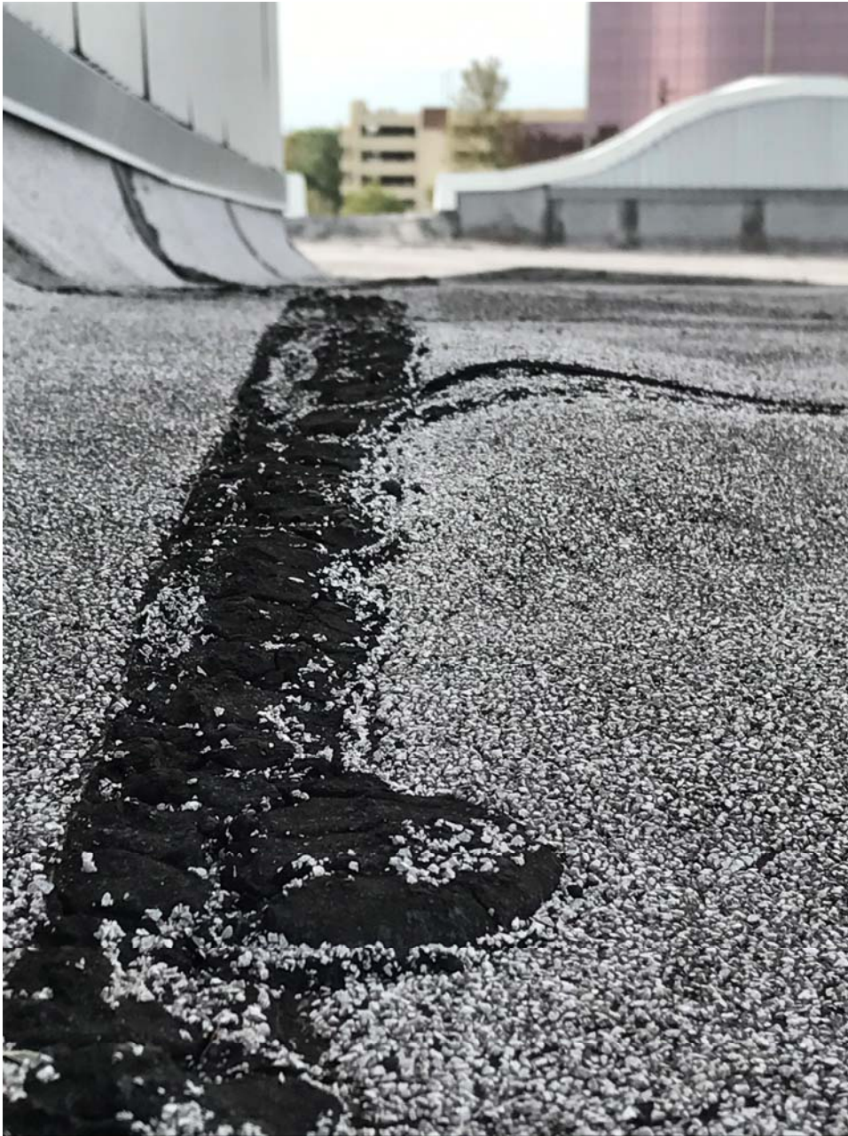
Figure 16: West end of Clearstory – roof system buckling 09-25-2017
