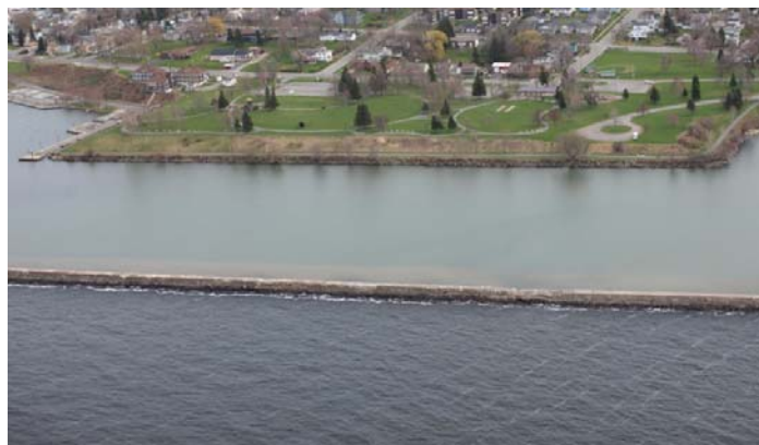
Figure 2-1 A reach of shoreline with primary revetment protection and secondary off-shore breakwater protection in Oswego (Oblique Imagery, USACE 2012)
