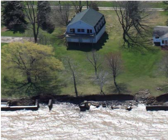
Poorly engineered. Will last 0-5 years.
