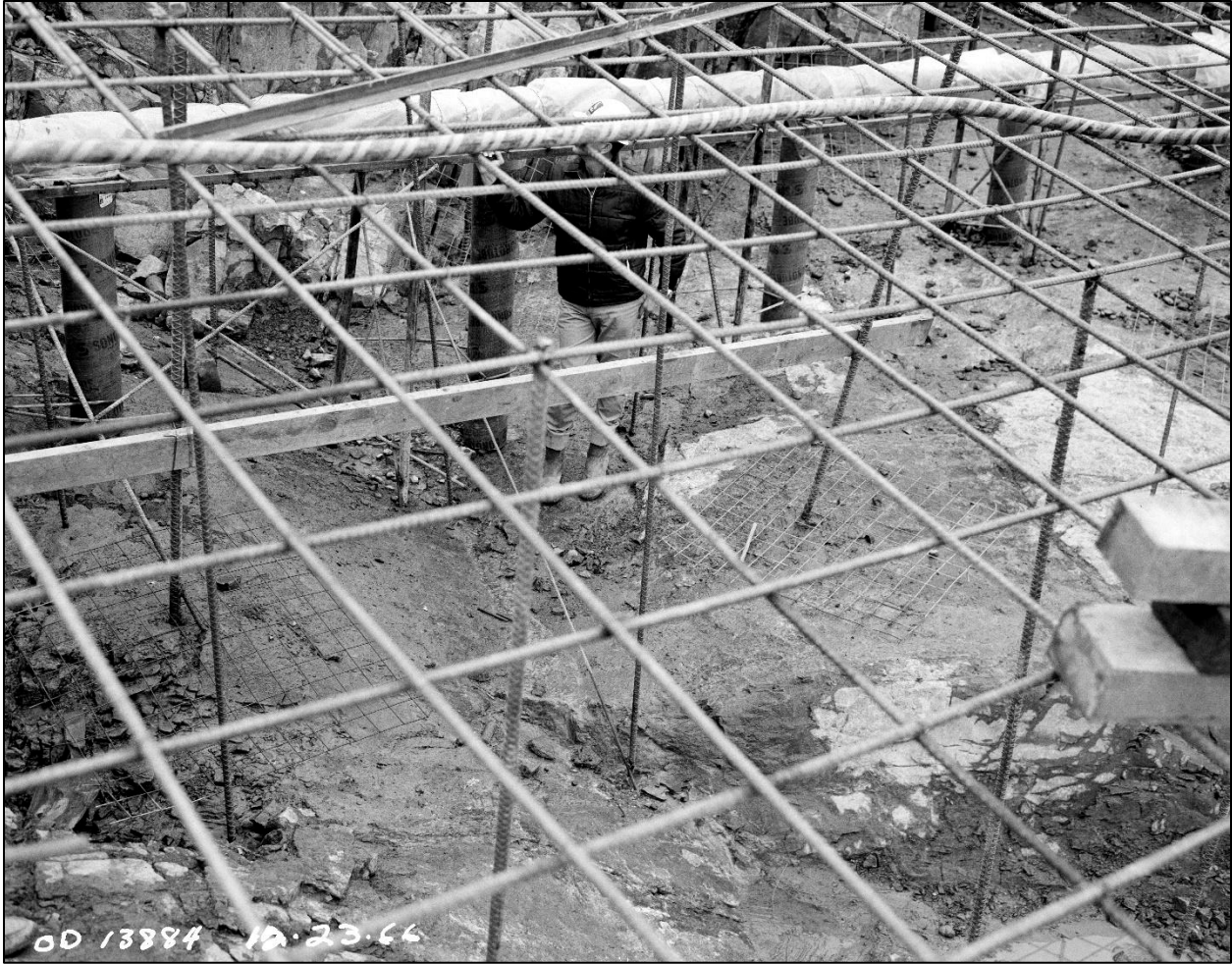
Figure A-26: Herringbone drains being constructed on top of gravel filled sonotubes. The drains appear to be wrapped in plastic. Based on the worker standing beneath the drain pipe, the drains were likely placed up to 6 feet above the foundation they were intended to drain.
