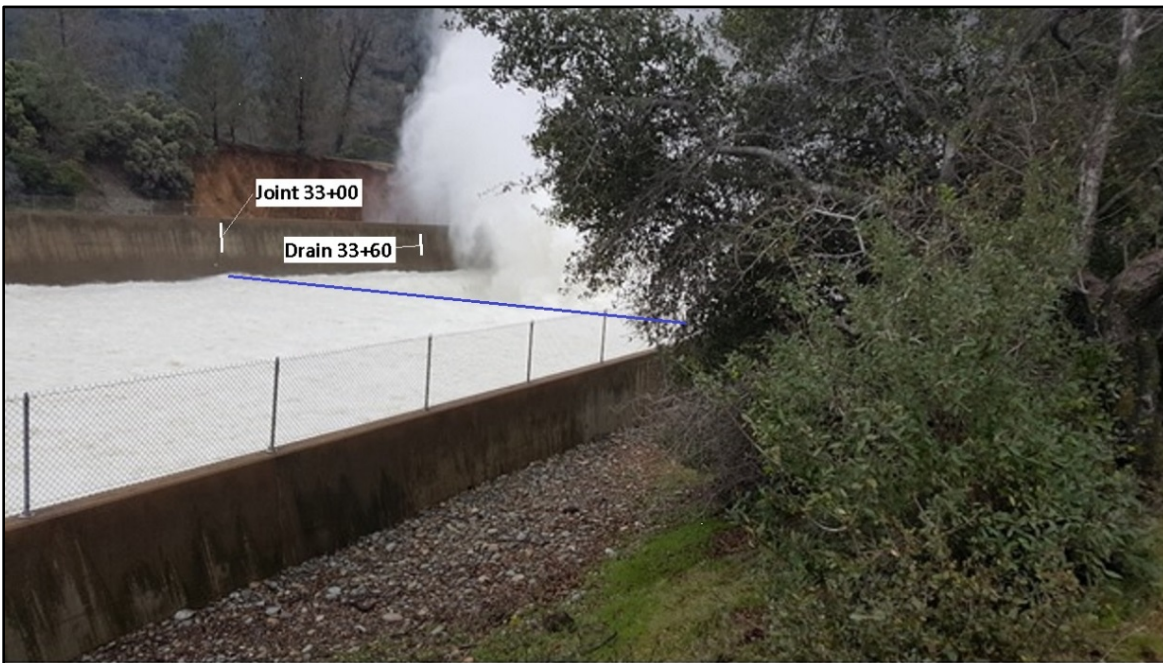
Figure 4-4: Flow in chute at 12:07 am (from DWR)
