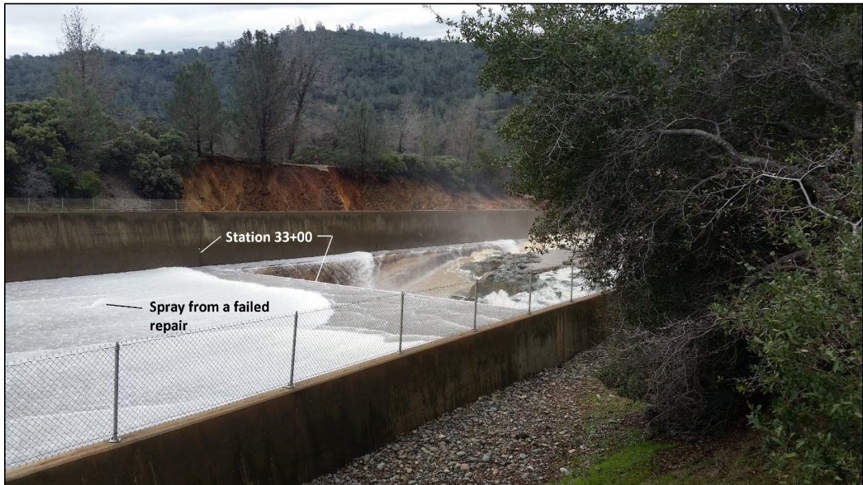
Figure I-9: Flow in Chute at 12:26 [I-2]
