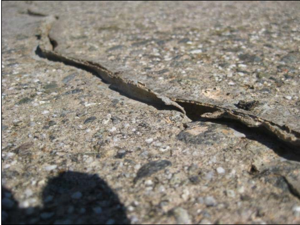
Figure G-5: Sealant Failure Over Herringbone Crack
