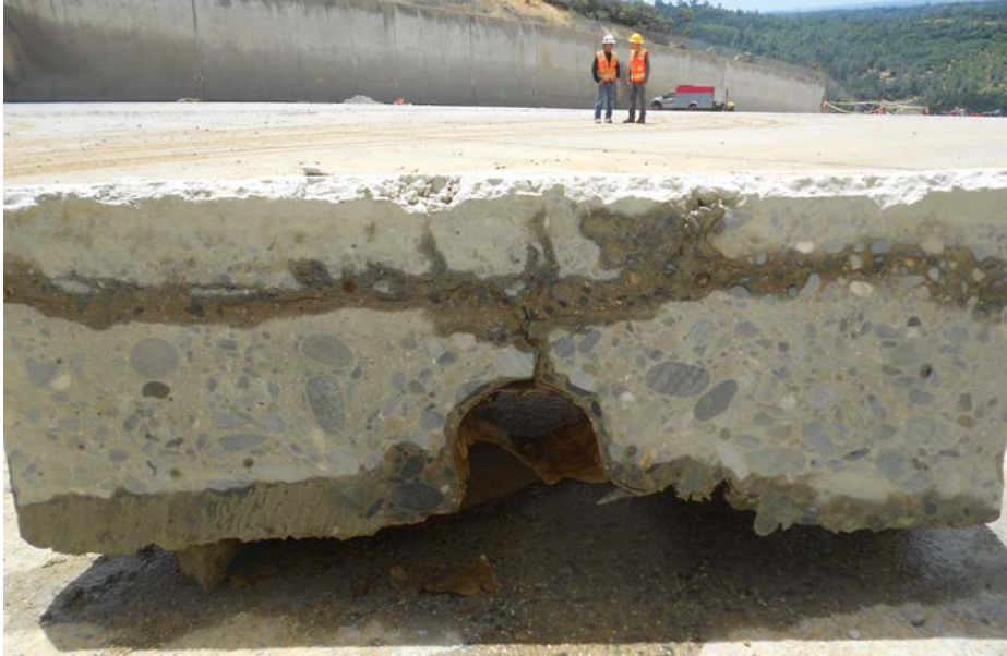
Figure D-26: Delamination Extending from Crack over Herringbone Drain Encountered in Forensic Trench 26F1 at Sta. 26+37
