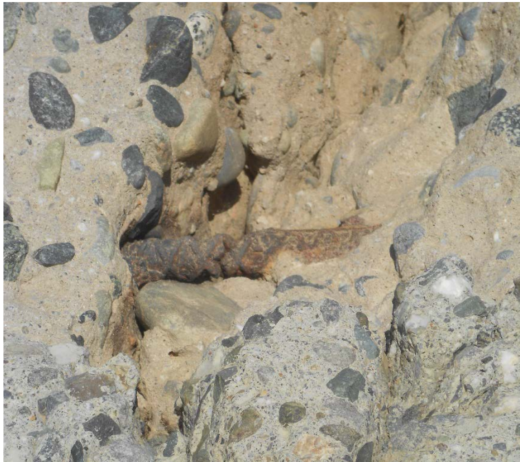
Figure D-16: Example of failed reinforcement steel with corrosion at a crack above a herringbone drain. The reinforcement is completely severed.
