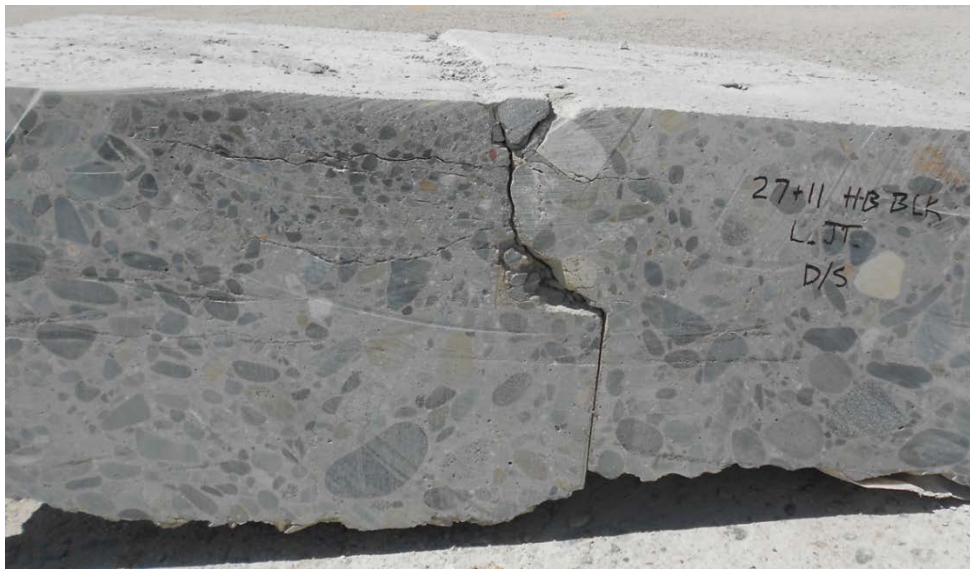
Figure D-27: Delamination Extending from Centerline Contraction Joint at Sta. 27+11
