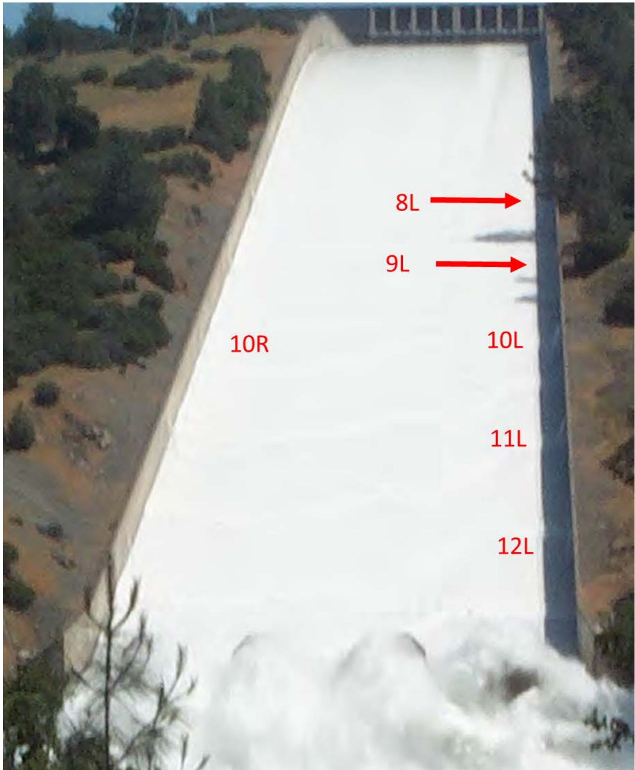
Figure F1-6: May 17, 2006 - Spillway in use (photo provided by DWR): obscured view, but possibly little to no flow in outfalls 9L and 8L and possibly 10R.
