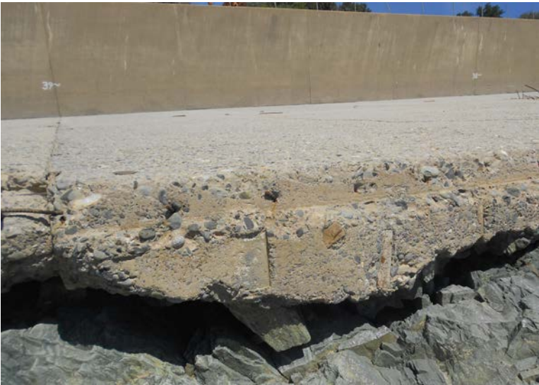
Figure D-21: Lateral Contraction Joint at Sta. 39+00 on Left Side of Photograph with Missing Joint Key
