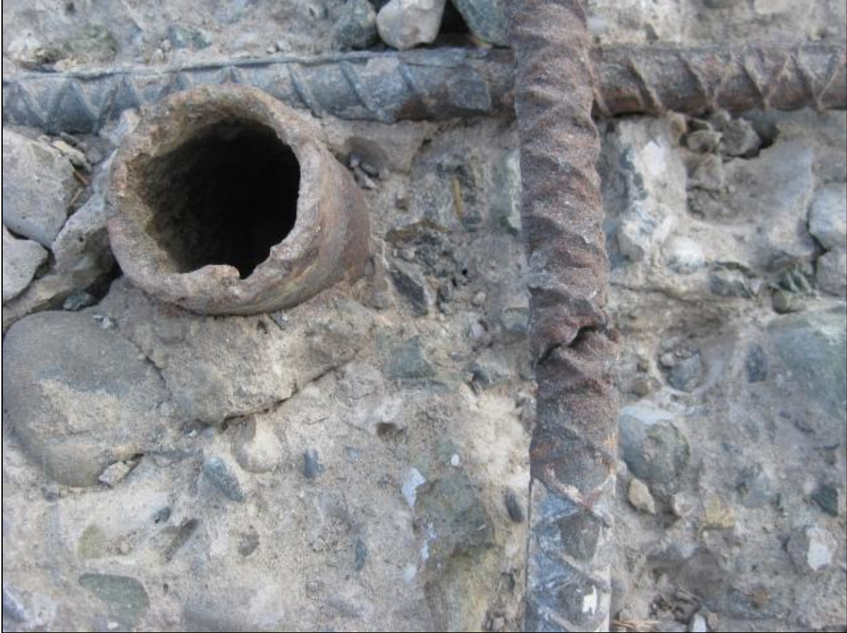
Figure A-30: Broken rebar at location of a crack above a herringbone drain. Note that the pipe shown in this photograph was used to support the wooden form for the gravel that encapsulates the drain pipe. (Photo taken during the 2009 repairs)
