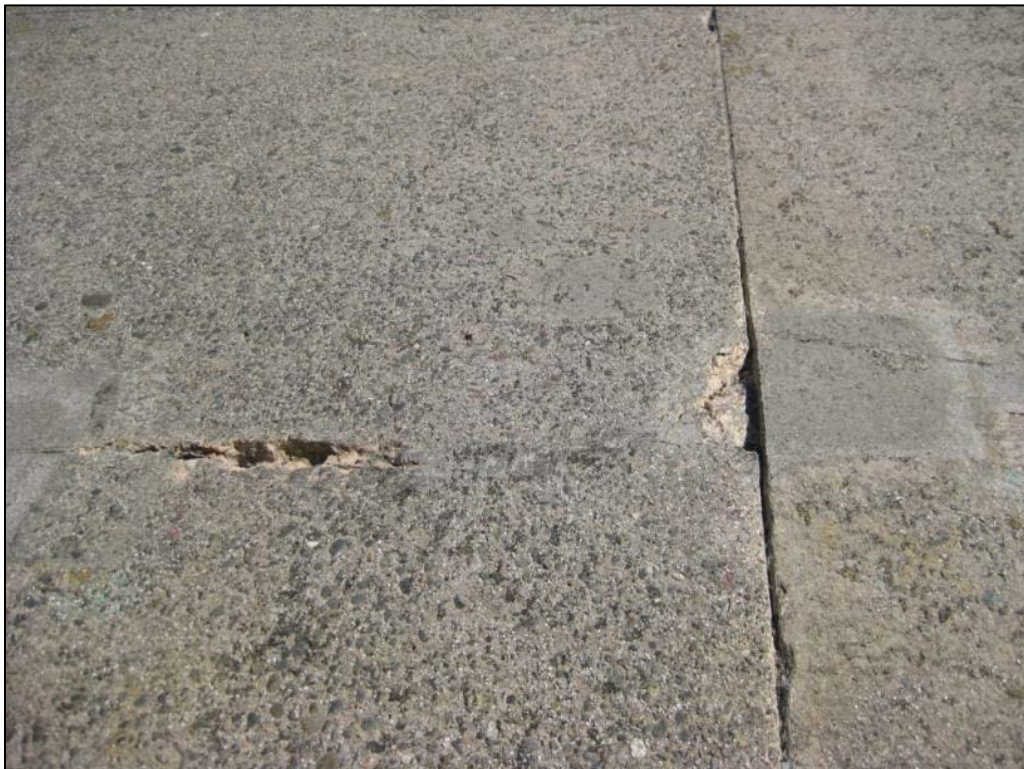
Figure G-6: New Concrete Deterioration
