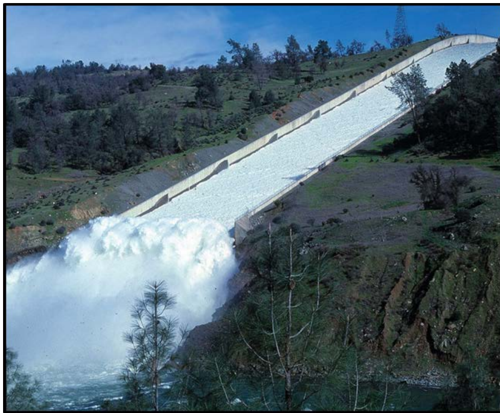
Figure F1-5: February 3, 2006 (Photo provided by DWR): Spillway in use - all right side drains apparently flowing well. No photos available for left side.
