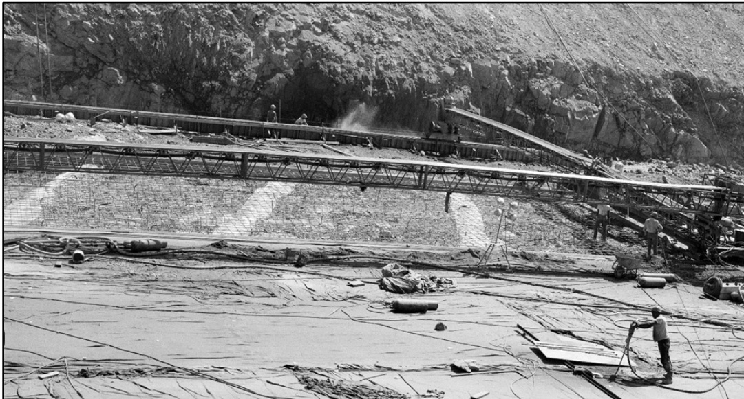
Figure 3-6: Plastic sheets covering herringbone drains before concrete slab placement – Photo dated 09/30/66 (Photo OD_13202_09_30_1966) [8]
