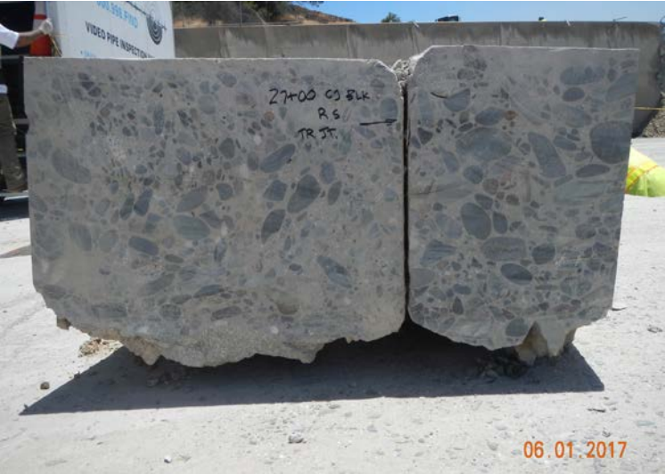
Figure D-20: Lateral Contraction Joint at Sta. 27+00; Joint Key Absent
