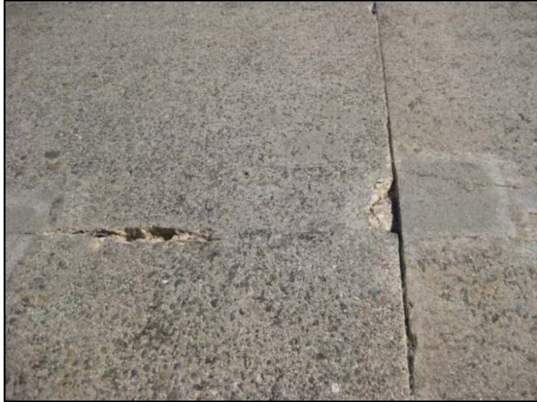
Figure 3-13: Concrete spall before repair [11]
