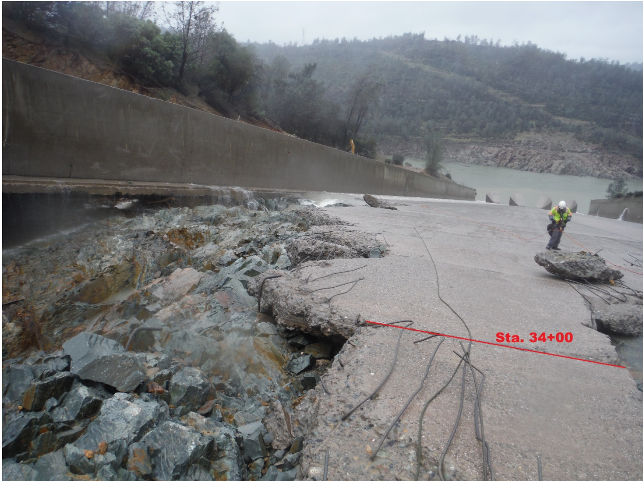
Figure I-10: Initial Damage Area Looking Downstream Showing Bent Bars Upstream of Sta. 34+00
