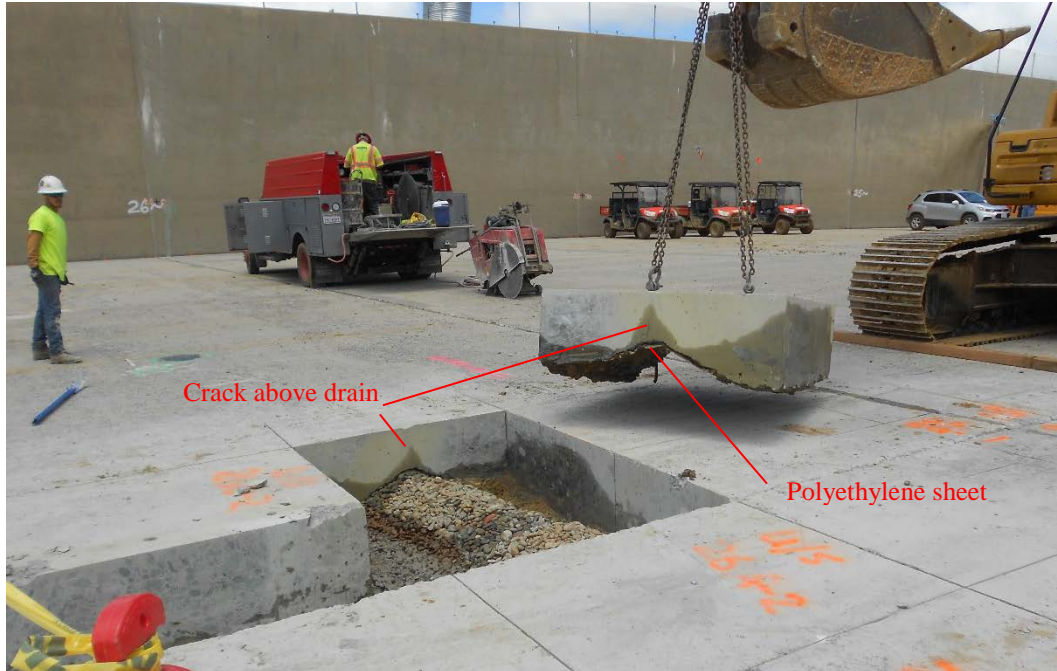
Figure D-34: Removal of Saw-cut Slab from Above Herringbone Drain in Upper Chute Area
