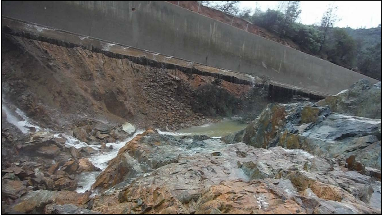
Figure A-28: Damaged area downstream from Sta. 33+00. Note the concrete wall base thickness varies. Also note the unevenness of the broken rock in the foreground.
