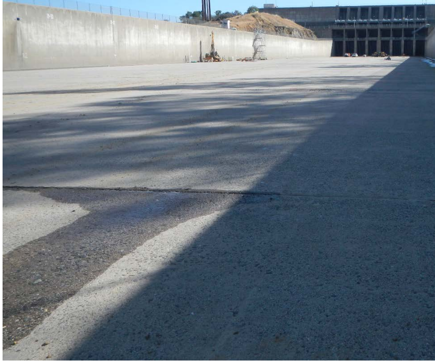
Figure D-10: Water Discharging from Lateral Contraction Joint at Sta 23+00
