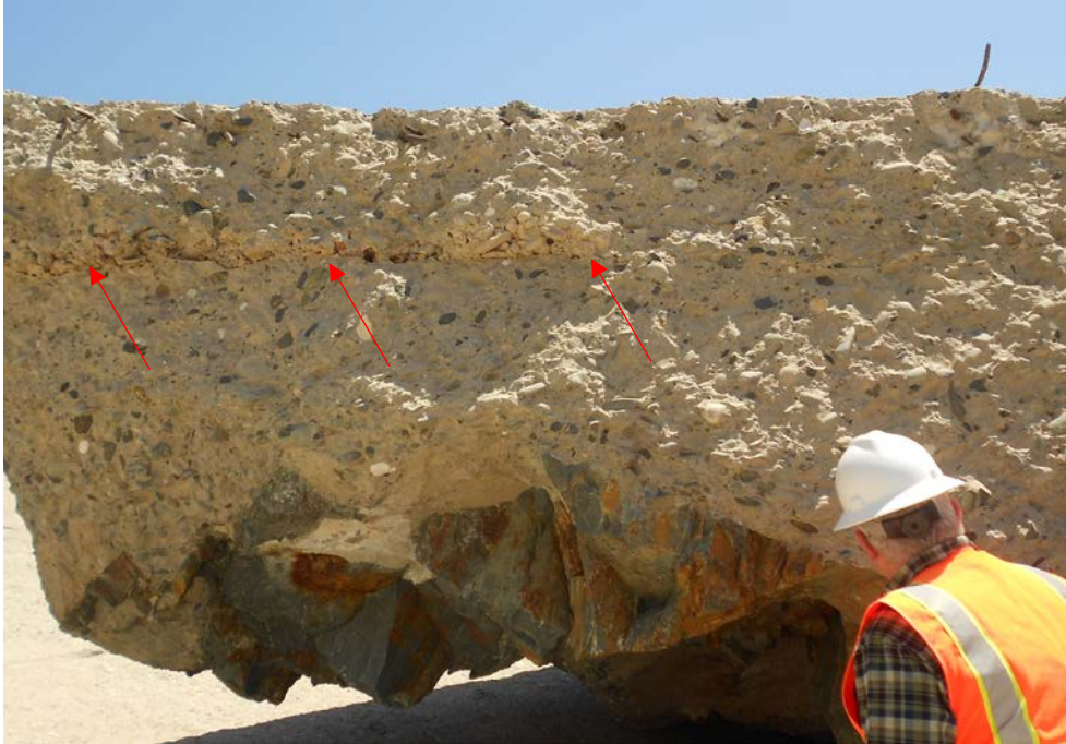
Figure D-15: Example of poorly prepared joint (red arrows) between two concrete placements in loose block lodged at dentates; joint was associated with open honeycombing, about 2 feet below top of slab; maximum slab thickness was ~6.2 feet. Note base of concrete bonded to relatively fresh rock, which became detached when the slab was lifted from foundation.
