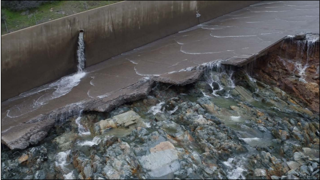
Figure I-29: Right Side of Failure Area Looking Upstream – Captured from Drone Video [I-2]
