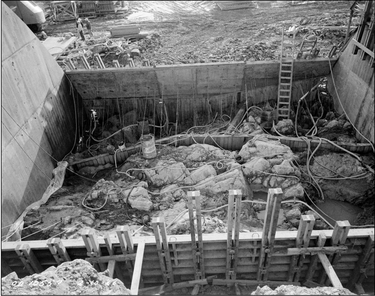
Figure A-15: Clean-up effort for the emergency spillway gravity crest structure just prior to placement. Note that all mud, debris, and loose or unsound rock fragments have been removed and the rock has been pressure washed. (Photo OD_10557_03_10_1966)
