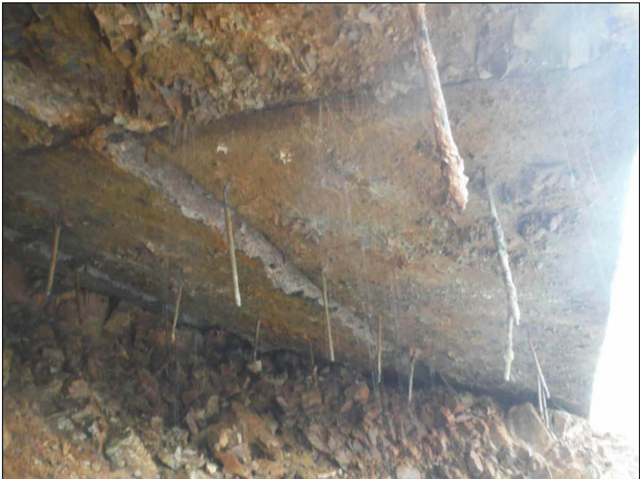
Figure A-19: Anchor bars on the underside of the slab upstream of Sta. 33+00 (on right edge). Note the smooth underside of the chute slab that was to have been placed on a rock foundation which would have been expected to be irregular. (Photo DSCF9788)
