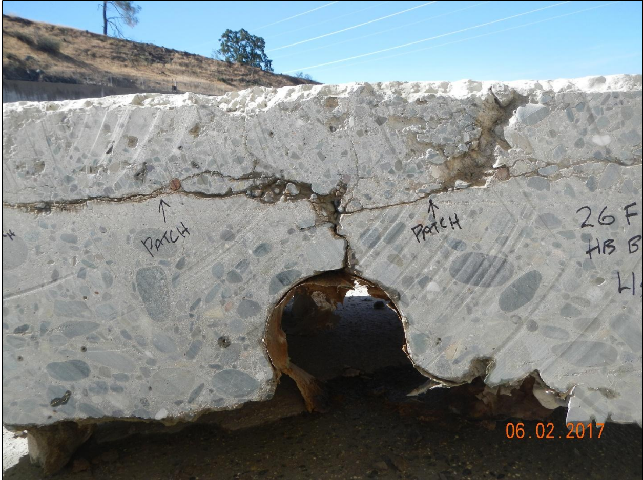
Figure A-29: Excavated section of concrete at herringbone drain location. Note the cracking associated with the drain and the delamination of concrete at the reinforcement layer. (IFT Photo taken during forensic investigation of the chute)
