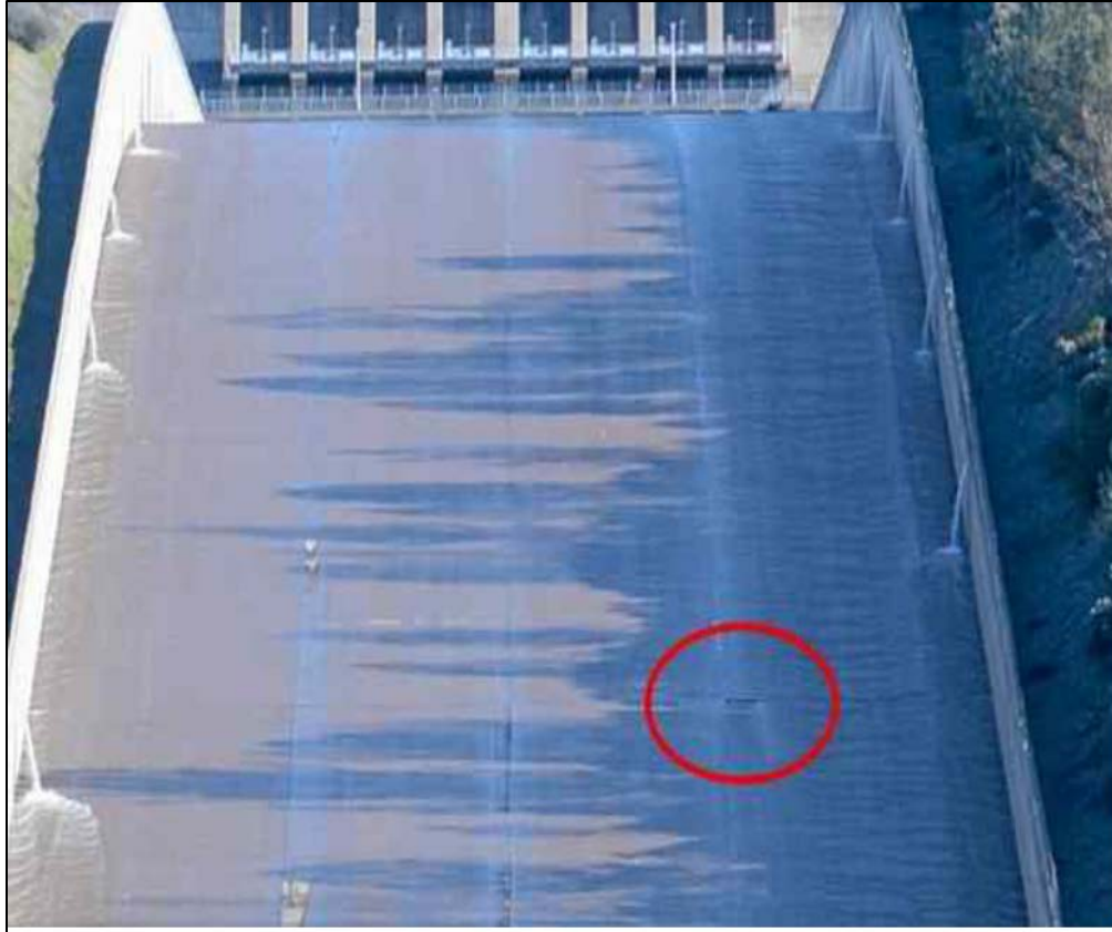
Figure I-16: Spall in Lane 5 Jan 27, 2017 [I-6]
