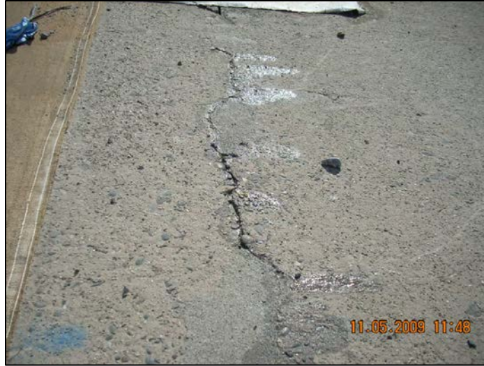
Figure B-10: Crack over Herringbone Drain at Oroville Dam Service Spillway, IFT Photo
