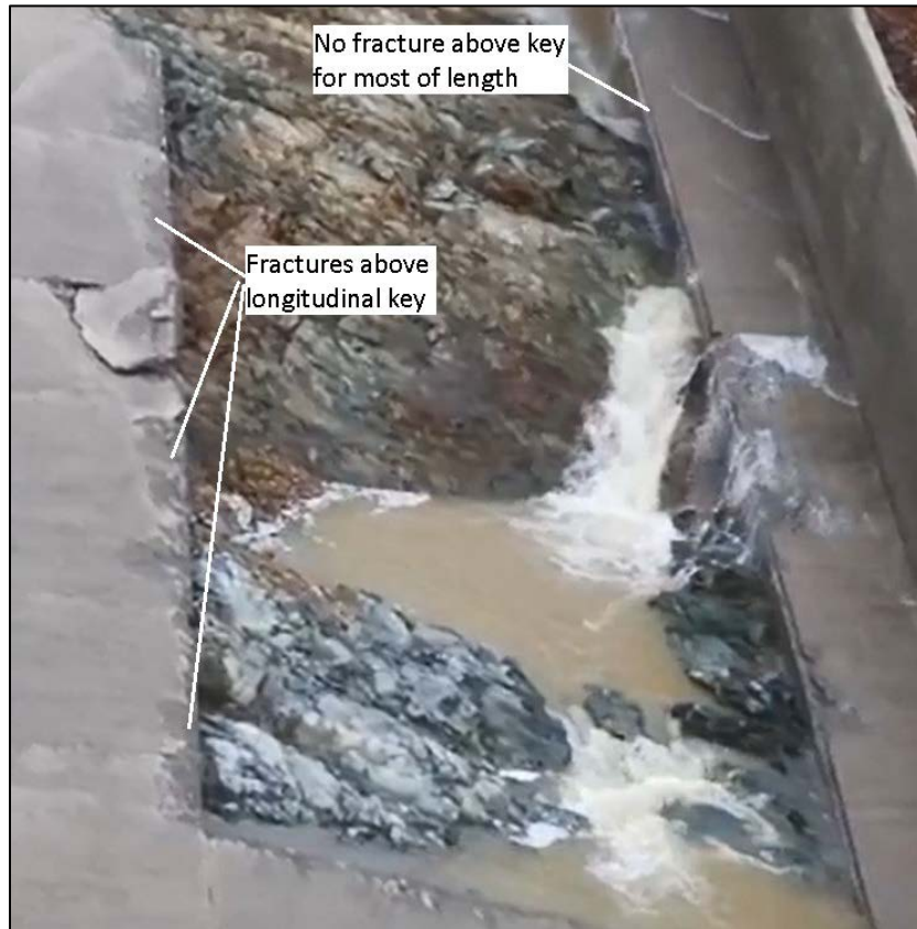
Figure I-28: Detail of Damage Downstream of Station 34+50 [I-2]
