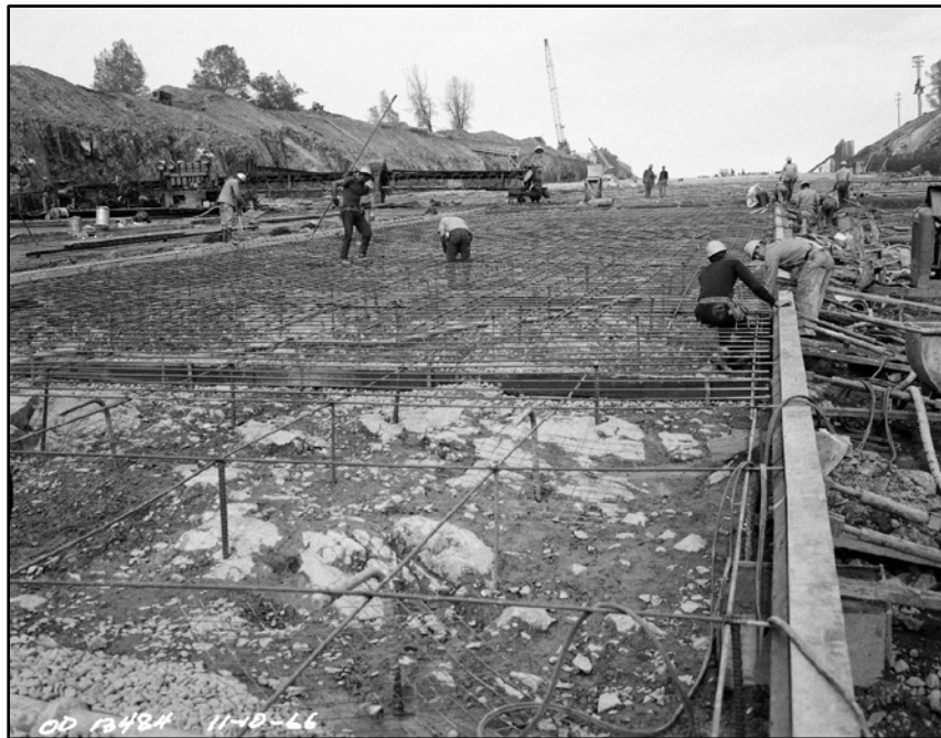
Figure 3-10: Example of the clean-up effort for the spillway chute prior to placement.
