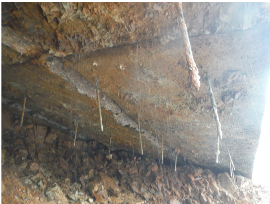
Figure D-29: Undercut Area of Chute Slab at Sta. 33+00 (left side) with Exposure of Anchor Bars
