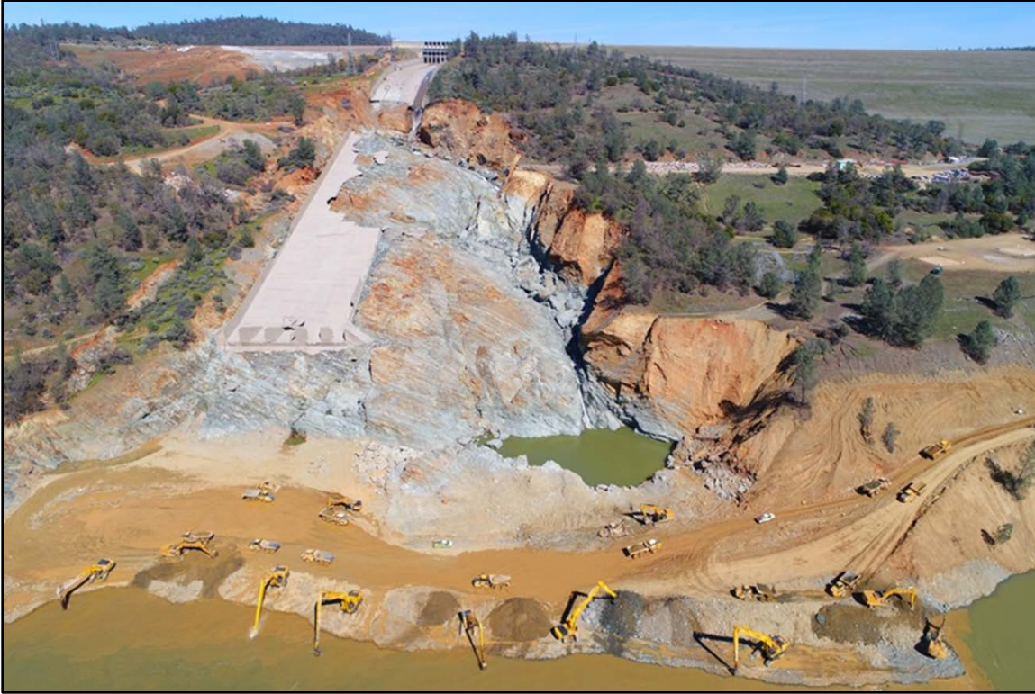
Figure 3-20: Ultimate damage at the service spillway (from DWR)
