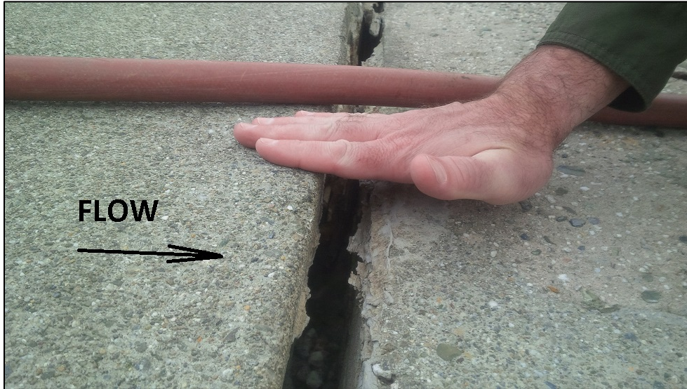
Figure I-23: Gap in Invert Slabs at Station 29+00 [I-2]
