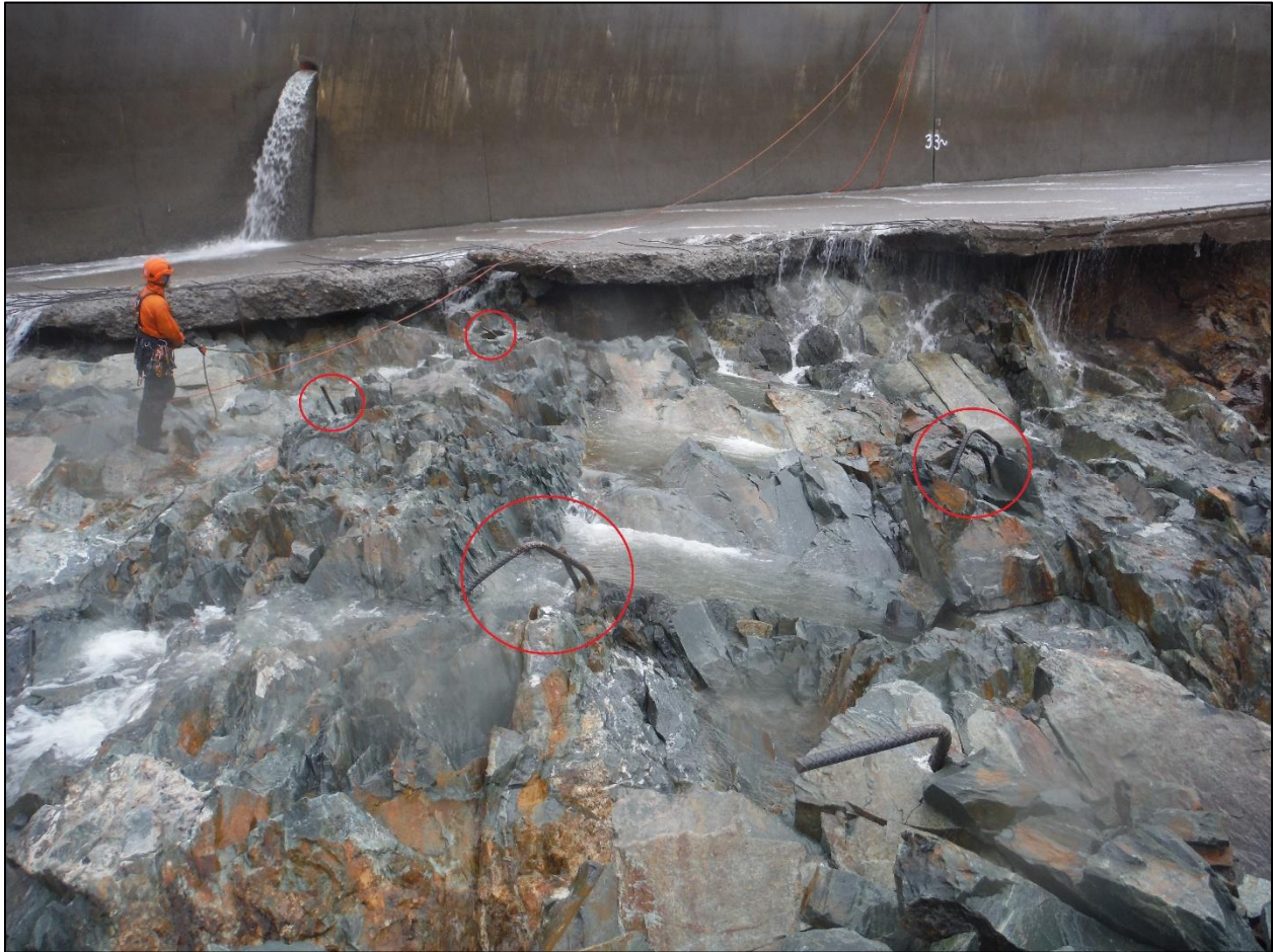
Figure A-20: Damage in Lane 3 downstream from Sta. 33+00. Cut anchor bars are circled. These were replaced because they were tilted. Replacement anchor bars can be seen in two locations. Note the drain discharging from the wall at approximate Sta. 33+60. (Photo DSCF5904r)
