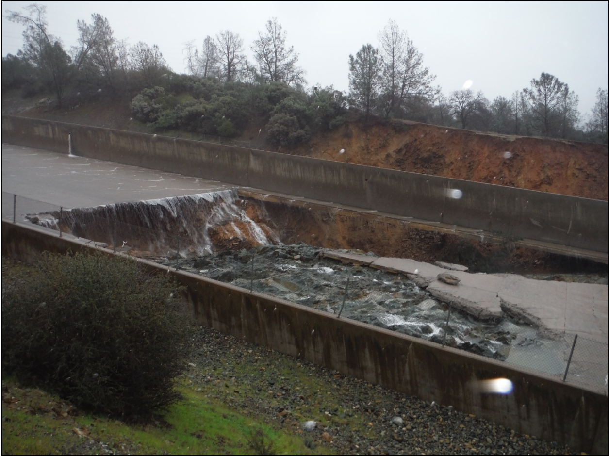
Figure A-27: Damaged area downstream from Sta. 33+00. Note the concrete slab thickness varies in the center of the chute (as discussed in Appendix D).
