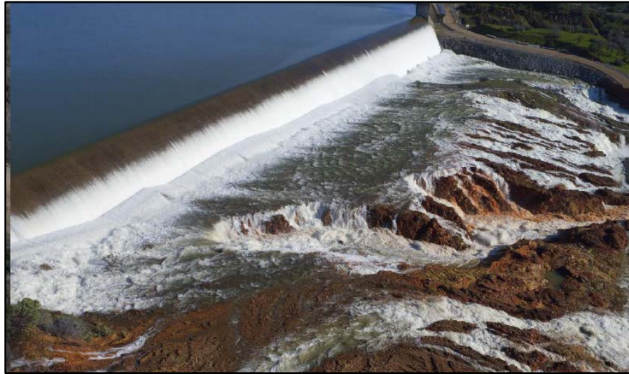
Figure 4-10: Emergency spillway headcutting on February 12 (from DWR)
