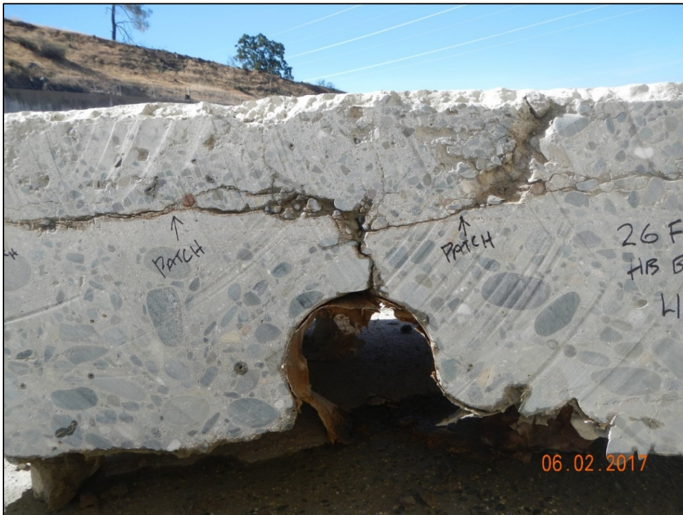
Figure 25: Delamination of Slab (IFT photo)
