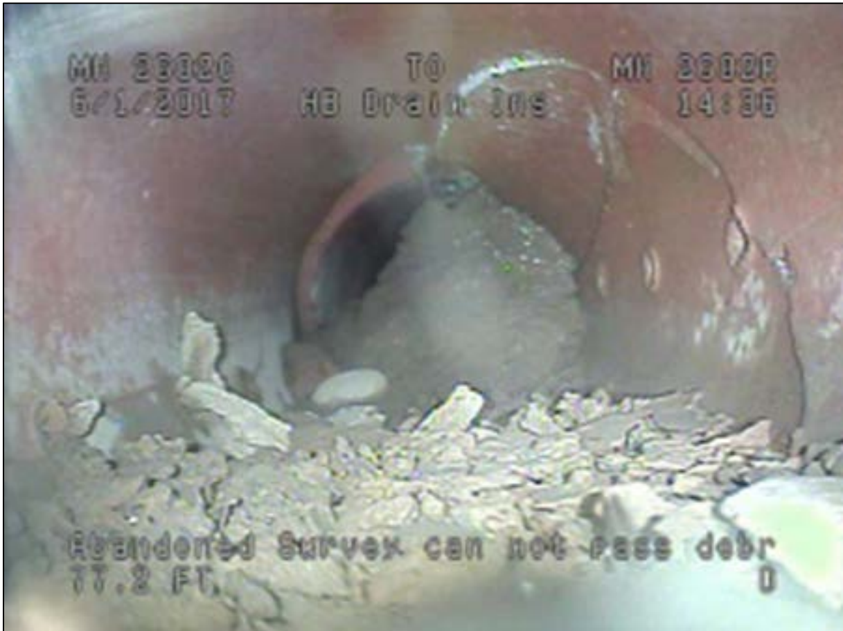
Figure A-23: Herringbone drain inspection image. Note the drain has been cracked. (from HDR investigation [A-6])
