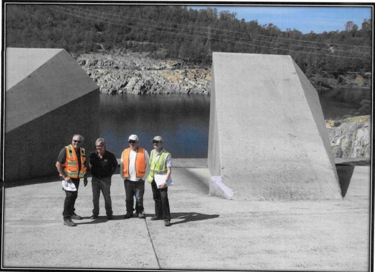
Figure B-8: Observation of Cavitation Damage to Dentates, Reference [B-7]
