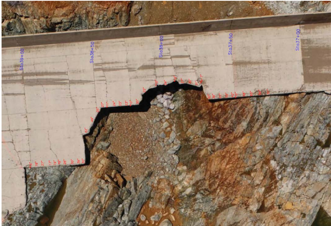
Figure D-13: Plan of Erosional Feature Between Sta. 37+00 and Sta. 39+00 Showing Observed Concrete Thickness Values (in inches)
