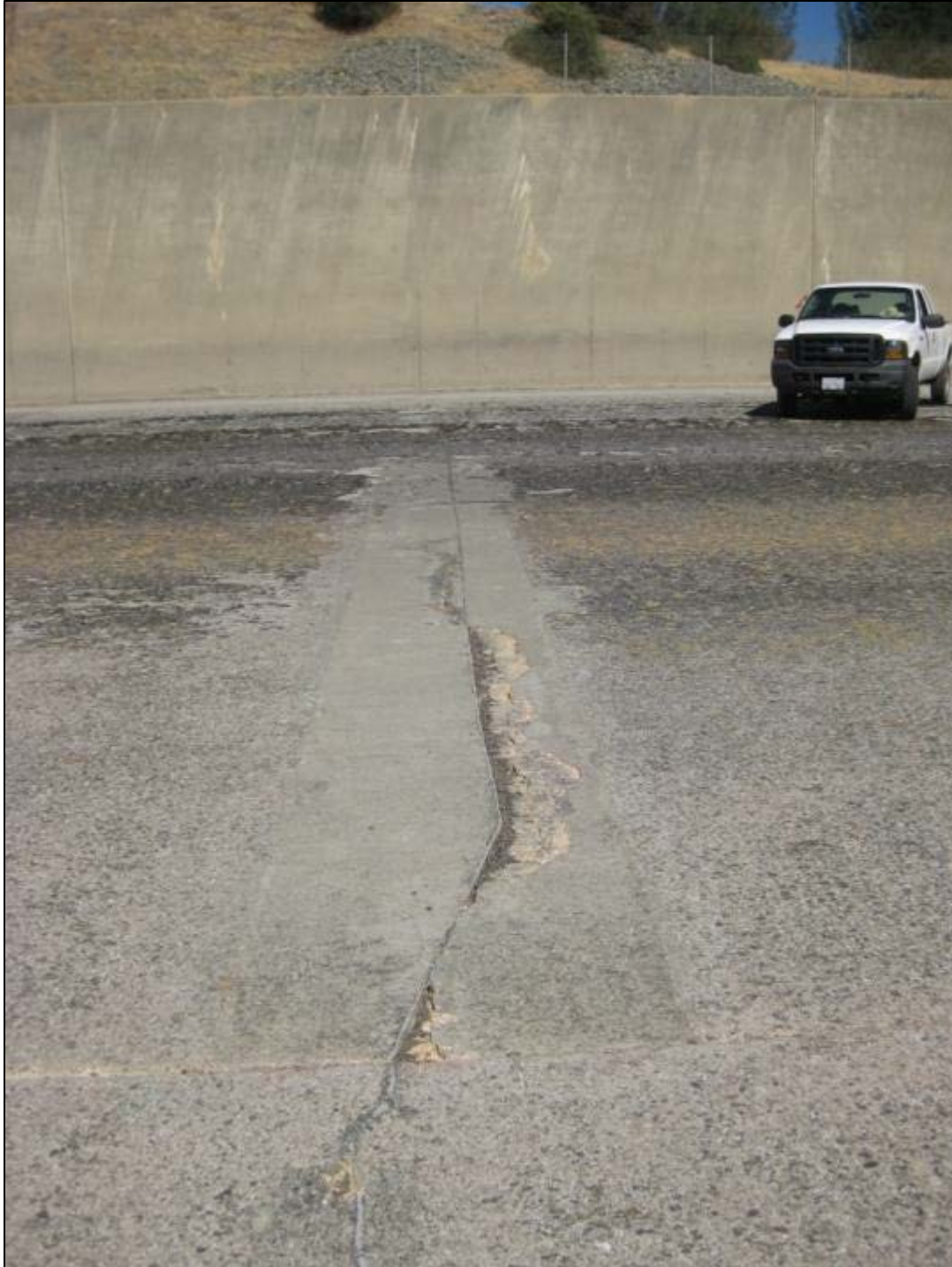
Figure G-7: Spalled Concrete in Previous Repair
