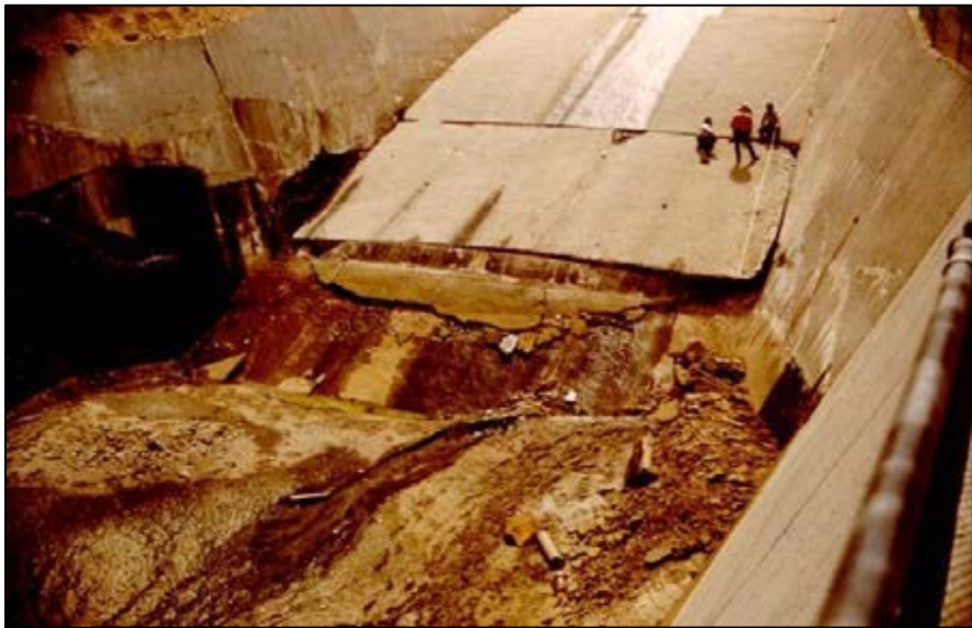
Figure B-9: Damage from Uplift of Chute Slab, USBR Report DSO-07-07
