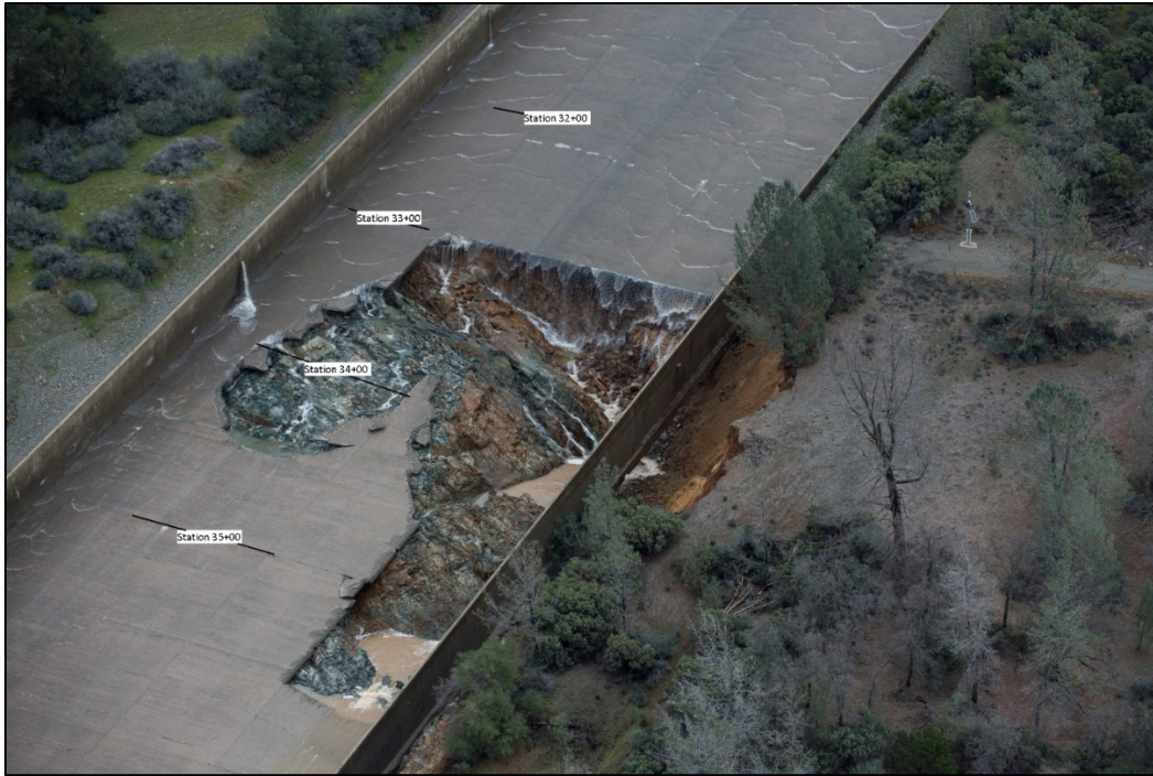
Figure I-27: Detail of Initial Spillway Damage [I-2]
