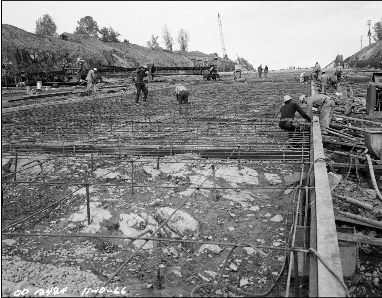
Figure A-17: Another example of the clean-up effort for the spillway chute prior to placement. Note what appears to be “compacted clayey fines” between the rock outcrops. (Photo OD_13484_11_10_1966)
