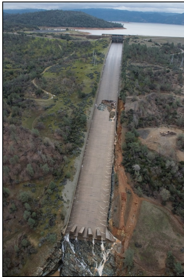
Figure 3-19: Service spillway chute damage observed after gates were closed on February 7 (from DWR)
