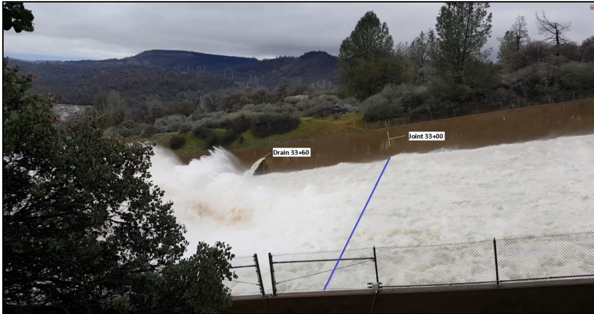
Figure 4-3: Flow in the chute at 10:32 am (from DWR)
