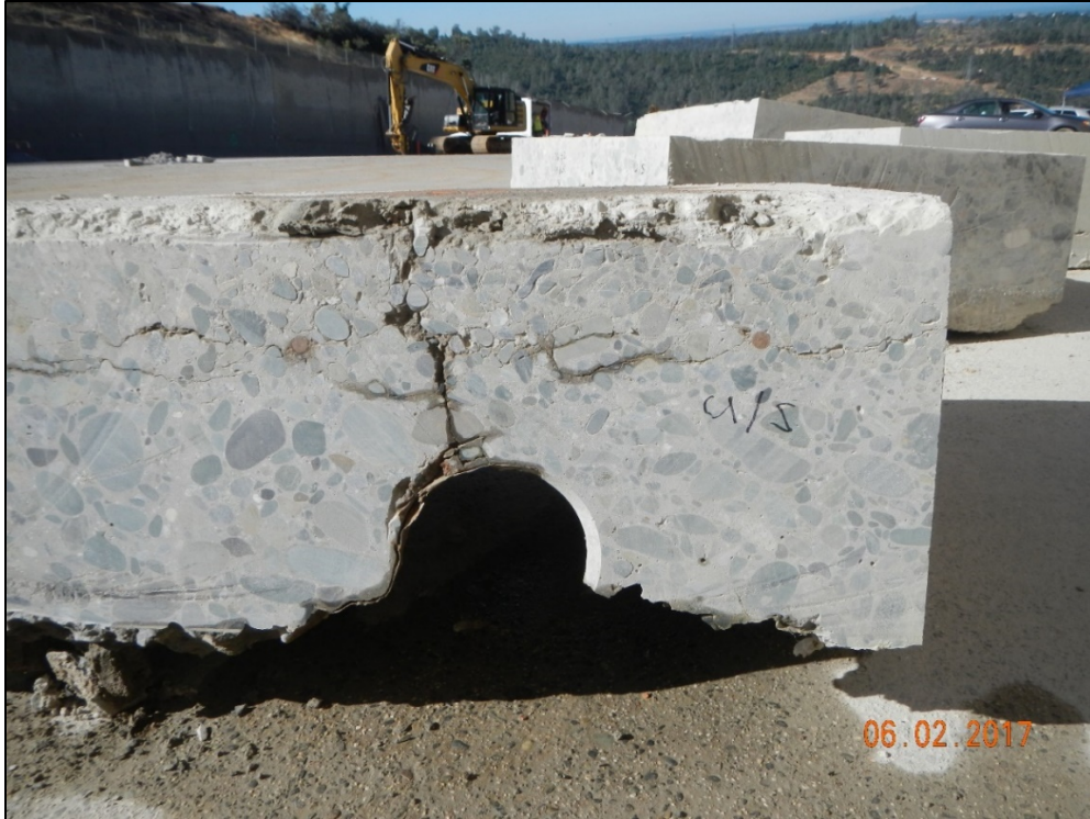
Figure I-24: Delamination of Slab (IFT photo)
