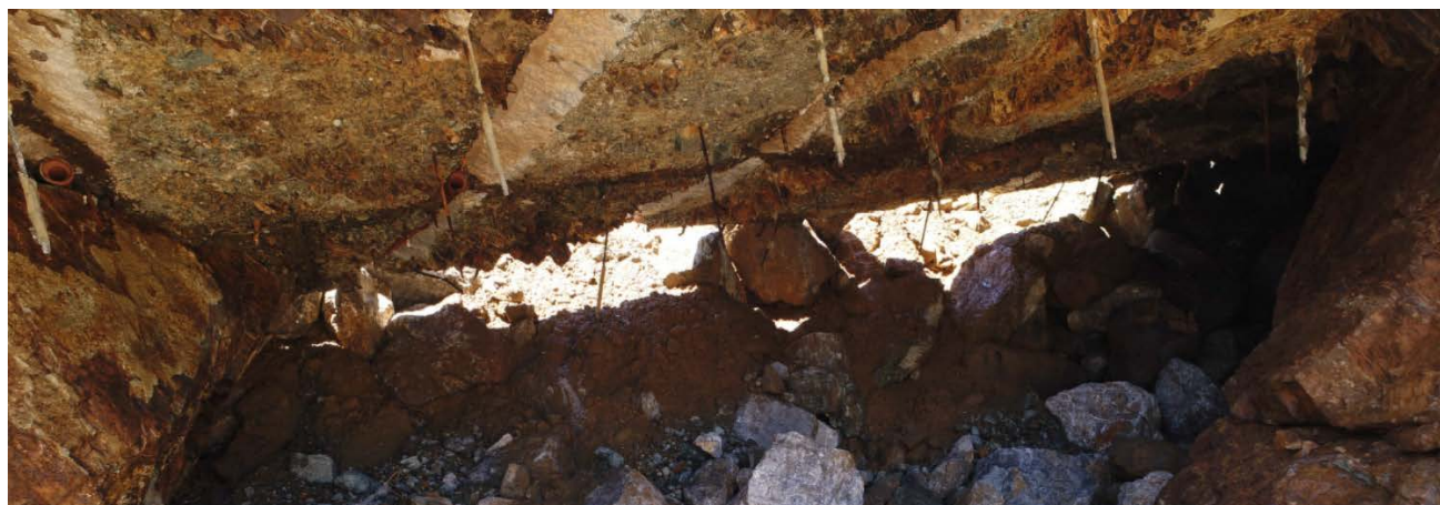
Figure D-30: Undercut Area of Chute Slab at Approximate Sta. 37+00 (left) to Sta. 38+00 (right)
