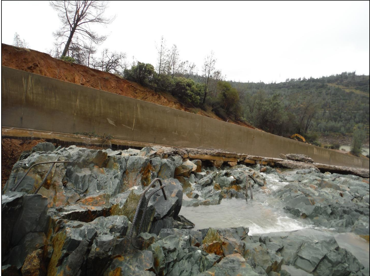
Figure A-22: Lane 3 downstream from Sta. 33+00 showing 3 sets of double anchor bars where one of the pair has been cut off. From this photo, it appears the bars at this location may have been adequately embedded in rock. (Photo DSCF5859)
