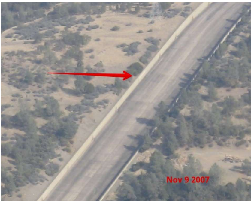
17 18 19 20 21 22 23 24 25 26 27 Non-functioning Sidewall drain revealed in a Nov. 9, 2007 spillway photograph 28 Source: CCRM Root Causes Report
