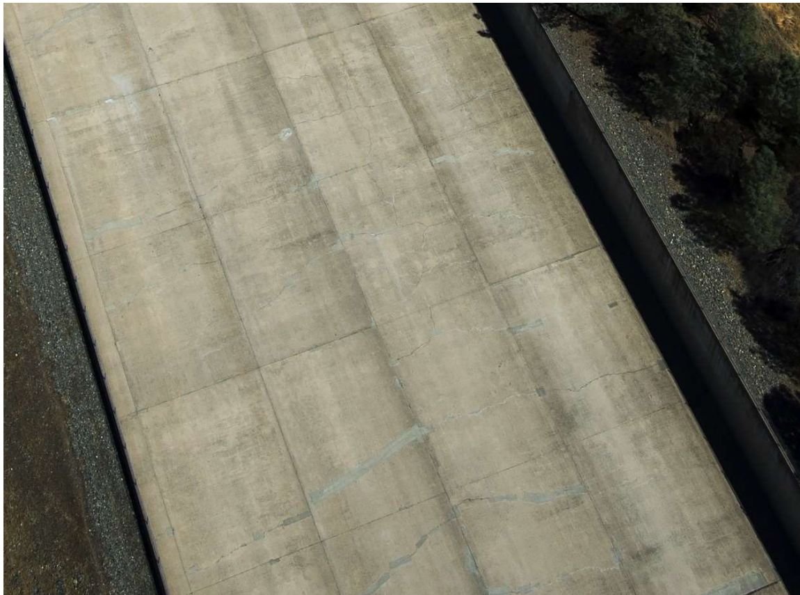
14 15 16 17 18 19 20 21 22 23 24 25 26 27 Photo of Cracks on Main Spillway 28 Source: UC Berkeley Center for Catastrophic Risk Management
