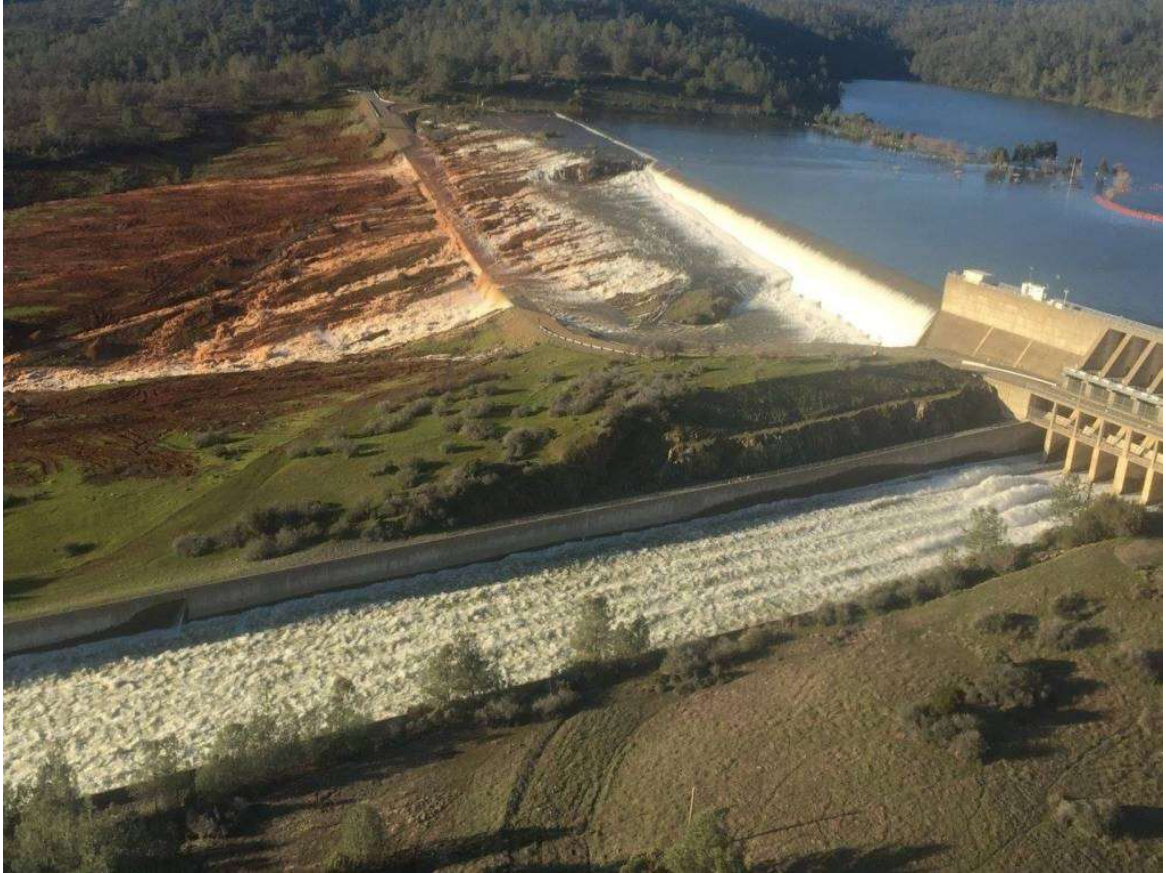
7 8 9 10 11 12 13 14 15 16 17 18 19 20 21 Main and auxiliary spillway at Oroville Dam on February 11, 2017 at 3 p.m. Source: William Croyle/California Department of Water Resources
