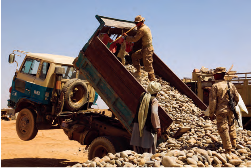
Marines unloading rocks at construction site in Helmand Province, 2009. Much of Afghanistan's current mineral production consists of sand, gravel, and construction stone. (USMC photo by Lance Corporal James Purschwitz)
