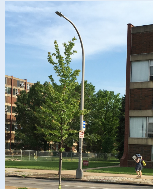
Existing Light Fixture
