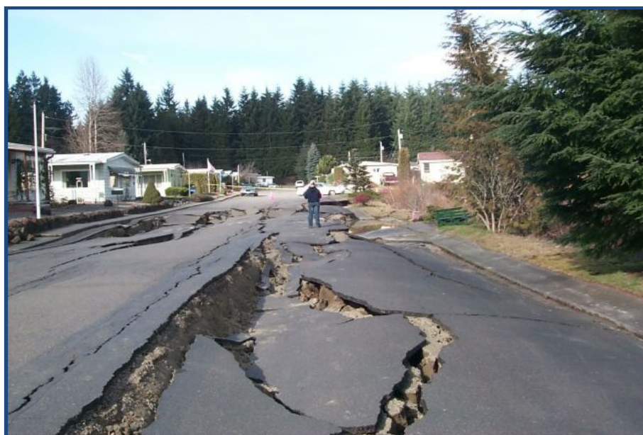
Figure 1-4. Damaged road due to liquefaction-induced lateral spreading, 2001 Nisqually, Washington earthquake. Photographic credit: DOGAMI Archives.
