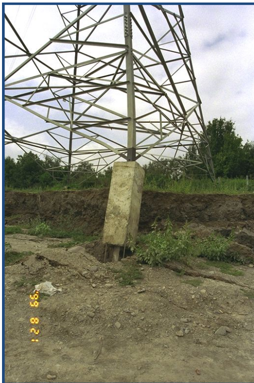
Figure 1-3. Example of ground failure underneath a transmission tower, 1999 İzmit earthquake (Turkey). Photographic credit: University of California, Irvine Consortium of University for Research in Earthquake Engineering Archives.
