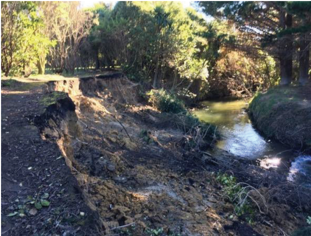
Figure 32: Bank erosion right bank upstream of Ngongotahā Road
