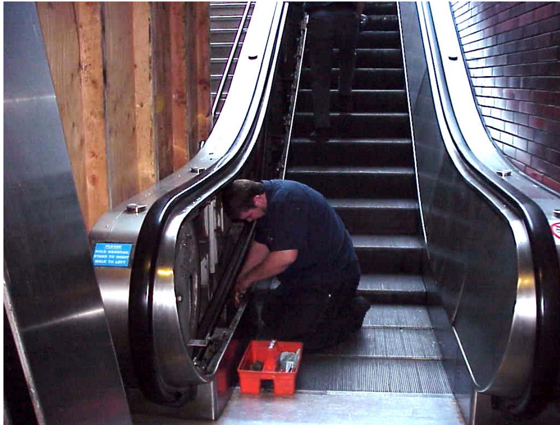
Escalators out of service
