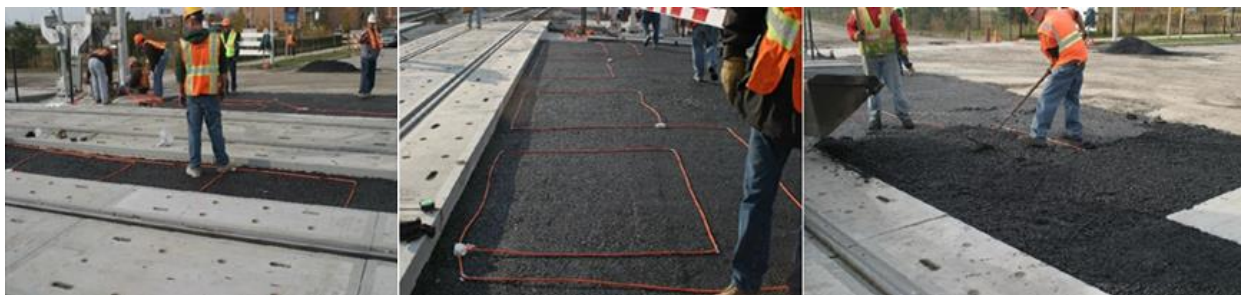
Figure 4-6: Vehicle Presence Detection Installation Sensors
