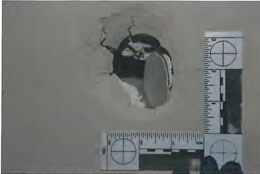
Figure 34 -- CSI photograph showing damage to the wall where Salena M. said Clark threw her head. Long, brown strands of hair are visible in and around the hole.
