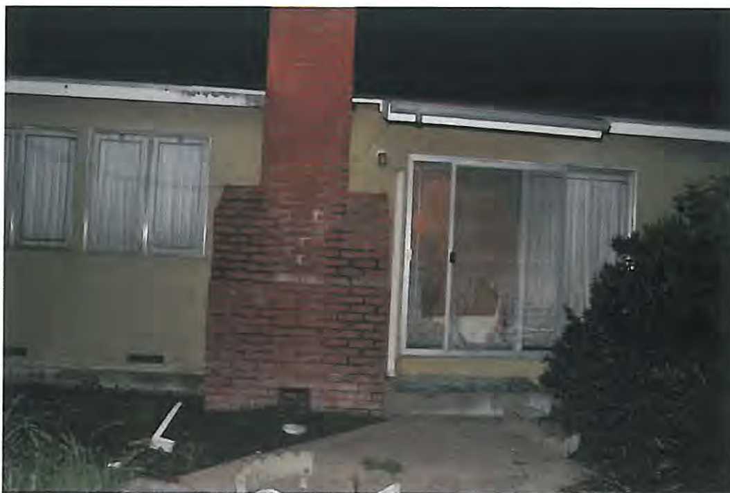
Figure 17 -- CSI photograph of Bill W.'s broken rear sliding glass door at 7570 29th Street with cinder block on ground. A gutter pipe is also visible on the ground. The broken sliding glass door had been covered with cardboard at the time this photo was taken.
