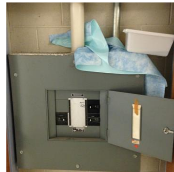
Frequent leaks threaten the electrical system at the current laboratory.
