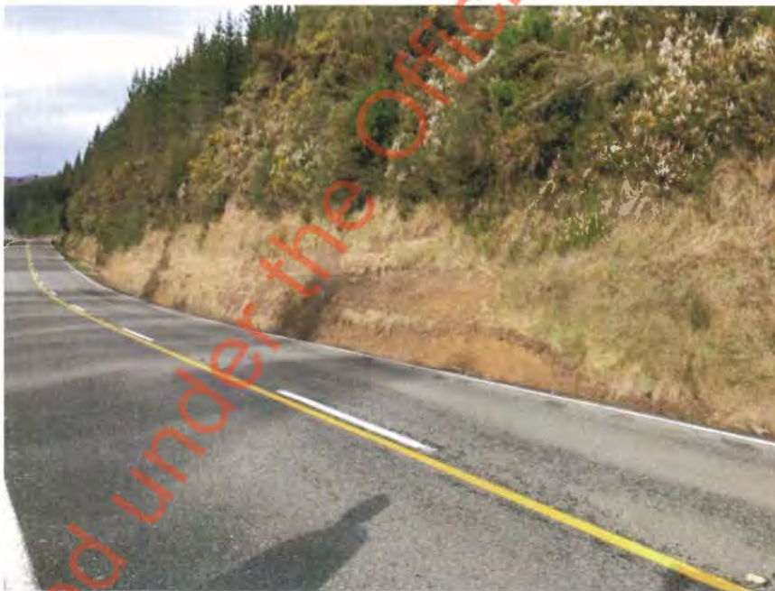
Figure 26 Embankment collision marks
