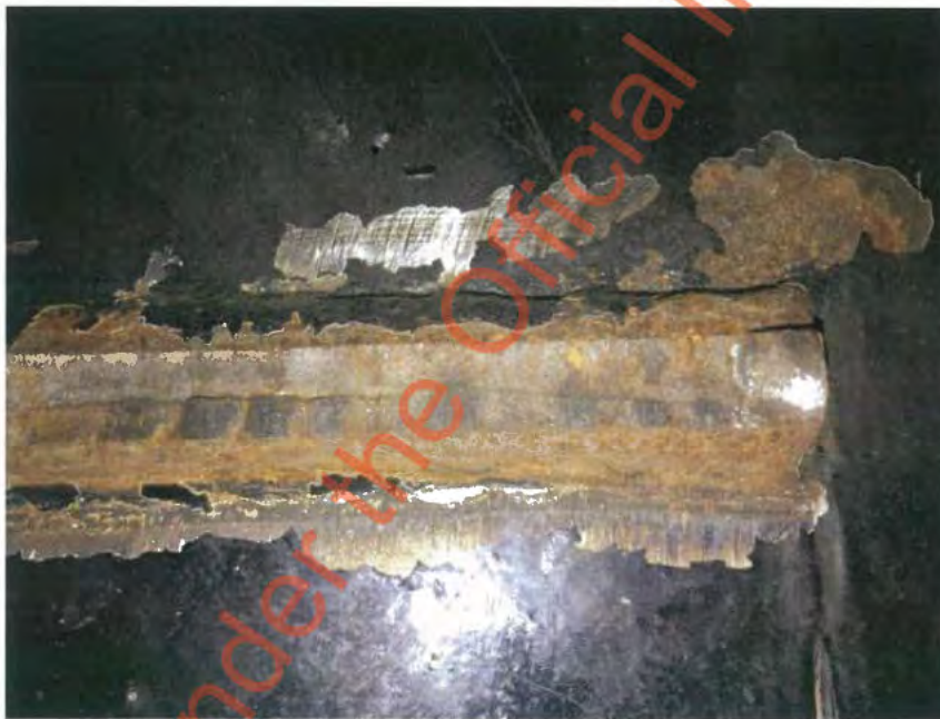
Figure 18 Plate crack propagation, stage II
