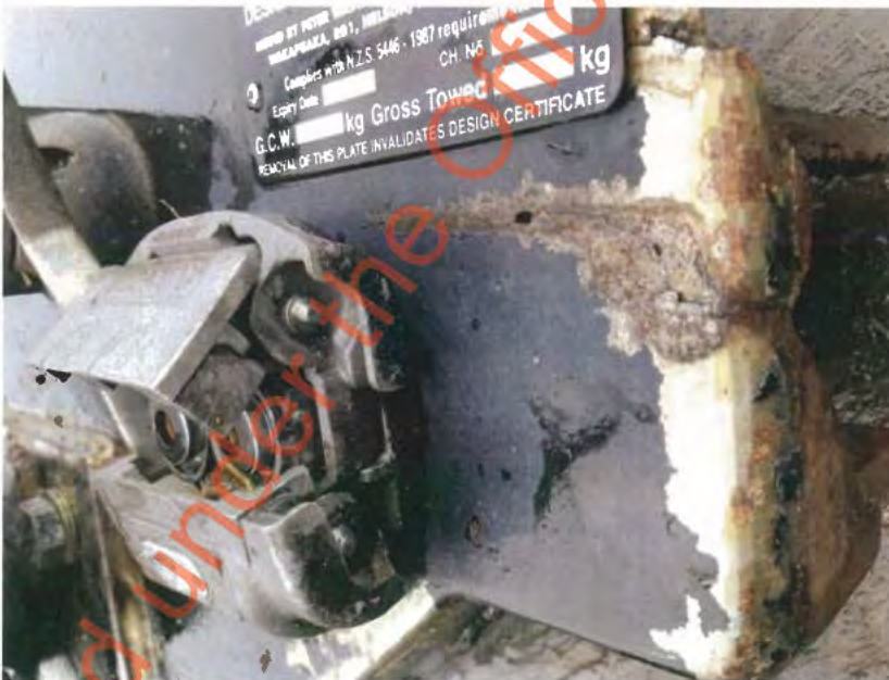
Figure 20 Plate rupture drawbeam face, stage III
