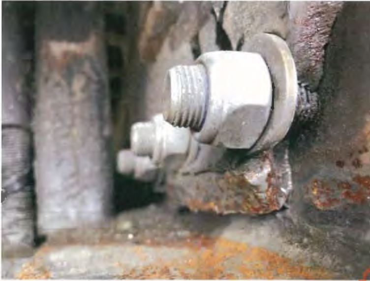
Figure 8 Bolt seating interference
