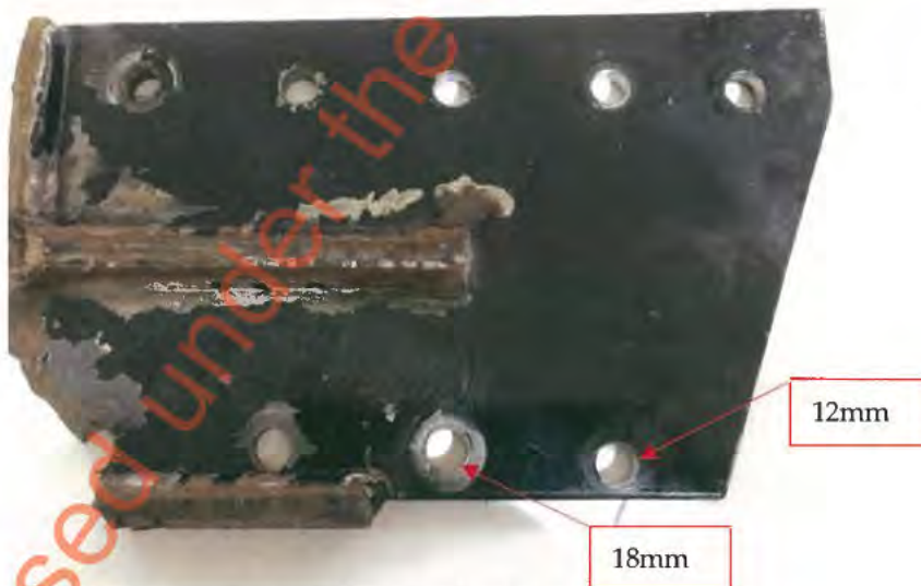
Figure 15 Bolts not meeting minimum edge distance
