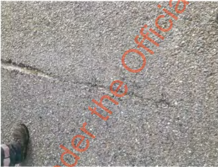
Figure 24 Groove on road surface
