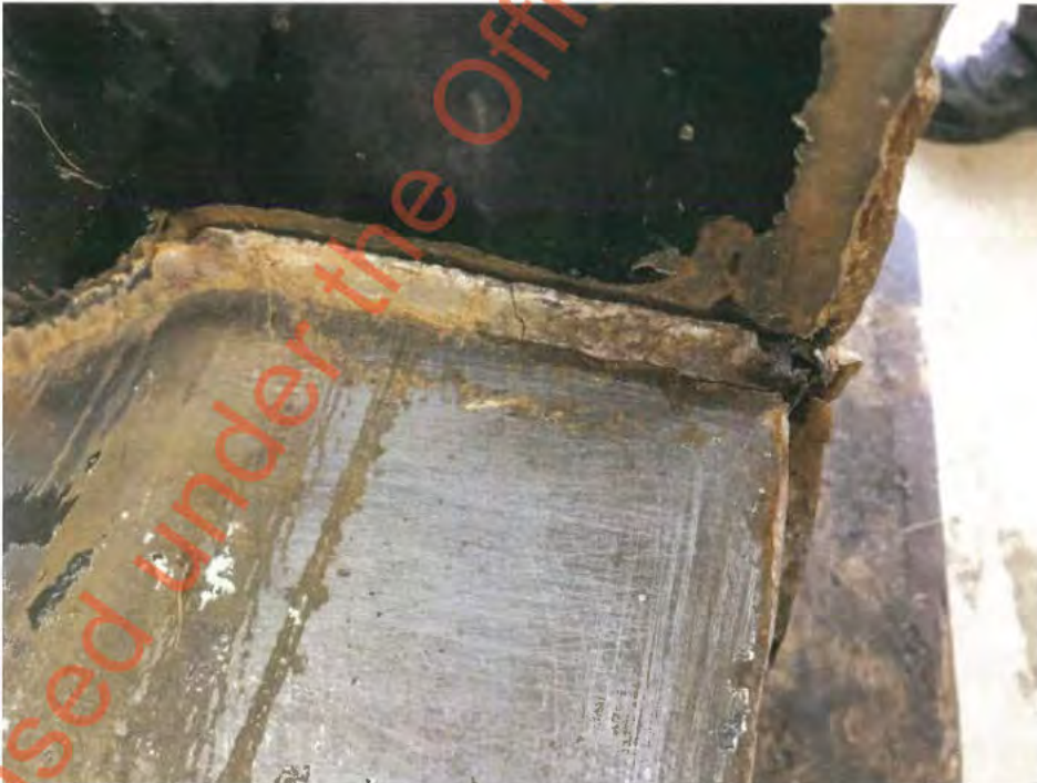
Figure 6 Cracks top stiffener to front plate
