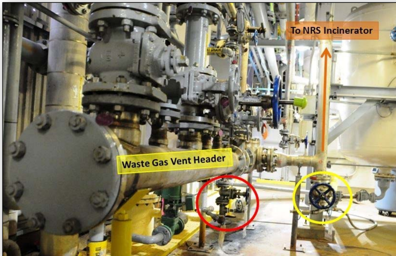
Figure 2. Waste Gas Vent Header Piping on the Third Floor of the Manufacturing Building. This portion, where several waste gas sources come together, is referred to as the waste gas vent header . Waste gas from this portion of the vent header traveled up to reach the NRS incinerator, a piping configuration that created a low spot where liquid accumulated. To remove the liquid during waste gas vent header piping high-pressure events, operators were instructed to open valves (yellow circle) and drain the system through a hose routed to a floor drain located near a safety shower. The floor drain is connected an open trench-type sump on the first floor. At the time of the incident, a second set of drain valves (red circle) were also opened directly to the floor inside the manufacturing building. Source: CSB.
