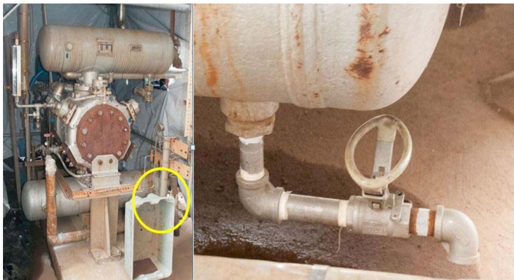
Figure 38. Methylene Chloride a Compressor. Photo shows where operators routinely drained liquid accumulation from a methylene chloride compressor without using line-breaking procedures. Source: CSB.
