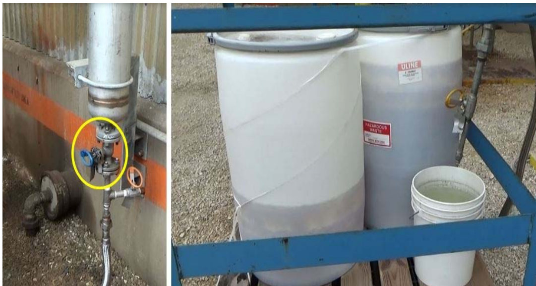
Figure 37. Photo Showing Another Line Break. Operators drained liquid accumulation in another vent header without using line-breaking procedures. Source: CSB.
