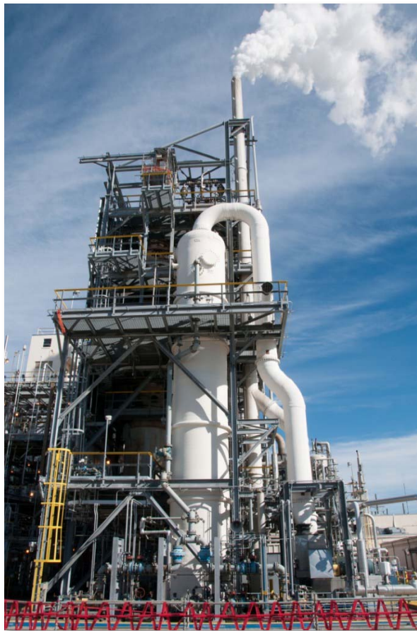
Figure 34. NRS Incinerator. NRS was installed in 2011 to reduce emissions and allow increased production at the DuPont La Porte facility. Source: CSB.
