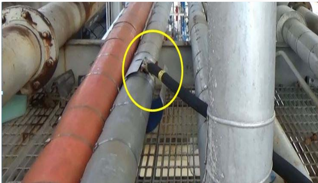
Figure 30. Hot Water Hose Positioned on the Liquid Methyl Mercaptan Feed Piping. Hot water flowed between the piping and the insulation to heat the piping and dissociate the solid hydrate that had formed after water inadvertently entered the methyl mercaptan storage tank. Source: CSB.
