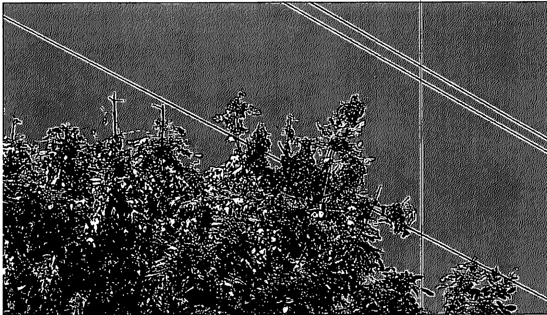
Figure 11: Tree found by Monitor team on July 12, 2019 within inches of the primary conductor and with evidence that tree leaves had been burned from contact with the primary conductor in a Tier 3 high fire-threat district.
