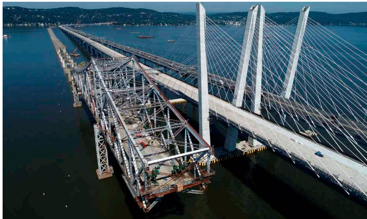
The new Governor Mario M. Cuomo Bridge alongside the former Tappan Zee Bridge ©NY State Thruway Authority
