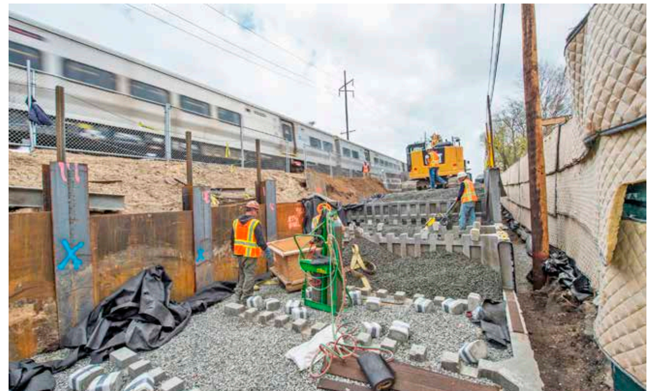
Sound and retaining walls under construction. Nearly nine miles of such walls will be built in the project area. © Metropolitan Transportation Authority
