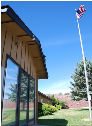
Blast-resistant film reflects the exterior landscape at a Bureau of Land Management field unit.
