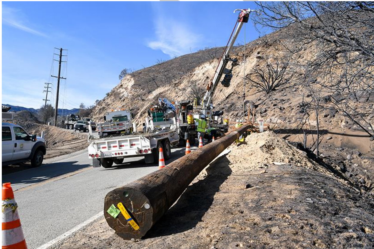
Figure 4—Infrastructure Damage – Power Pole
