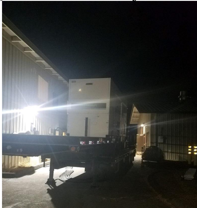
Figure 9 – Mobile Generation at a County Water District Facility
