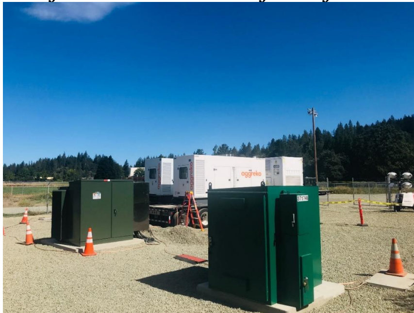
Figure 2 – Mobile Generation Staged at Angwin PIH
