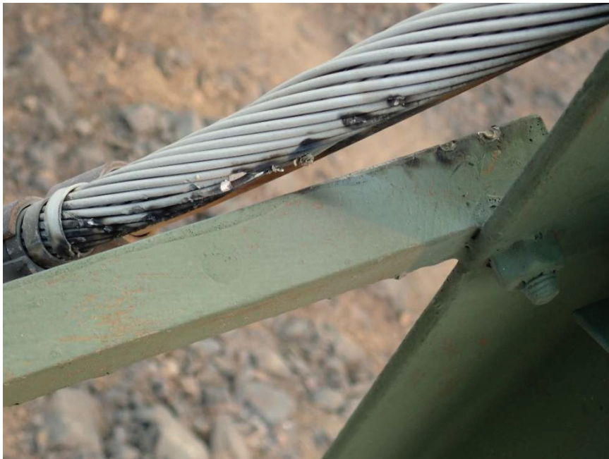
Figure 5. Flash marks on the transposition jumper and steel member on the Incident Tower. Photo provided by PG&E. 81
