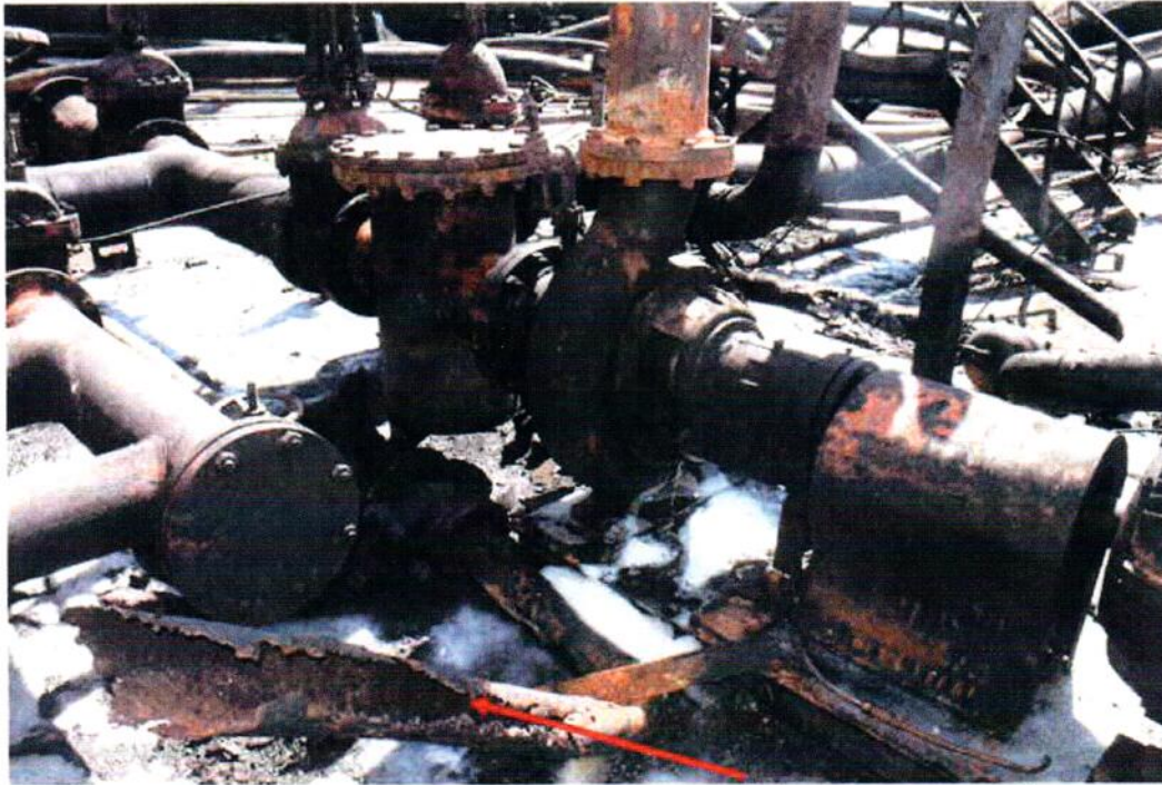
Overview of Power Frame with Damaged Pipe in Foreground
