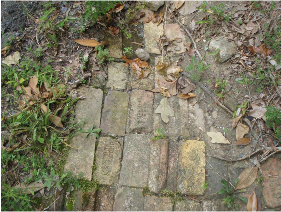
Stop 8a - Storm Drain at Falls Road and Stanly Street Made from Furnace Brick
