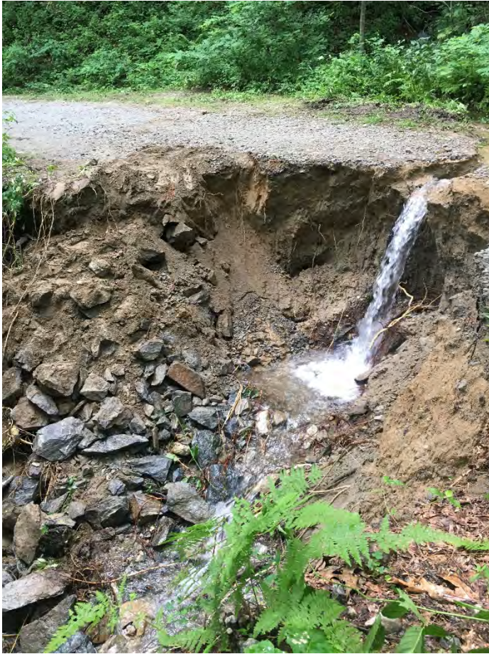
Photo 17 Damage to a Forest Road after a Culvert was Blocked with Debris during a Storm Event
