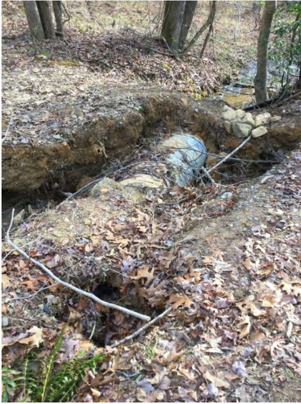
Photo 6 Failed Culverts Impact both Access and Streams
