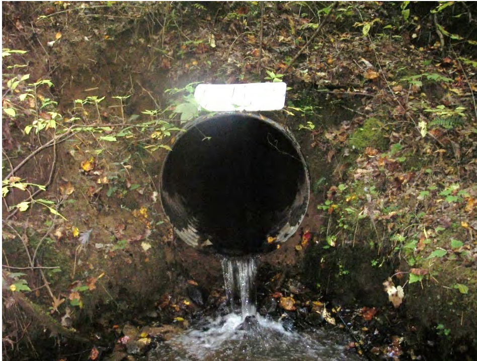
Photo 5 Example of Perched Culvert Prohibiting Fish Passage
