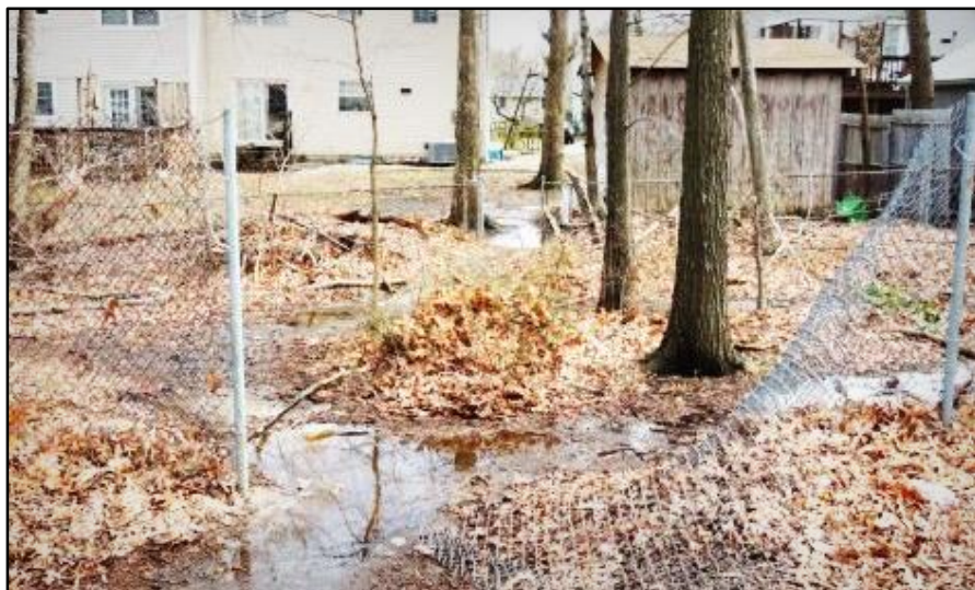
Figure 2: Inadequate perimeter fence.
