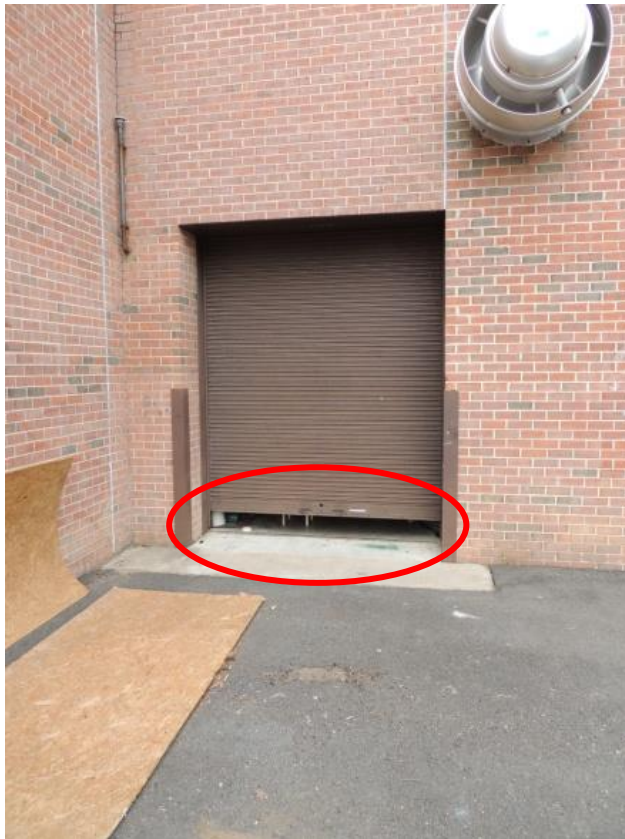
Unsecured service door
