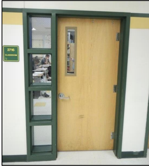
Figure 22: Example of non-ballistic resistant glass near and in door, creating vulnerability to assailants.
