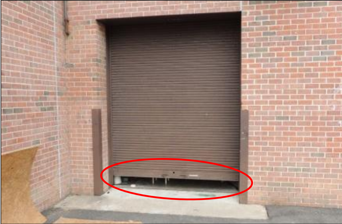
Figure 17: Partially opened service door.
