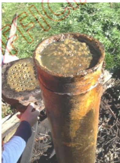
Figure 40 – Waitangi-1 casing filled with fluid and bubbles percolating (minor)
