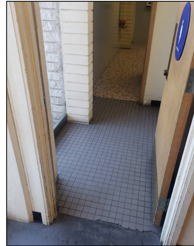
Barriers to wheelchair access at restroom entry
