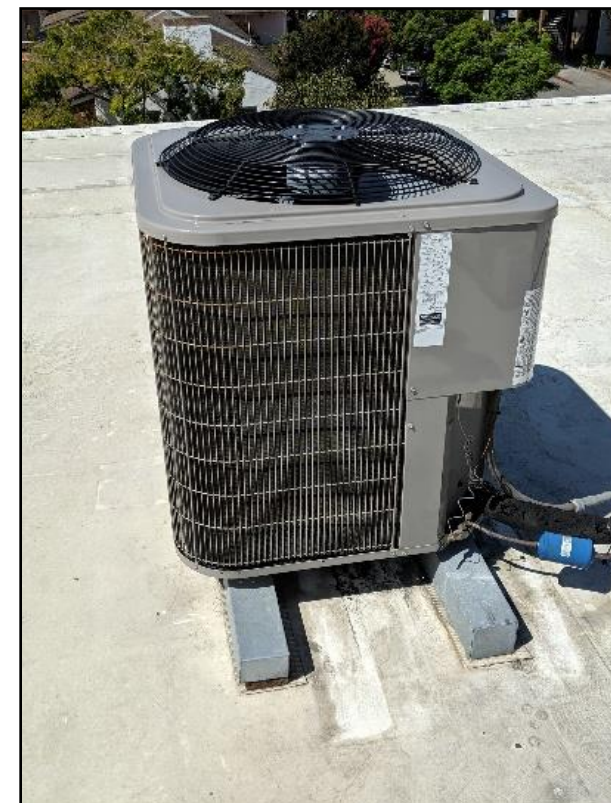
Mechanical Figure 10: Server Room Condensing Unit
