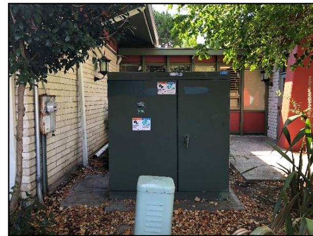
Civil Figure 10: PG&E transformer on Locust Street
