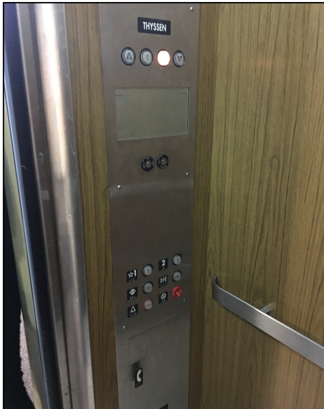
Unreliable and non-compliant elevator
