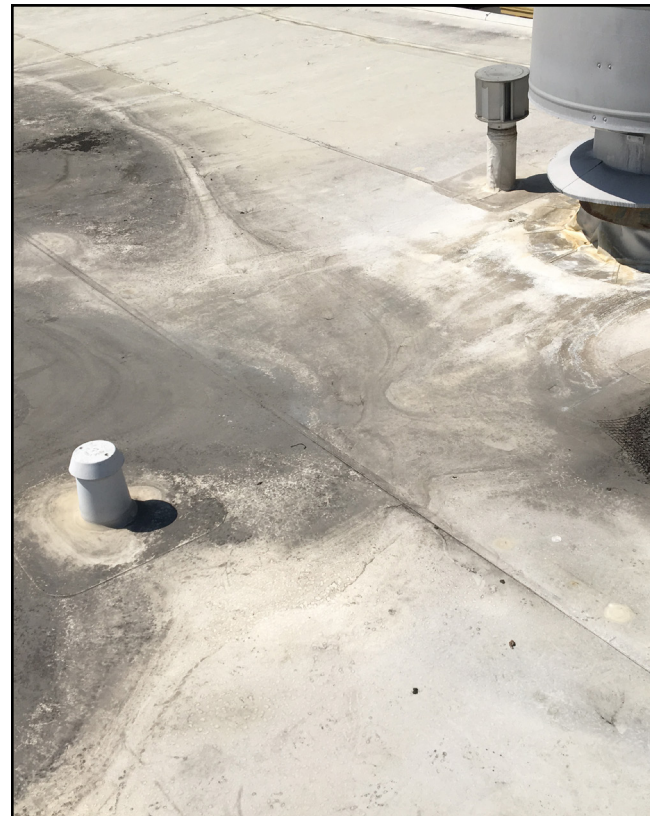
PVC roof overdue for replacement
