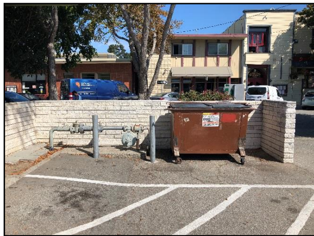
Civil Figure 9: Gas meter on Locust Street
