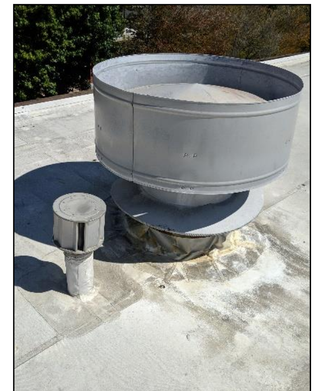
Mechanical Figure 12: Boiler Flue and Intake
