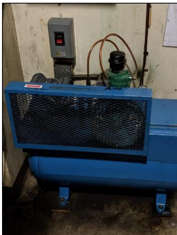
Mechanical Figure 14: Pneumatic Controls Air Compressor
