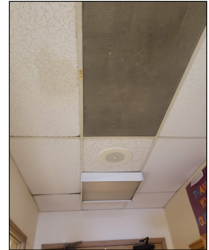
Deteriorating and water damaged ceilings
