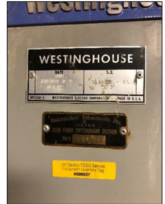
Electrical Figure 2: Electrical Gear Manufacturer
