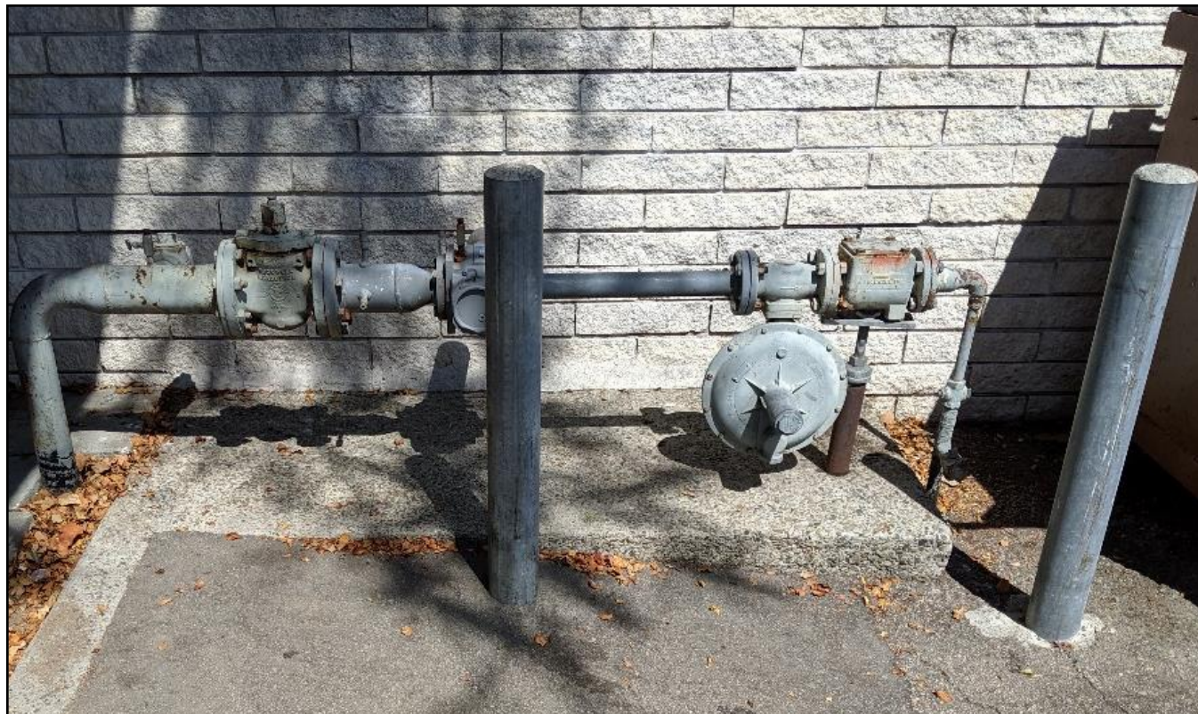
Mechanical Figure 13: Building Gas Meter
