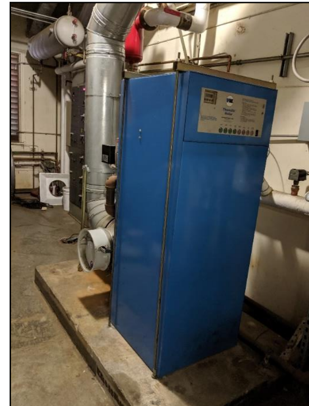
Mechanical Figure 3: Gas Fired Heating Hot Water Boiler
