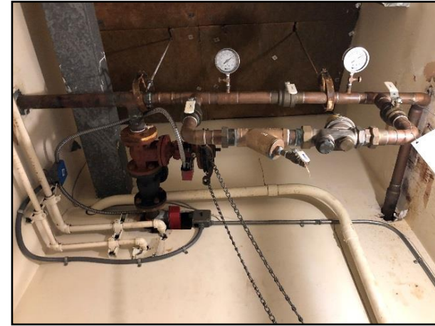
Civil Figure 8: Backflow preventer inside the building
