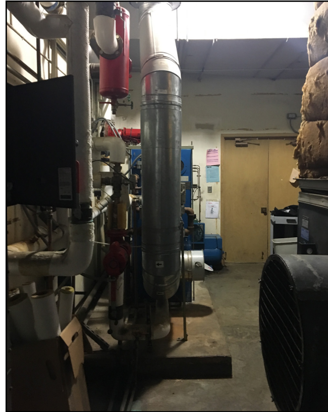
Obsolete mechanical and plumbing distribution systems
