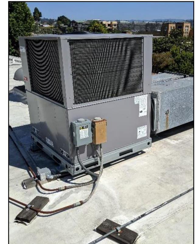
Mechanical Figure 11: Conference Room Package Unit
