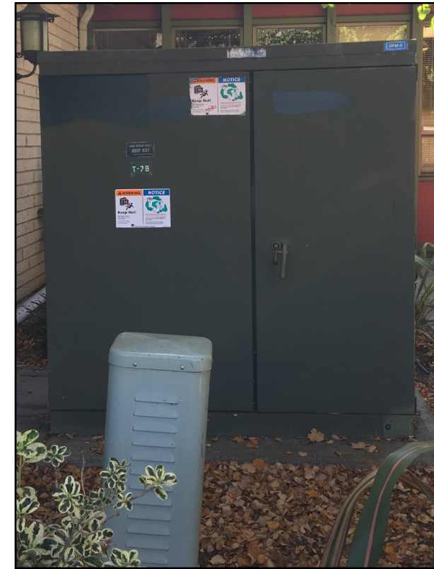
Electrical Figure 1: Utility Transformer
