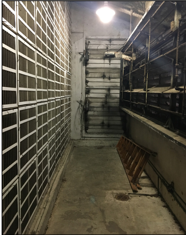
Outdated and worn air handling system
